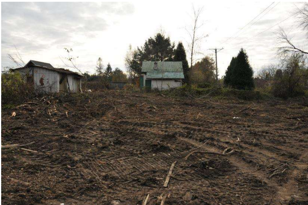
Photo. 12. Zone of demolition works of building structures in area of allotment gardens, 2nd decade of November 2020.
