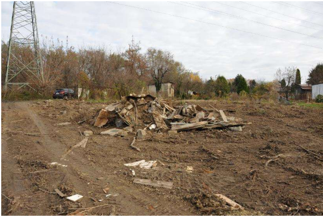
Photo. 13. Zone of demolition works of building structures in area of allotment gardens, 2nd decade of November 2020.
