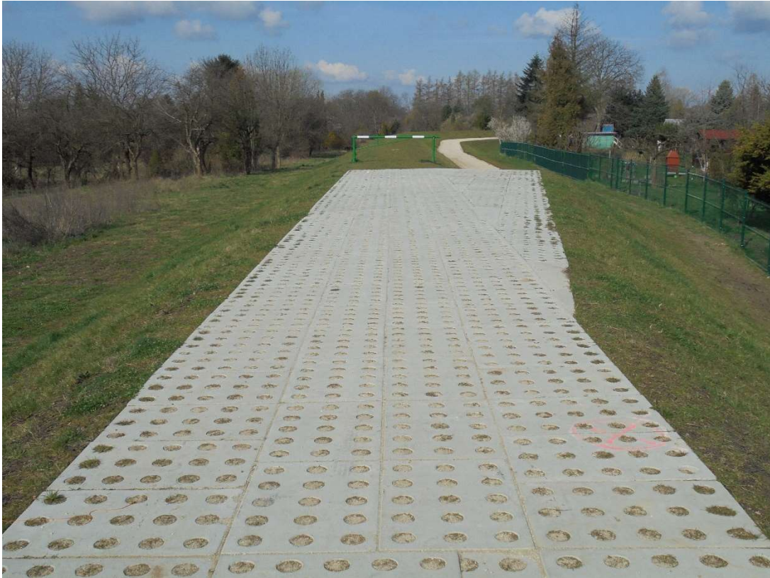
Photo. 22. New embankment of the Biała River after completion of construction. Visible fence of FAG SEMAFOR made as part of the Contract.
