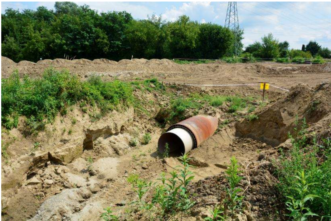
Photo. 17. Zone of works and excavation for storm sewer, 3rd decade of July 2021.
