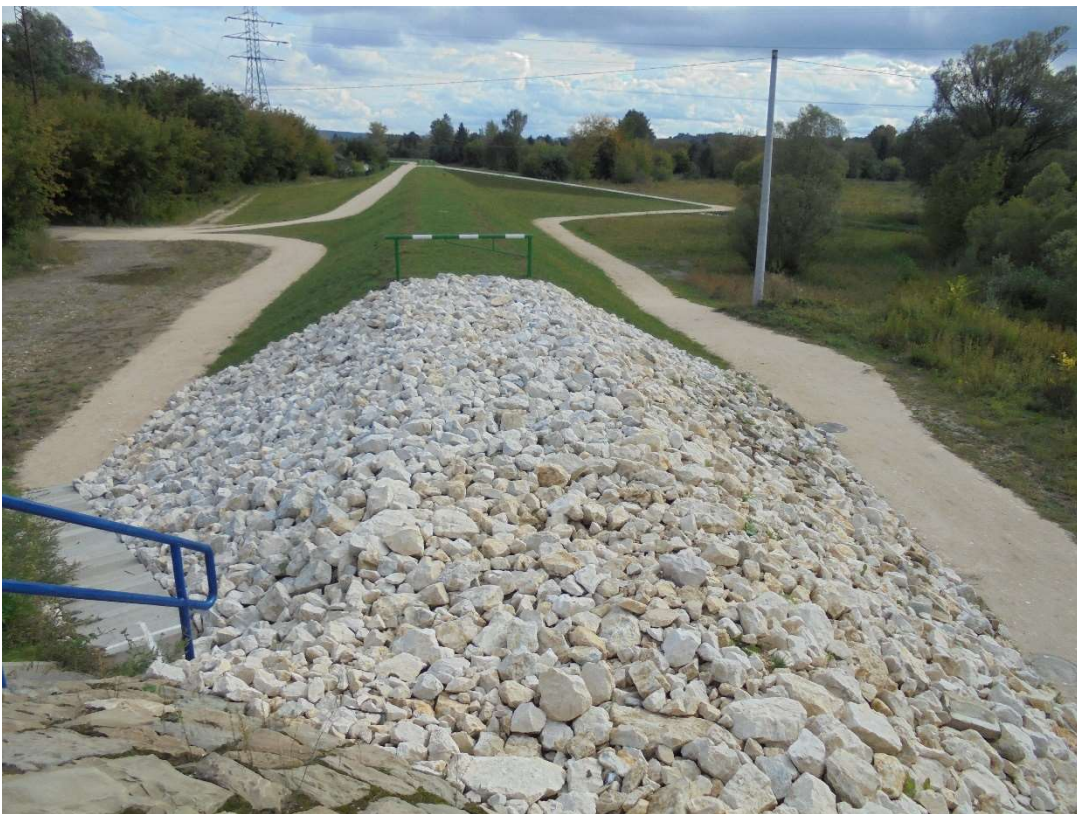
Photo. 21. New embankment of the Biała River after completion of construction. Connection to the railway embankment.
