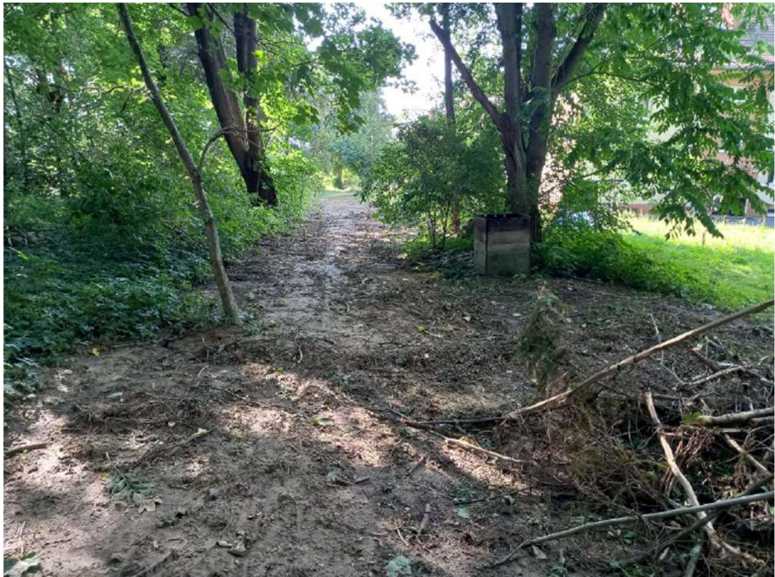
Photo. 16. Construction site of the teletechnical network along the distance of the sluice channel of the Przewóz barrage, status in the third decade of July 2022 (view towards the west).
