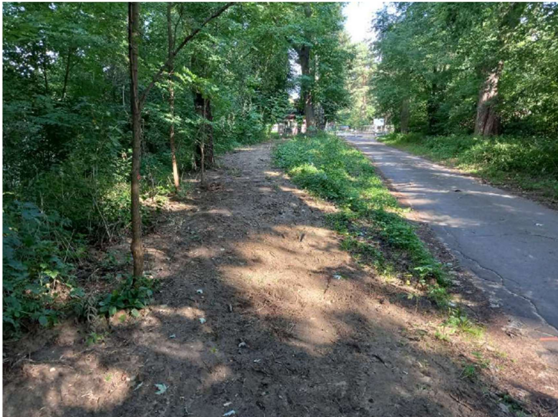
Photo. 17. Construction site of the teletechnical network at the distance along the sluice channel of the Przewóz barrage, status in the third decade of July 2022 (view towards the east).
