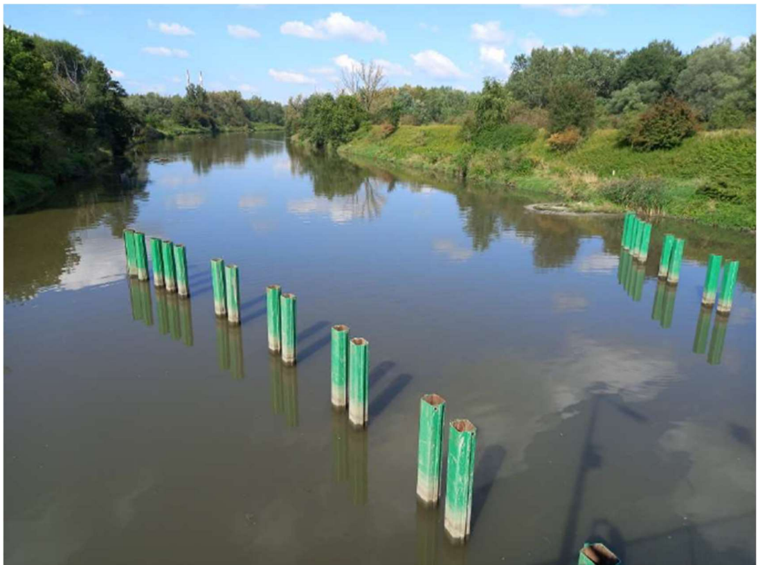
Photo. 30. Construction site of the flood gate on the Kujawy port channel – northern part, status in the third decade of August 2023 (view towards the north).
