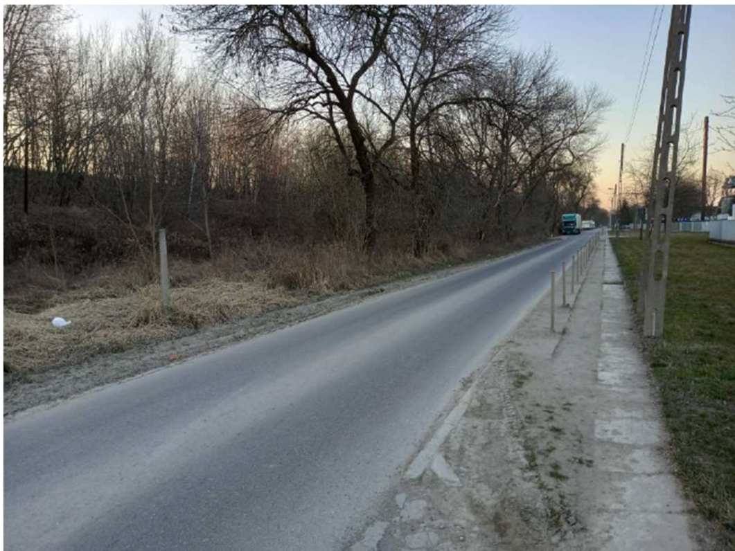
Photo. 8. Condition of the site before the start of construction - construction of the power network along Dymarek Street, status in the third decade of March 2022 (view towards the north).
