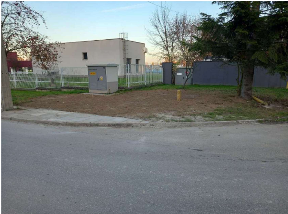
Photo. 21. Construction site of the power network at the distance along Dymarek Street, status in the third decade of October 2022 (view towards north-east).
