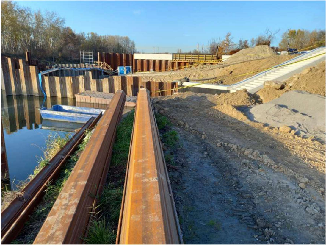
Photo. 19. Embanked area on the east bank of the Kujawy port channel at the height of the construction site of the flood gate, status in the third decade of October 2022 (view upstream the channel).
