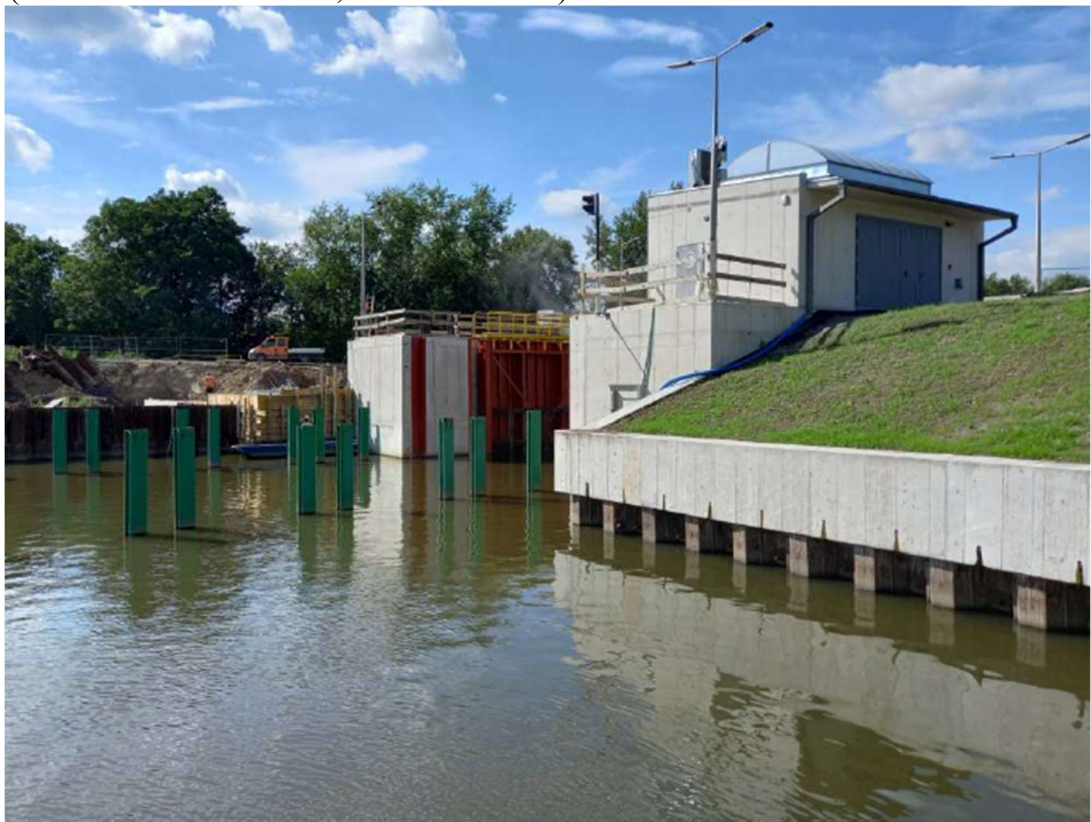
Photo. 26. Construction site of the flood gate on the Kujawy port channel – south part, status in the third decade of July 2023 (view from the east bank, towards the west).
