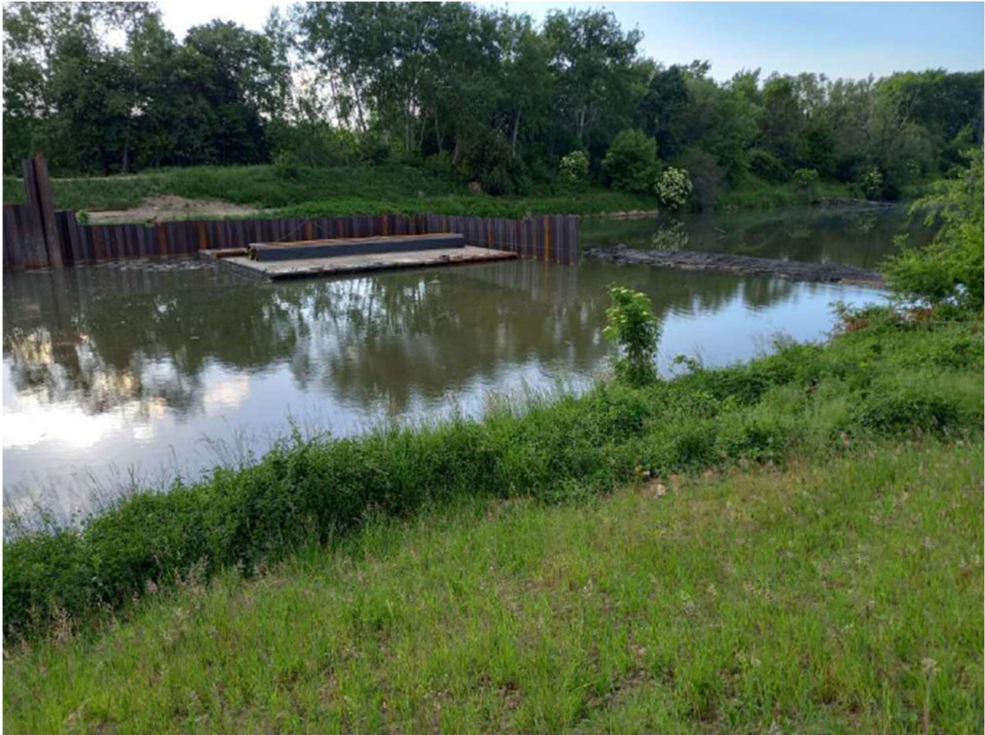
Photo. 13. Construction site of the flood gate on the Kujawy port channel, status in the third decade of May 2022 (view from the east bank, upstream the channel).
