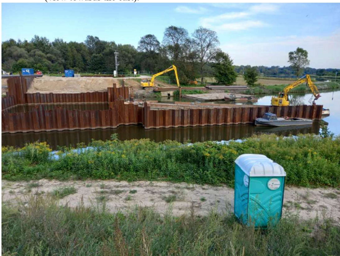
Photo. 18. Construction site of the flood gate on the Kujawy port channel, status in the third decade of August 2022 (view from the west bank, downstream the channel).
