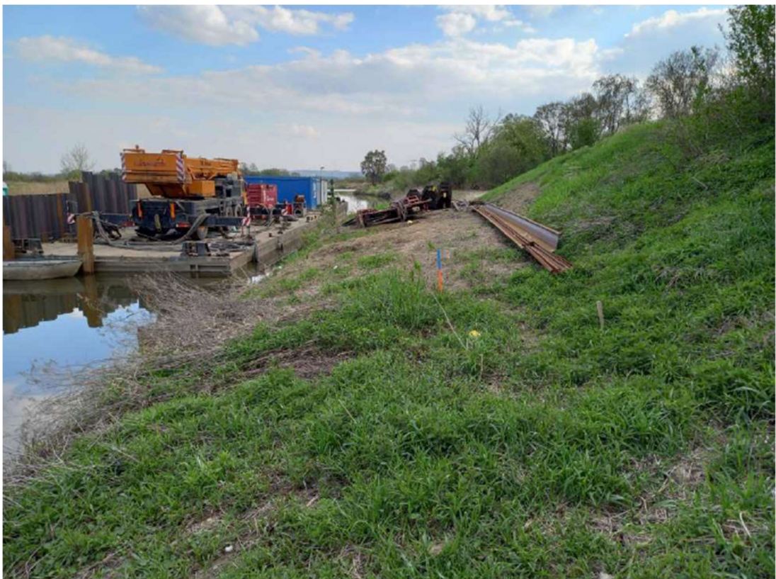
Photo. 12. Embanked area on the west bank of the Kujawy port channel at the height of the construction site of the flood gate, status in the third decade of April 2022 (view downstream the channel).
