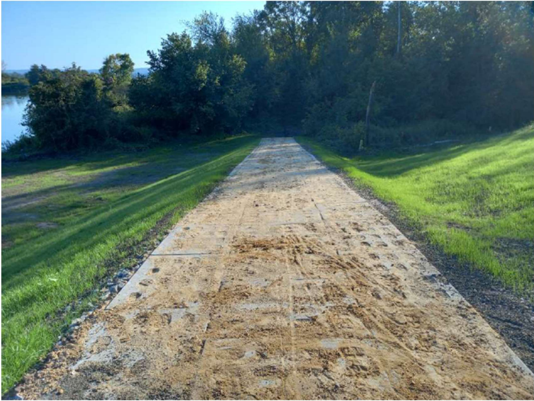
Photo. 33. Reconstructed south descent way from the flood embankment on the west bank of the channel of Kujawy port, status in the third decade of September 2023 (view towards the south).
