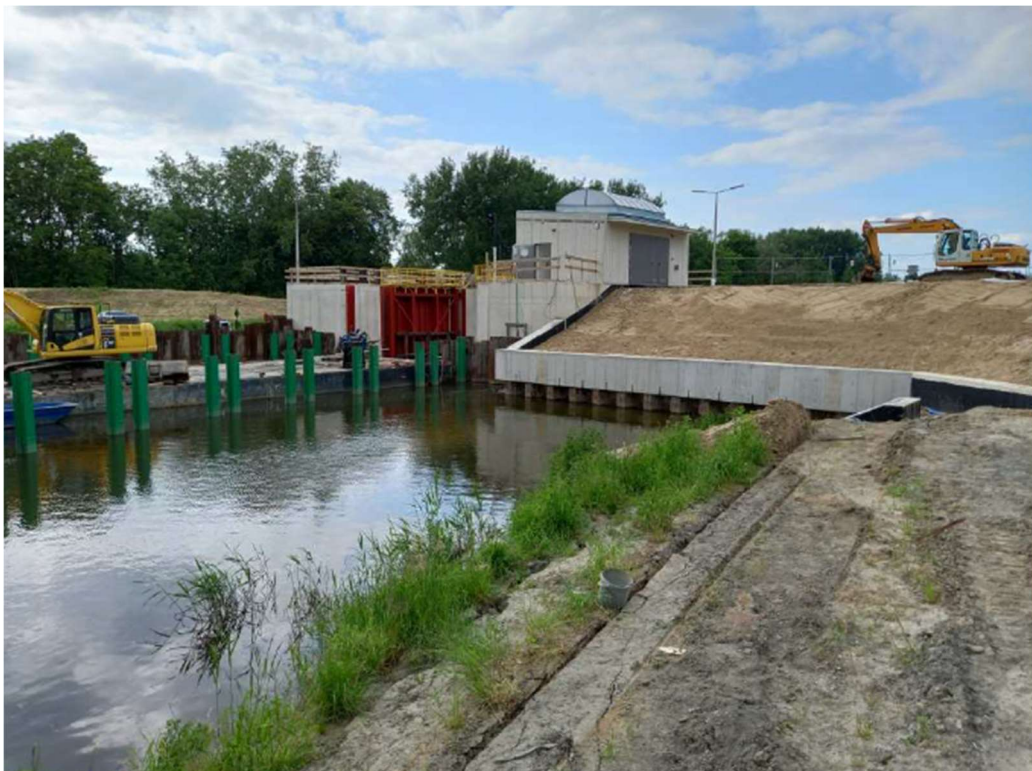
Photo. 24. Construction site of the flood gate on the Kujawy port channel – south and central part, status in the third decade of May 2023 (view from the east bank, towards the north-west).
