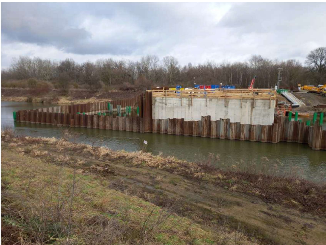
Photo. 22. Construction site of the flood gate on the Kujawy port channel, – northern and central part, status in the third decade of January 2023 (view from the west bank, upstream the channel).
