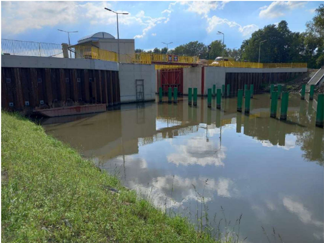
Photo. 29. Construction site of the flood gate on the Kujawy port channel – northern part, status in the third decade of August 2023 (view from the east bank, towards the south-west).
