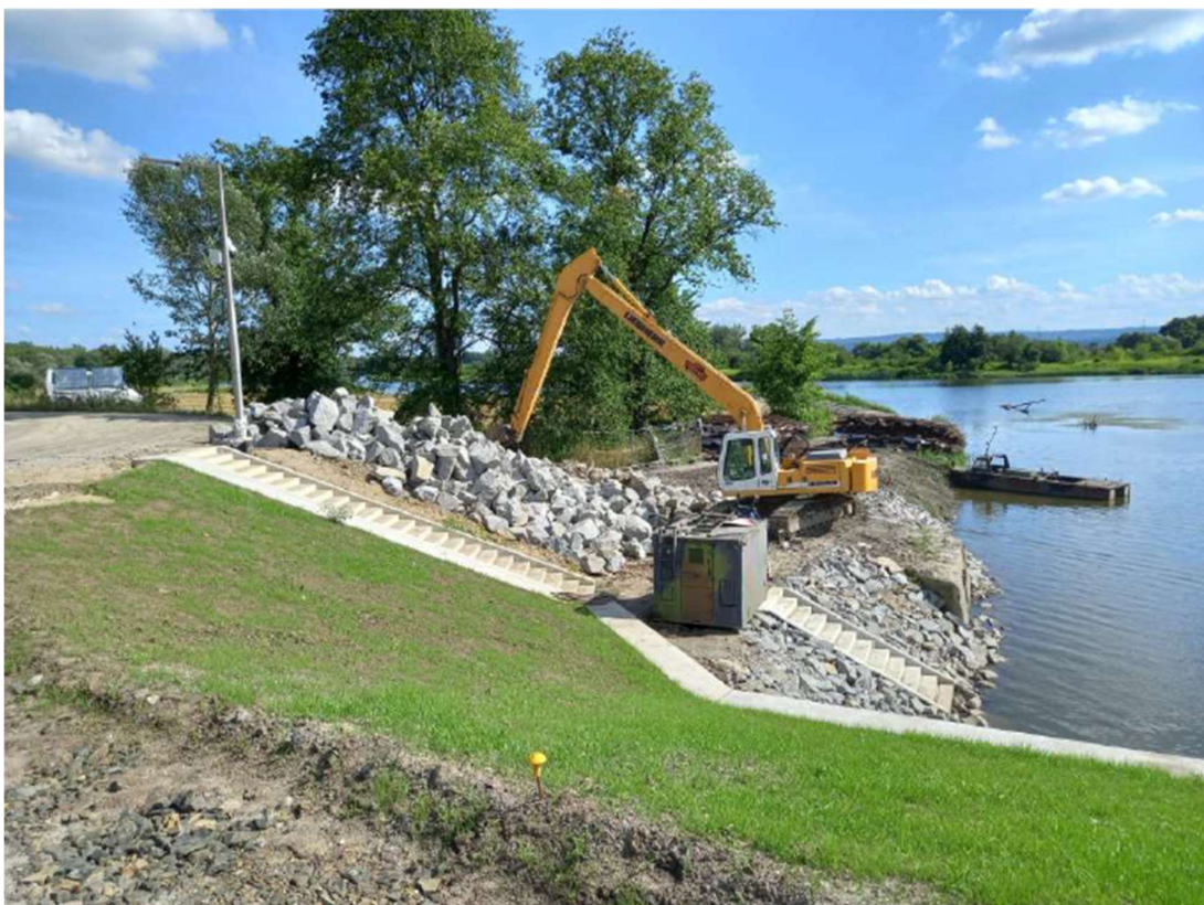
Photo. 28. Construction site on the eastern embanked area of the Kujawy port channel, – south part, status in the third decade of July 2023 (view towards the south).
