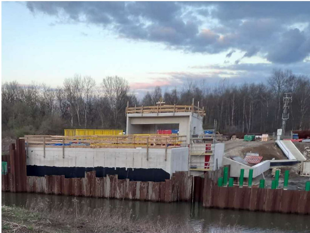
Photo. 23. Construction site of the flood gate on the Kujawy port channel – central part, status in the third decade of March 2023 (view from the west bank, towards the east).
