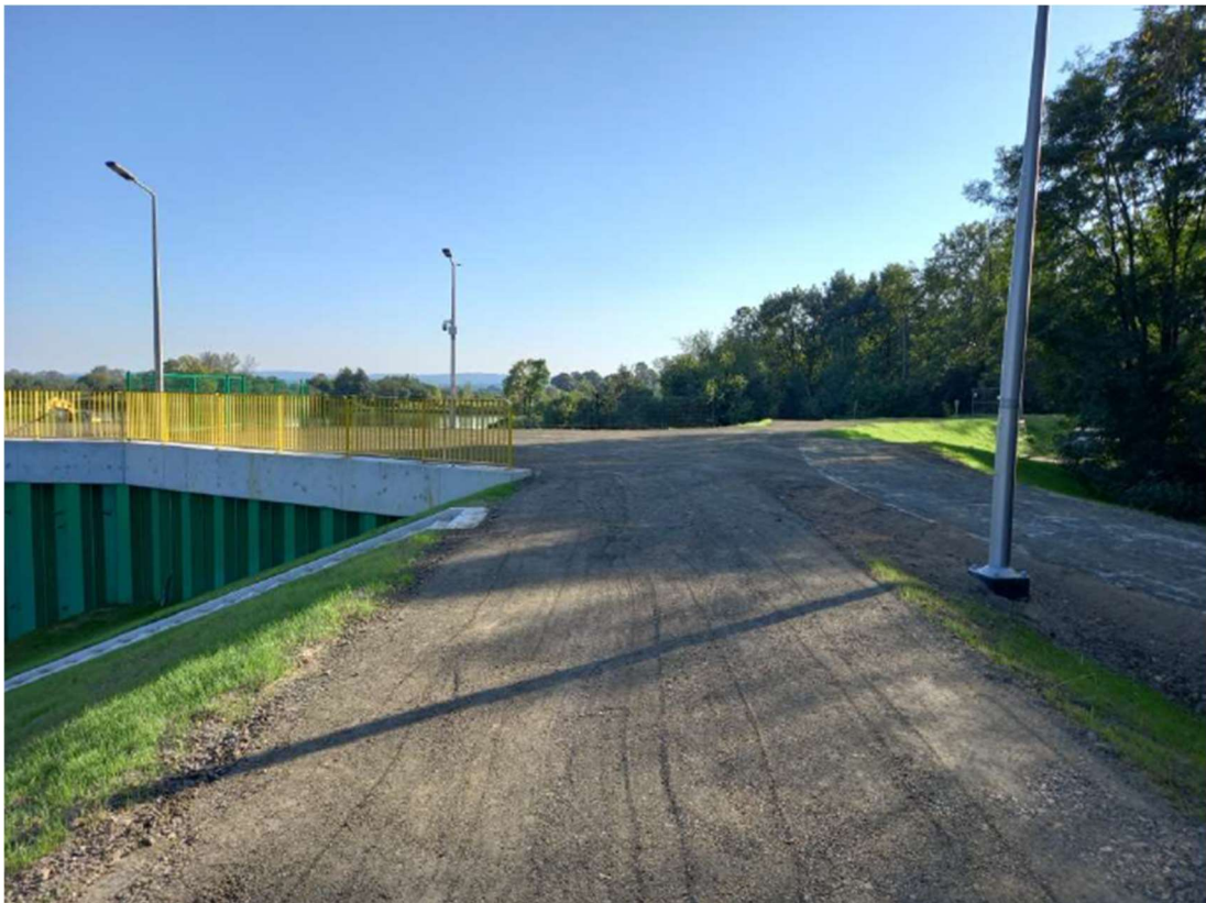
Photo. 32. Reconstructed flood embankment on the west bank of the Kujawy port channel, status in the third decade of September 2023 (view towards the south).
