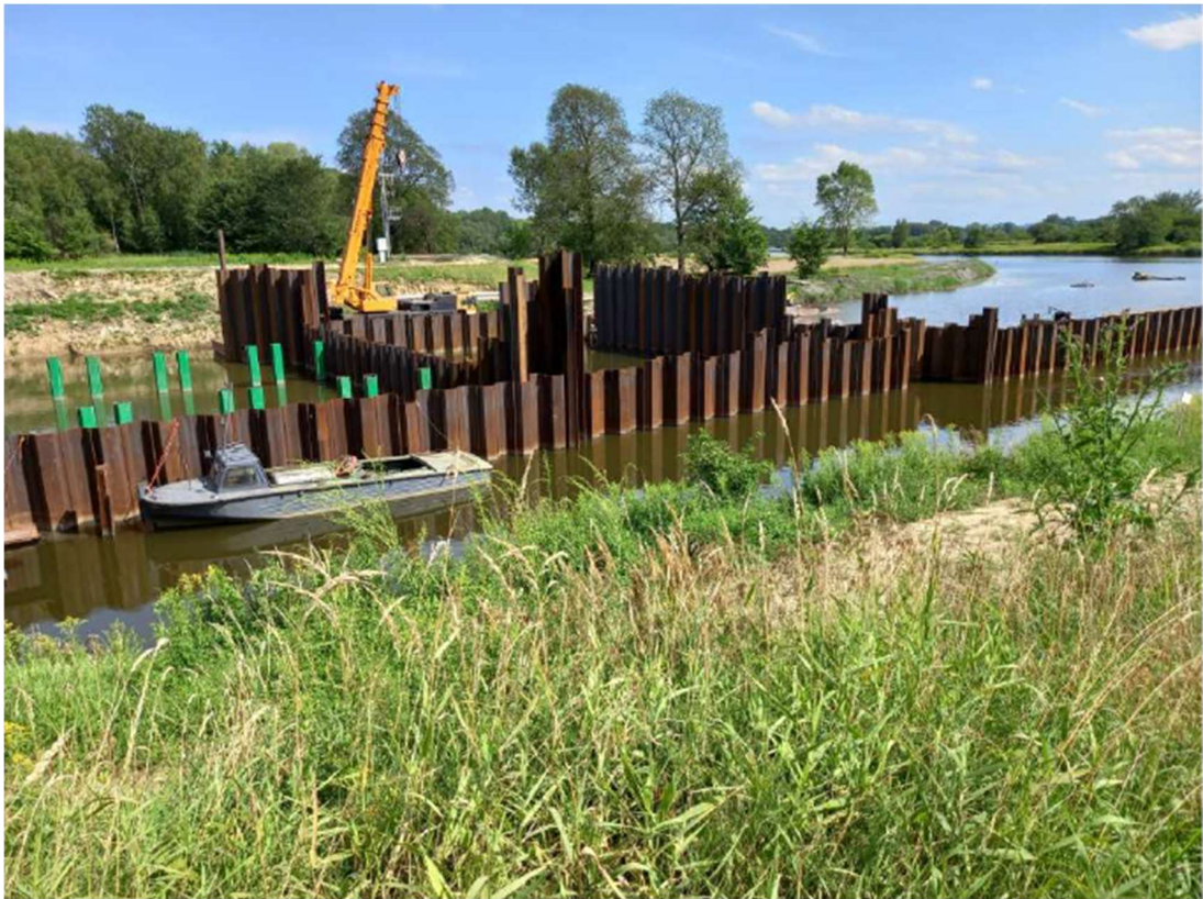
Photo. 15. Construction site of the flood gate on the Kujawy port channel, status in the third decade of July 2022 (view from the west bank, downstream the channel).
