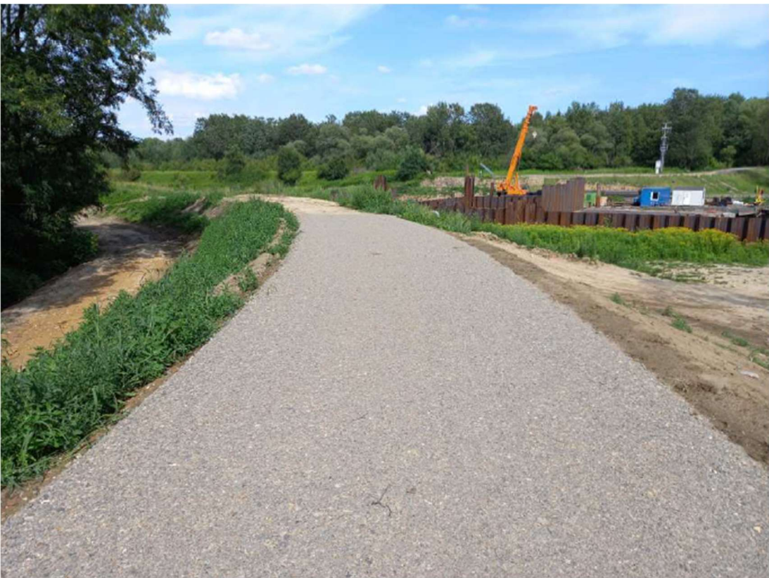
Photo. 14. Reconstructed flood embankment on the west bank of the Kujawy port channel, status in the third decade of July 2022 (view upstream the channel).
