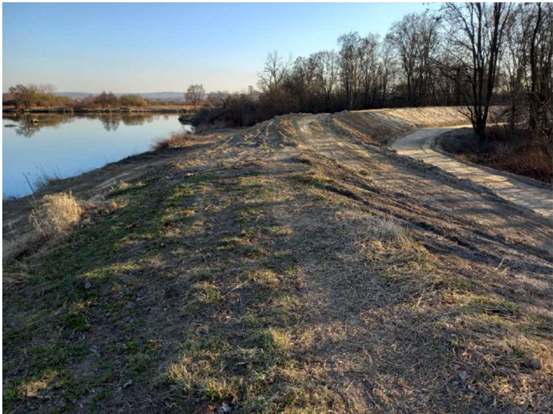
Photo. 4. Condition of the site before the start of construction – flood embankment on the right bank of the channel of Kujawy port.
