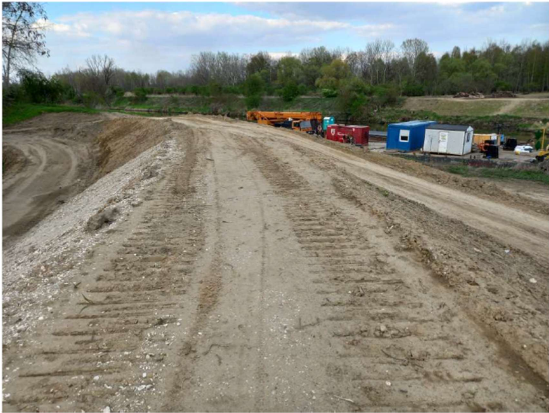
Photo. 11. Reconstructed flood embankment on the west bank of the Kujawy port channel, status in the third decade of April 2022 (view upstream the channel).
