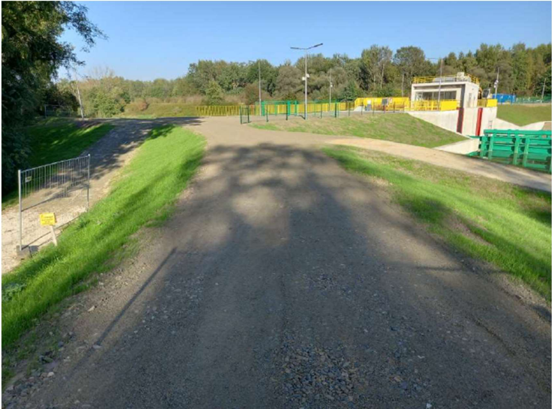
Photo. 31. Reconstructed flood embankment on the west bank of the Kujawy port channel, status in the third decade of September 2023 (view towards the north).
