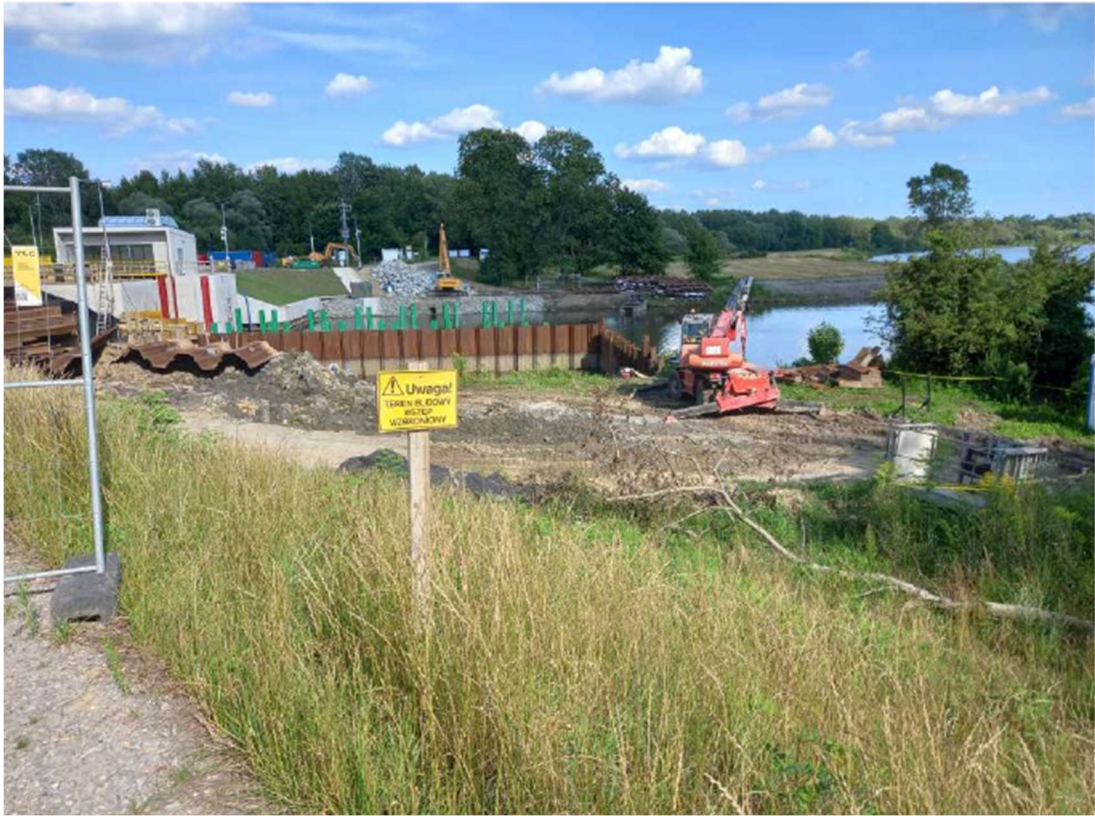
Photo. 25. Construction site of the flood gate on the Kujawy port channel, – south part, status in the third decade of July 2023 (view from the west bank, towards the east).
