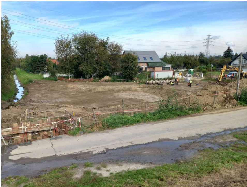
Photo. 30. Forming of slopes of the storage reservoir at Ditch 2a, status in the third decade of September 2022 (view towards the north).
