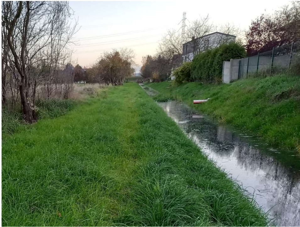
Photo. 37. Growth of grass on bank slopes at Ditch 2a after finishing the works at this section, (view towards the south).
