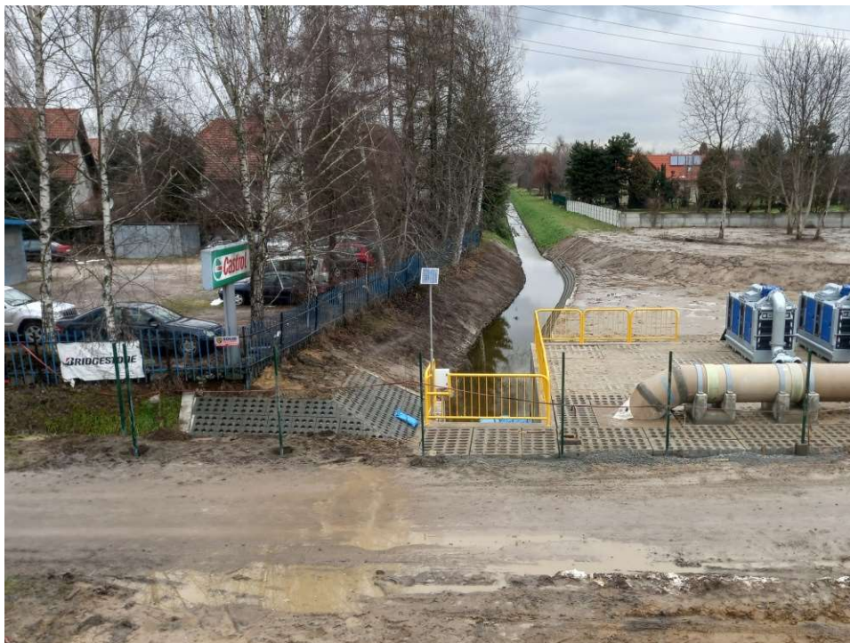
Photo. 44. Condition of the construction site in the last month of the execution of works – construction site of the embankment sluice at Ditch 2a from the side of the area beyond the embankment of the Vistula, status in the third decade of January 2023 (view towards the north).
