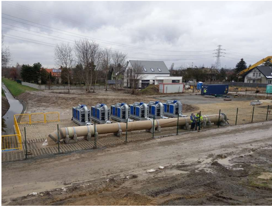
Photo. 45. Condition of the construction site in the last month of the execution of works – construction site of the pumping station for mobile pumps and the storage reservoir upstream of the embankment sluice, status in the third decade of January 2023 (view towards the north).
