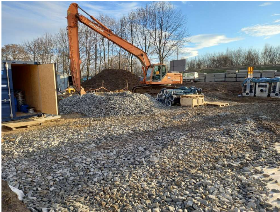
Photo. 33. Construction of manoeuvring yard at the station of mobile pumps at Ditch 2a, status in the third decade of December 2022 (view towards the south-east).
