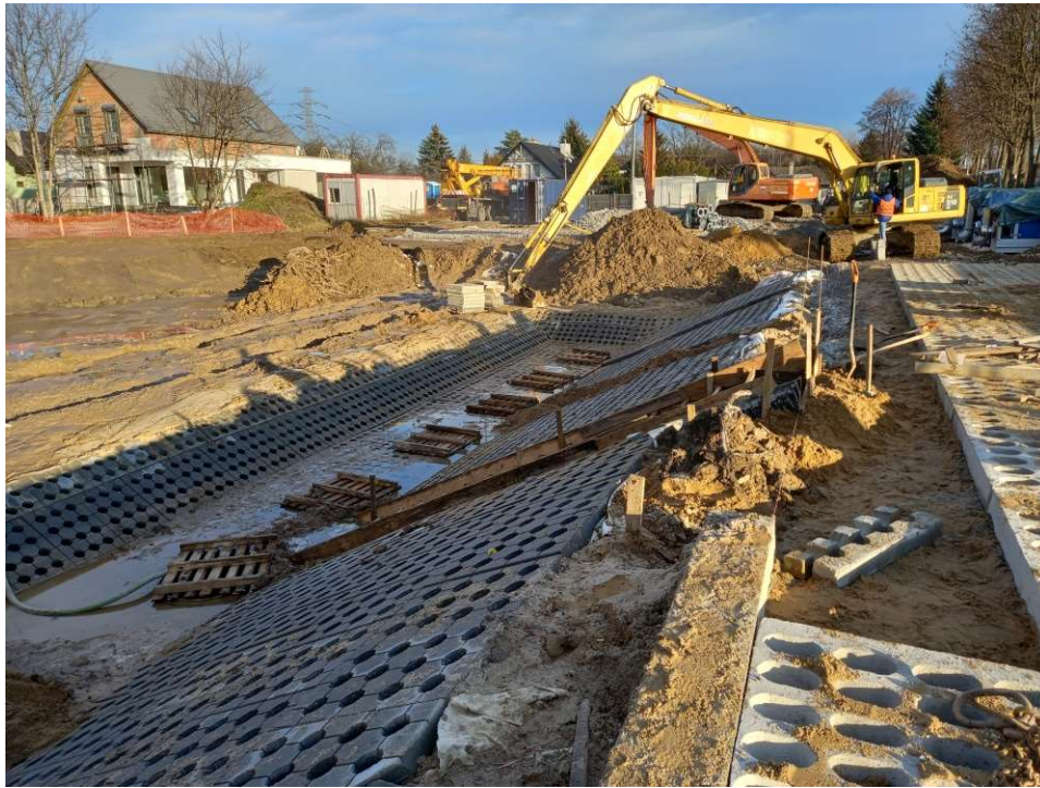
Photo. 31. Construction of a station for mobile pumps at Ditch 2a, status in the third decade of December 2022 (view towards the east).
