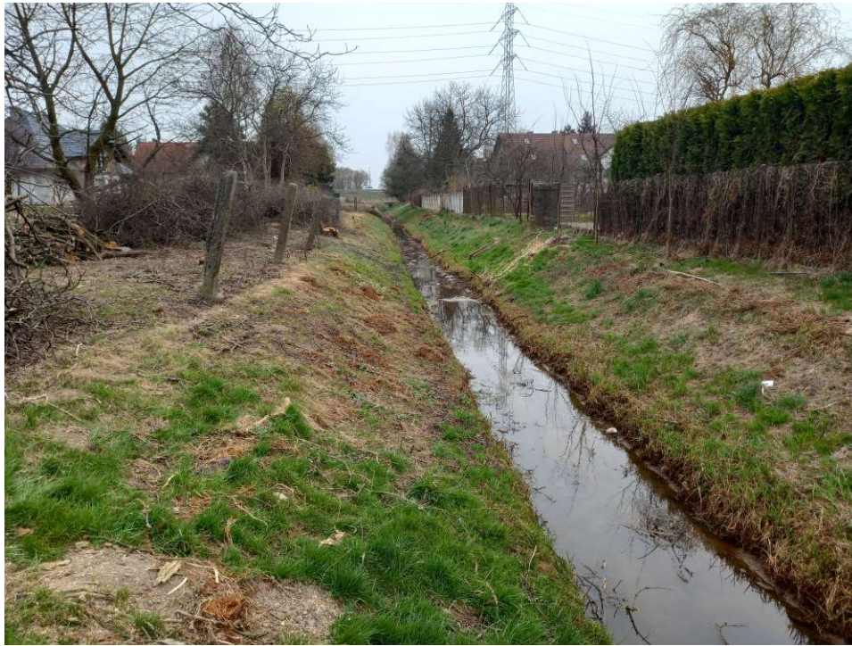
Photo. 13. Condition of the construction site in the first month of the execution of works – the reconstructed section of Ditch 2a – the lower part, status in the third decade of March 2022 (view towards the south).
