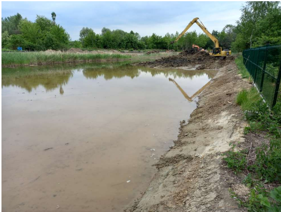
Photo. 40. Earthworks on the south bank of the enlarged reservoir at Ditch 2, status in the third decade of May 2022 (view towards the east).
