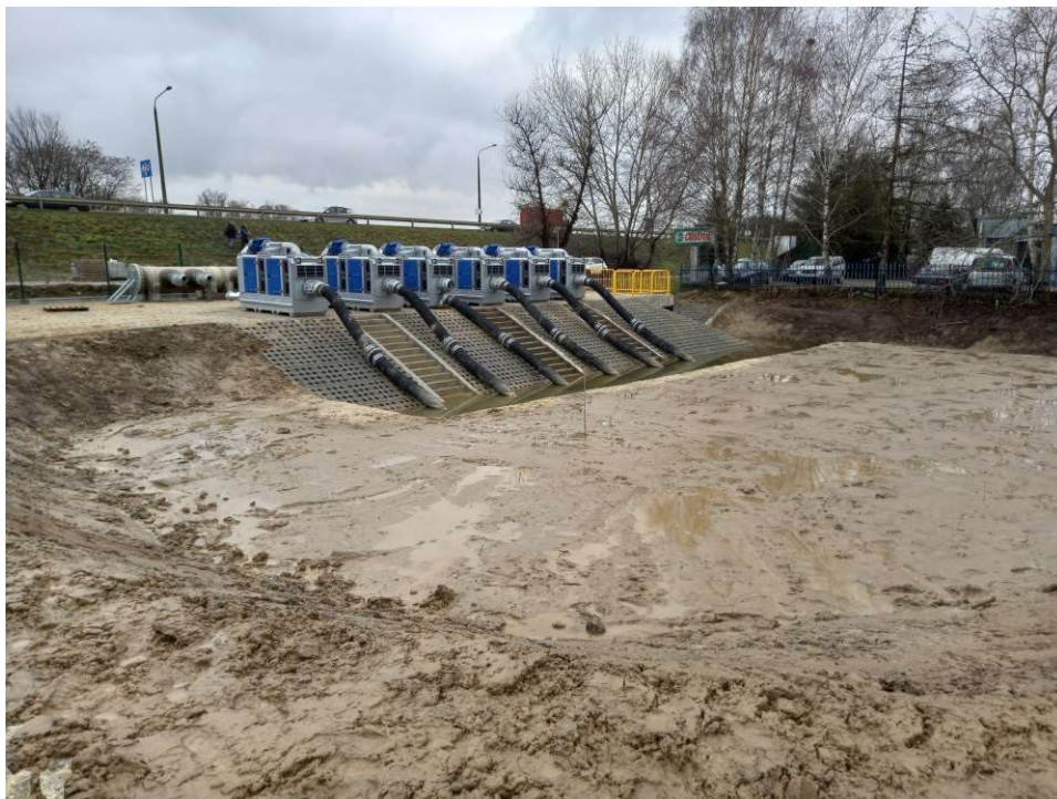
Photo. 46. Condition of the construction site in the last month of the execution of works – construction site of the storage reservoir upstream of the embankment sluice and of the pumping station for mobile pumps, status in the third decade of January 2023 (view towards the south).
