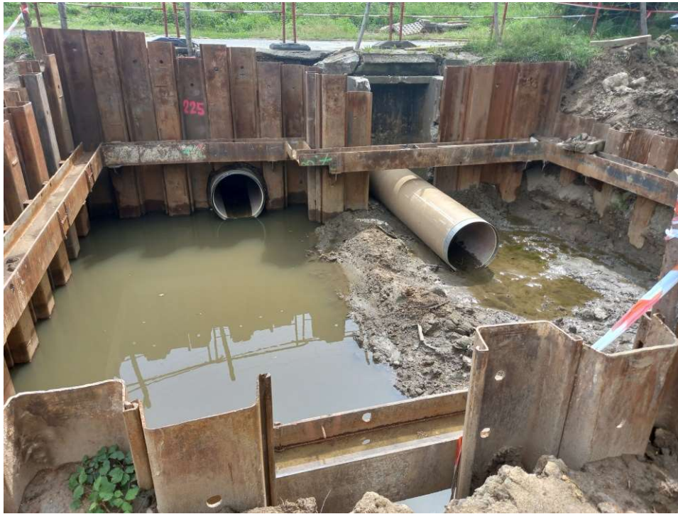
Photo. 27. Reconstructed gravity pipeline (on the right) and new pressure pipeline (on the left) at the embankment sluice construction site at Ditch 2a, status in the third decade of July 2022 (view towards the south).
