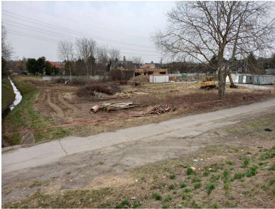
Photo. 11. Condition of the construction site in the first month of the execution of works – construction site of the pumping station for mobile pumps and the storage reservoir upstream of the embankment sluice, status in the third decade of March 2022 (view towards the north).
