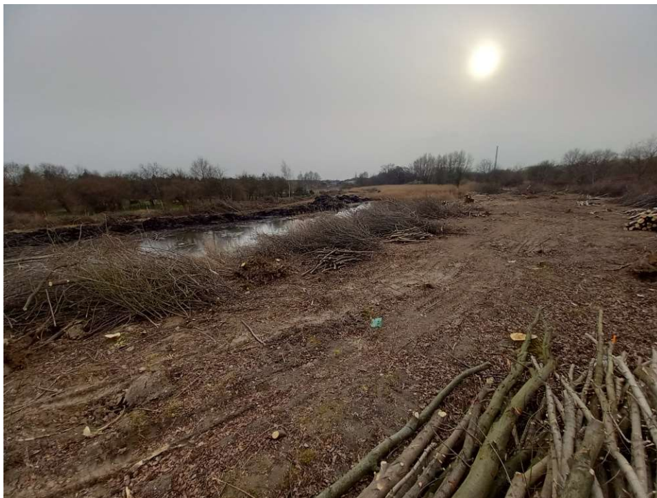
Photo. 18. Condition of the construction site in the first month of the execution of works – the reconstructed reservoir at Ditch 2, western part, status in the third decade of March 2022 (view towards the west).
