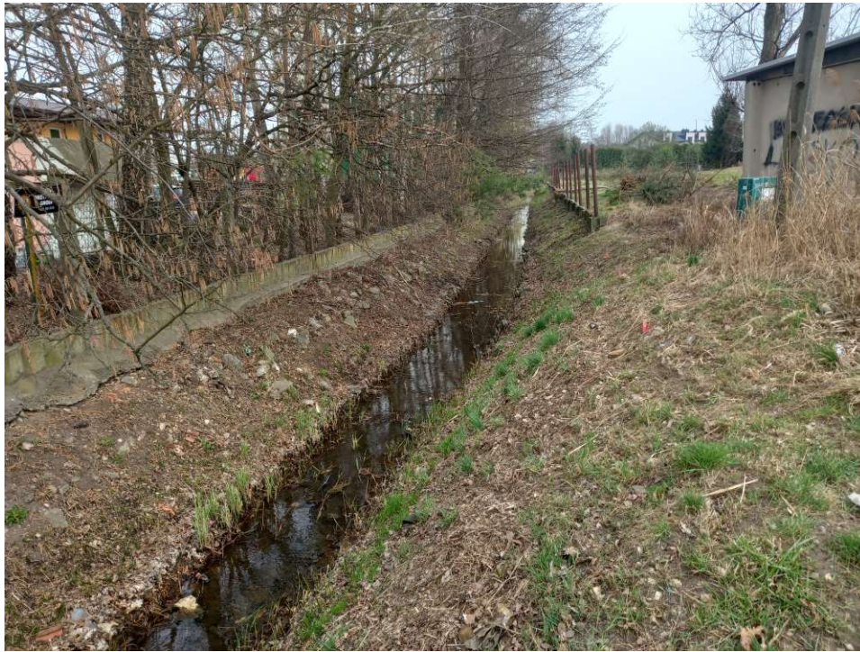
Photo. 15. Condition of the construction site in the first month of the execution of works – the reconstructed section of Ditch 2 – the lower part, status in the third decade of March 2022 (view towards the east).
