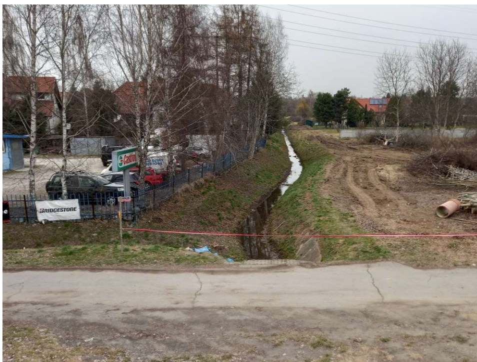
Photo. 10. Condition of the construction site in the first month of the execution of works – construction site of the embankment sluice at Ditch 2a from the side of the area beyond the embankment of the Vistula, status in the third decade of March 2022 (view towards the north).
