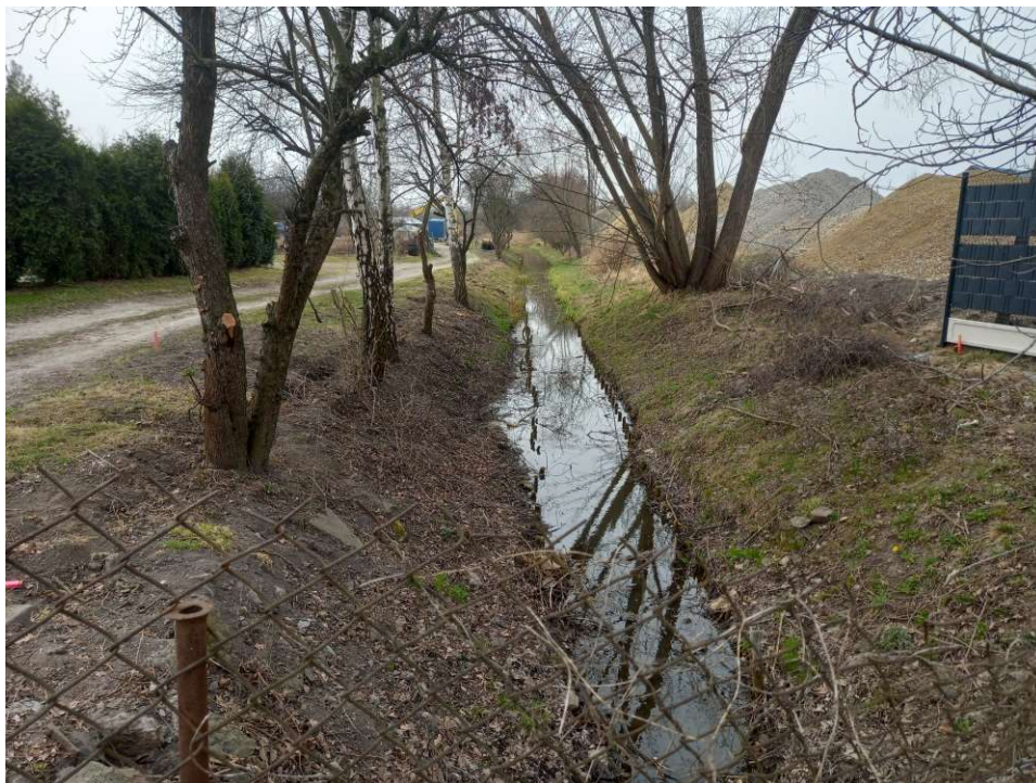
Photo. 16. Condition of the construction site in the first month of the execution of works – the reconstructed section of Ditch 2 – the upper part, status in the third decade of March 2022 (view towards the west).
