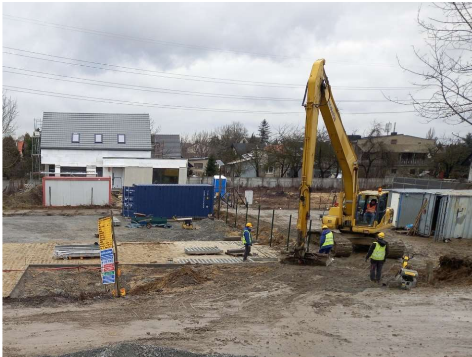
Photo. 34. Land reclamation in the surrounding of the manoeuvring yard and the station of mobile pumps at Ditch 2a, status in the third decade of January 2023 (view towards the north).
