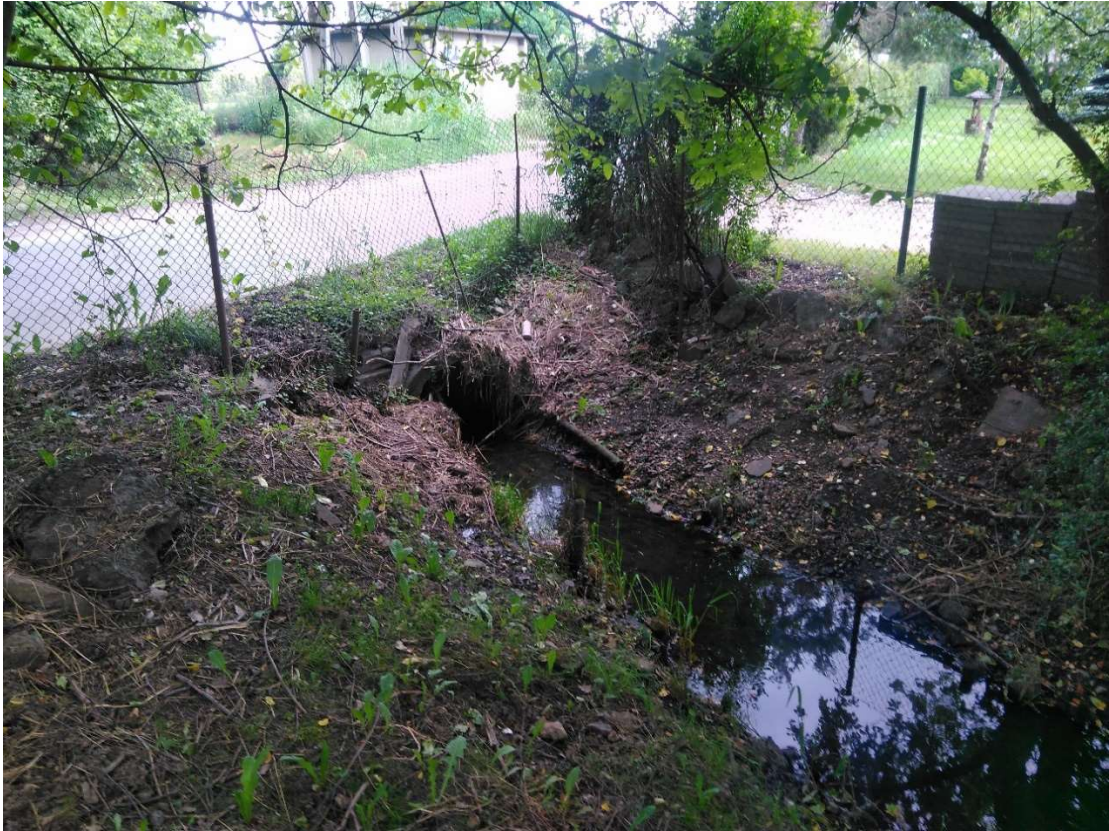
Photo. 7. Condition of the site before the start of construction – bed of the Lesisko channel.
