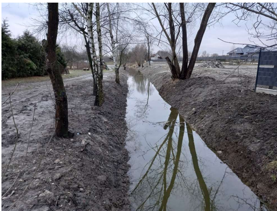
Photo. 50. Condition of the construction site in the last month of the execution of works – the reconstructed section of Ditch 2 – upper part, status in the third decade of January 2023 (view towards the west).
