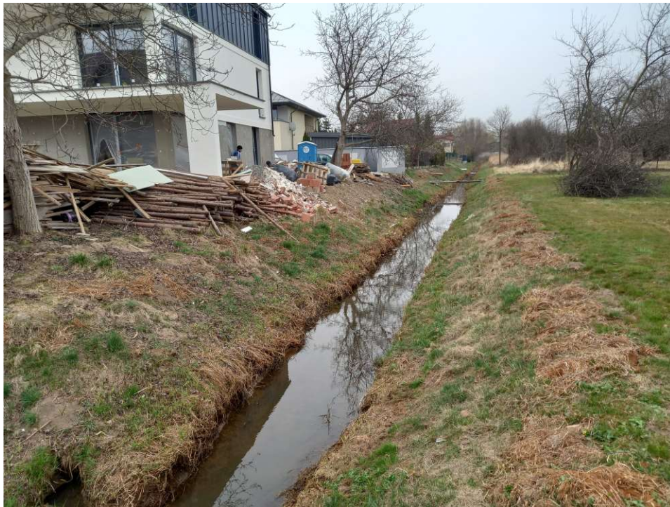
Photo. 14. Condition of the construction site in the first month of the execution of works – the reconstructed section of Ditch 2a – the upper part, status in the third decade of March 2022 (view towards the north).
