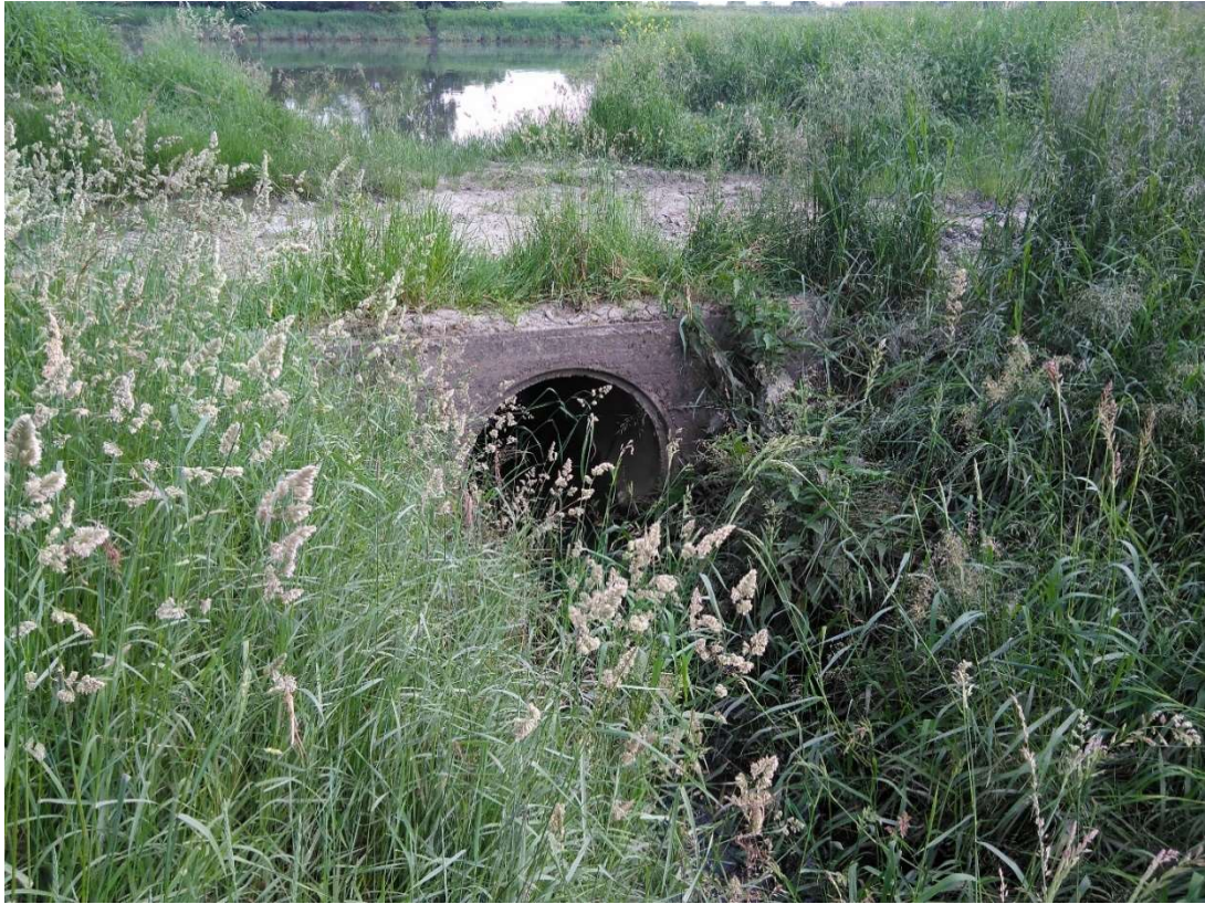
Photo. 1. Condition of the site before the start of construction – embankment culvert by which the Lesisko channel drains water to the Vistula.
