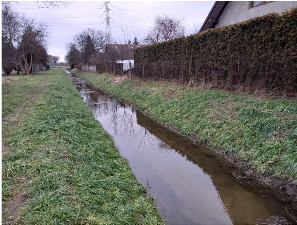
Photo. 47. Condition of the construction site in the last month of the execution of works – the reconstructed section of Ditch 2a – the lower part, status in the third decade of January 2023 (view towards the south).
