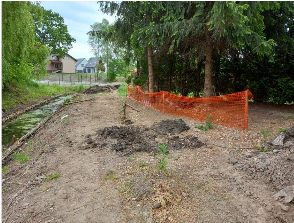
Photo. 25. Protection of trees and bushes not planned for removal in the vicinity of the construction site at Ditch 2, status in the third decade May 2022 (view towards the east).
