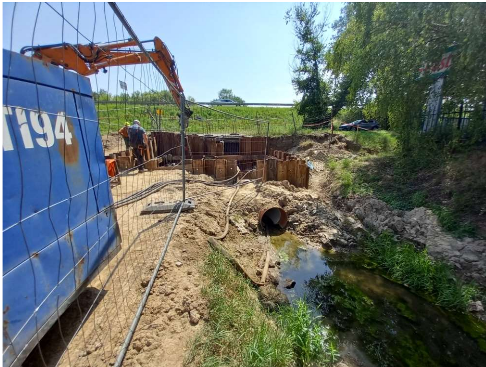
Photo. 28. Ensuring that the Ditch 2a remains unobstructed over the period of works at the embankment sluice, status in the third decade of June 2022 (view towards the south).
