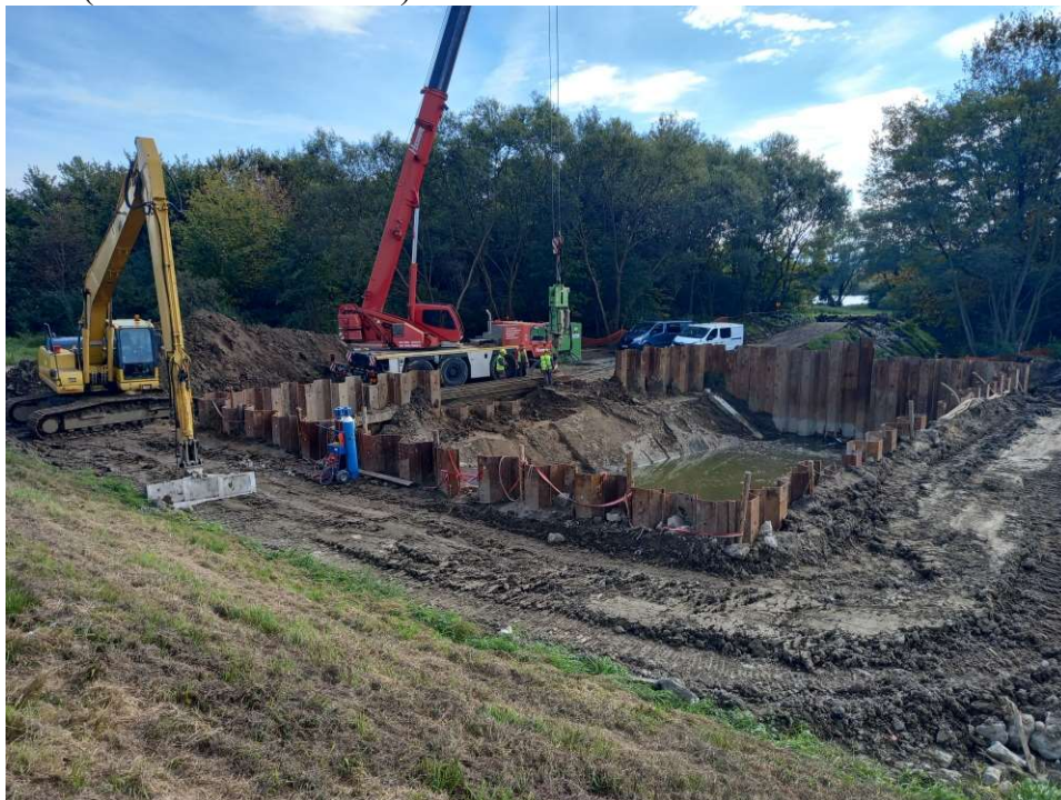
Photo. 26. Larsen works at the downstream station of the embankment sluice at Ditch 2a, status in the third decade of September 2022 (view towards the south).
