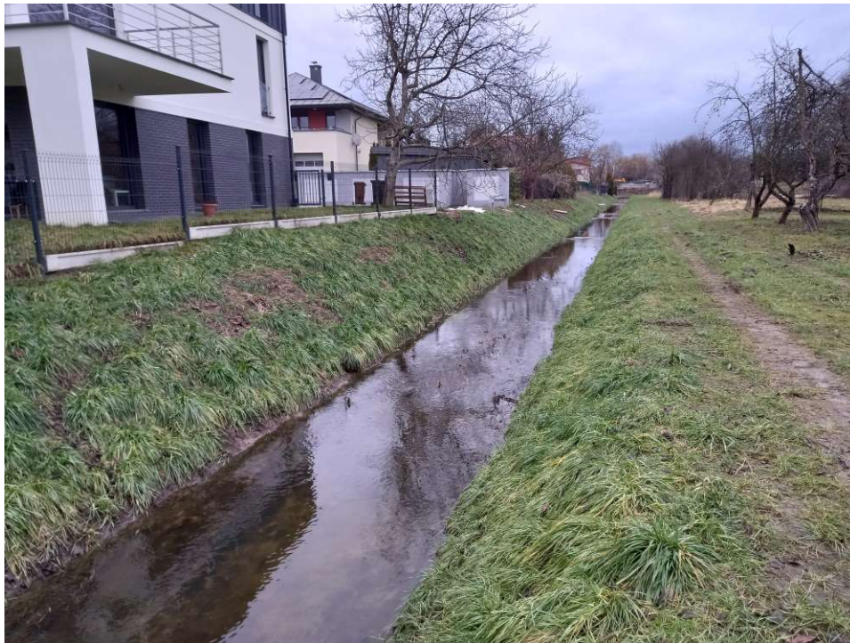
Photo. 48. Condition of the construction site in the last month of the execution of works – the reconstructed section of Ditch 2a – upper part, status in the third decade of January 2023 (view towards the north).
