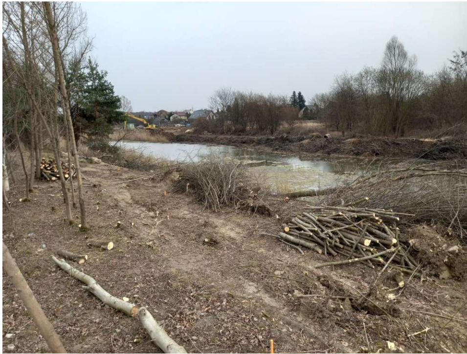
Photo. 17. Condition of the construction site in the first month of the execution of works – the reconstructed reservoir at Ditch 2, eastern part, status in the third decade of March 2022 (view towards the east).
