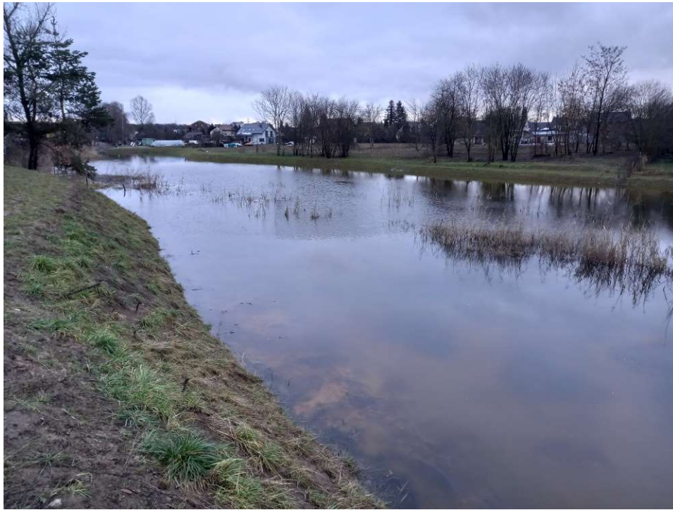
Photo. 51. Condition of the construction site in the last month of the execution of works – the reconstructed reservoir at Ditch 2, eastern part, status in the third decade of January 2023 (view towards the east).
