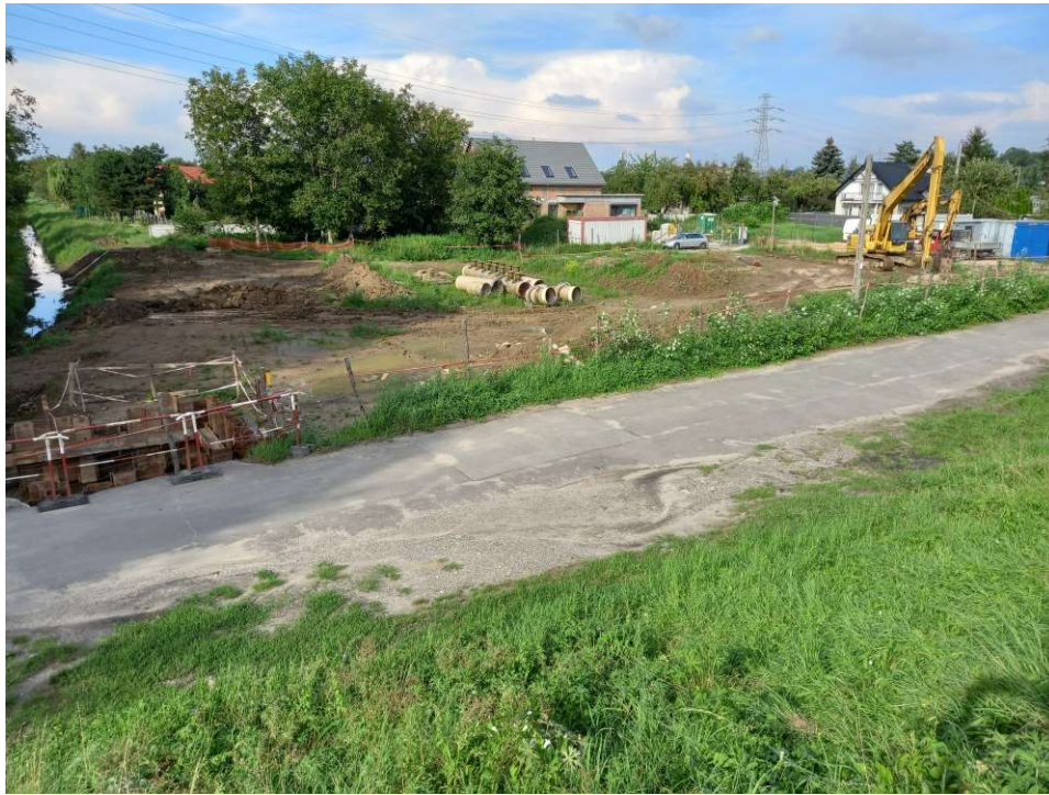
Photo. 29. Earthworks when building a storage reservoir at Ditch 2a, status in the third decade of August 2022 (view towards the north).
