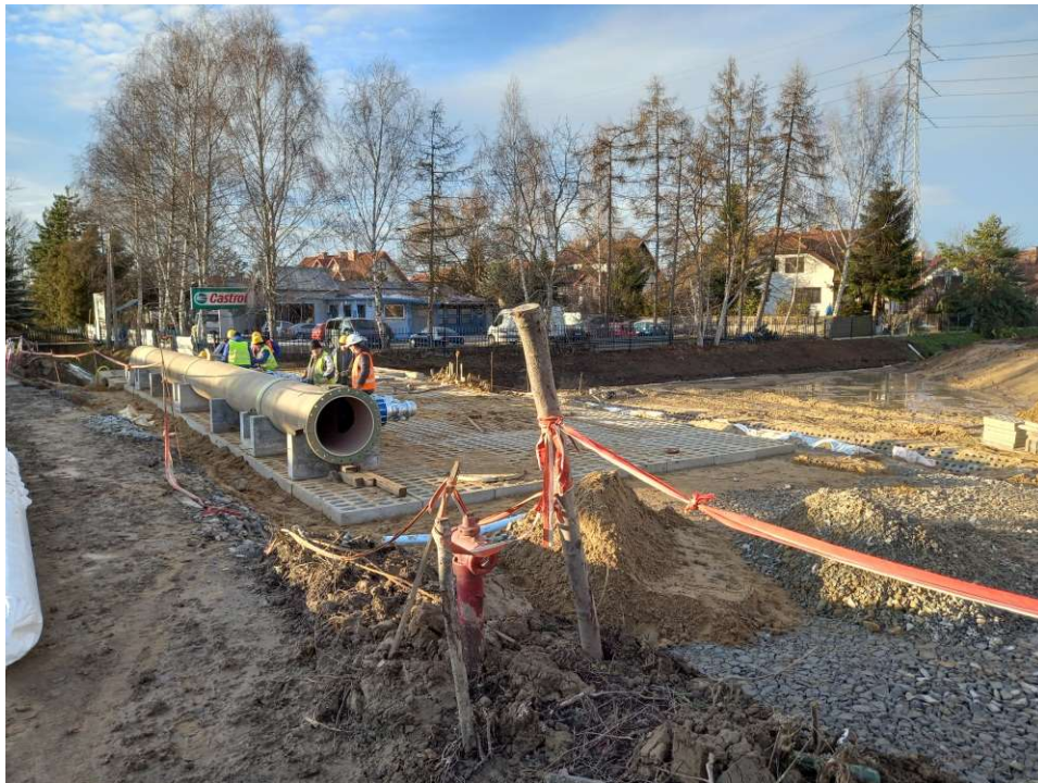
Photo. 32. Construction of a station for mobile pumps at Ditch 2a, status in the third decade of December 2022 (view towards the west).
