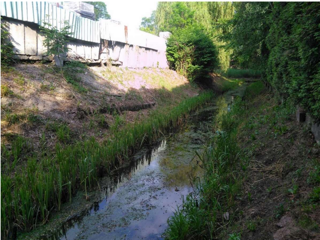
Photo. 6. Condition of the site before the start of construction – bed of the Lesisko channel.
