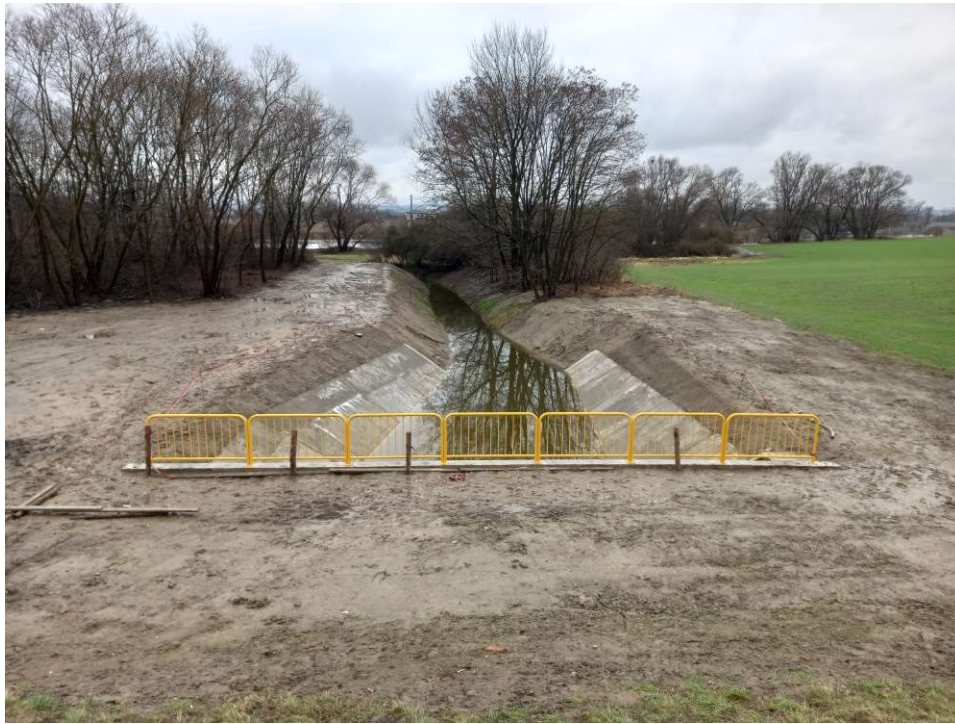
Photo. 43. Condition of the construction site in the last month of the execution of works – construction site of the embankment sluice at Ditch 2a from the side of the embanked area of the Vistula, status in the third decade of January 2023 (view towards the south).
