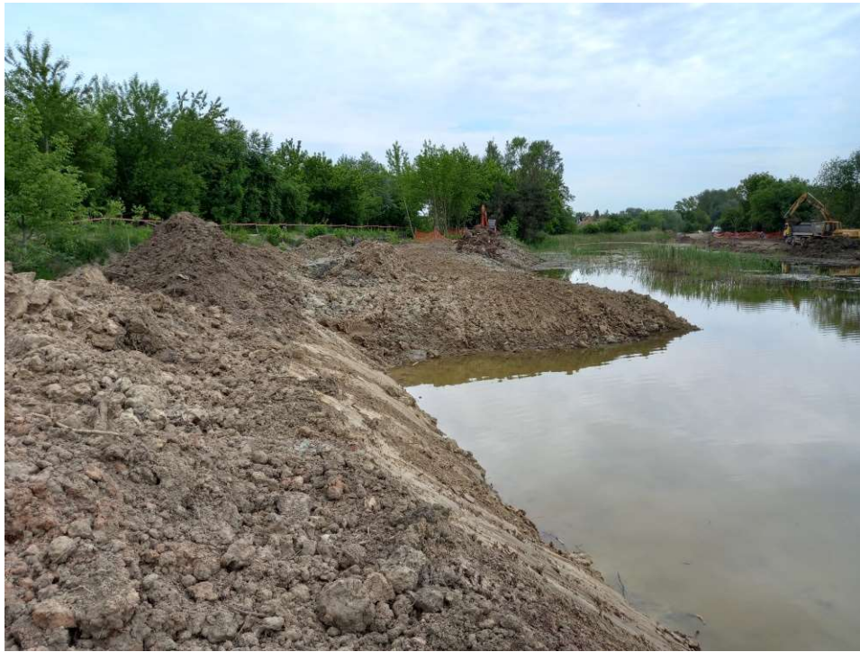
Photo. 39. Earthworks on the north bank of the enlarged reservoir at Ditch 2, status in the third decade of May 2022 (view towards the east).
