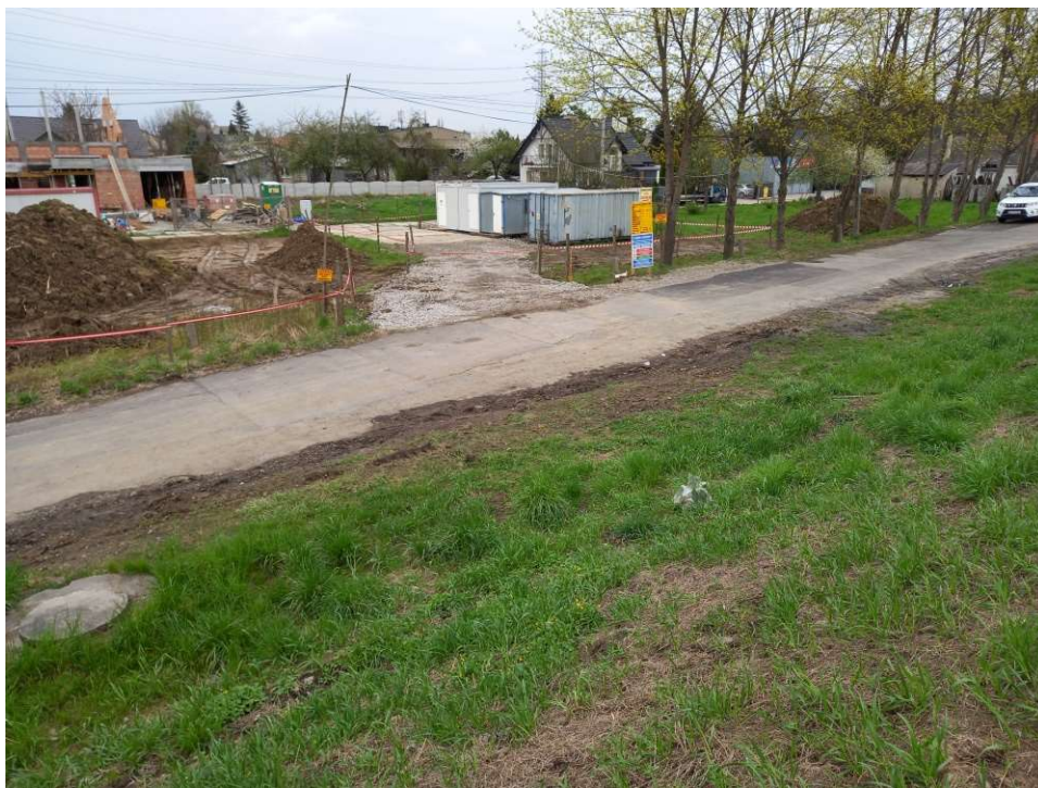
Photo. 20. Marking of the entrance to the construction site from Zagłoby Street, status in the third decade of April 2022 (view towards the north- east).
