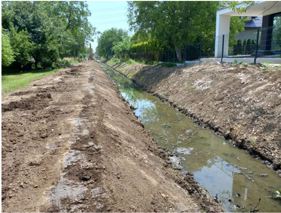
Photo. 35. Forming of bank slopes at Ditch 2a, status in the third decade of June 2022 (view towards the south).
