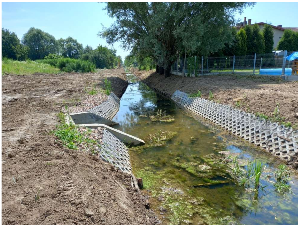
Photo. 36. Revetment of slope banks at Ditch 2a, status in the third decade of September 2022 (view towards the south).
