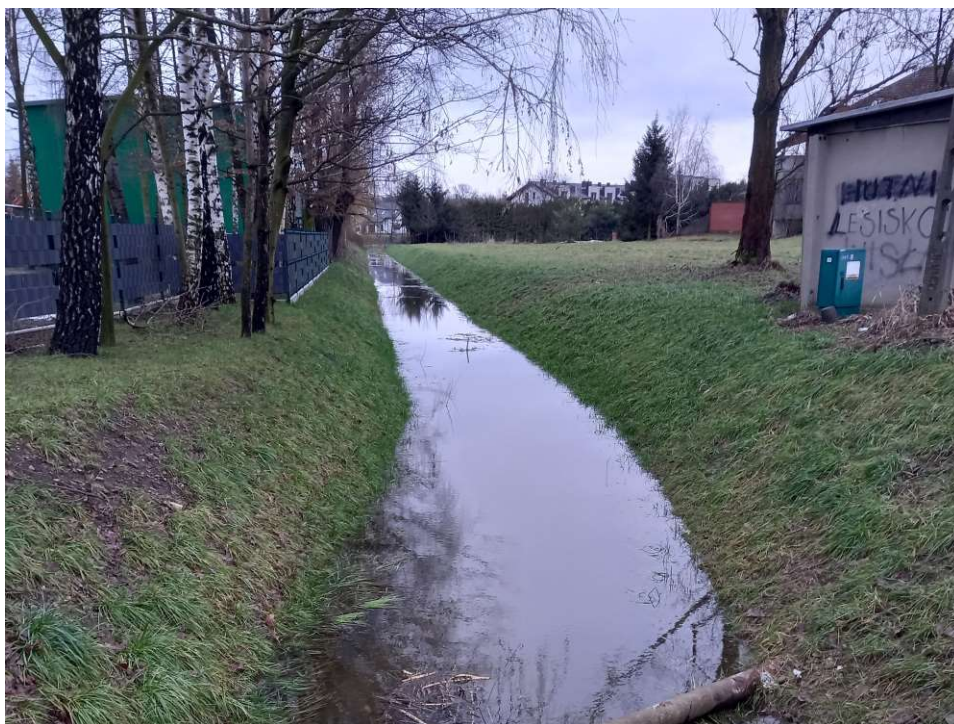
Photo. 49. Condition of the construction site in the last month of the execution of works – the reconstructed section of Ditch 2 – lower part, status in the third decade of January 2023 (view towards the east).
