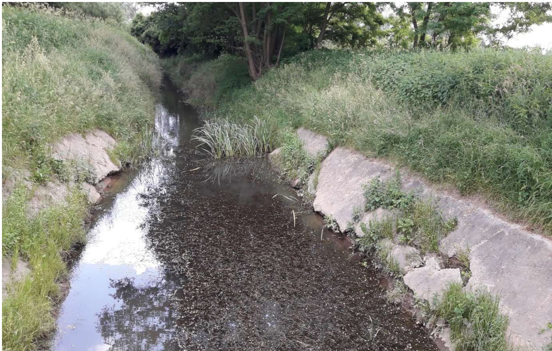
Photo. 2. Condition of the site before the start of construction – bed of the Lesisko channel.
