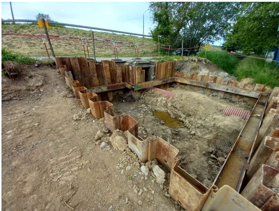
Photo. 24. Protection of hazardous places on the construction site of the embankment sluice at Ditch 2a at the area beyond the embankment of the Vistula River, status in the third decade of July 2022 (view towards the north).
