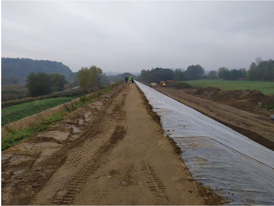
Photo. 30. Placement of bentonite mat on the flood protection embankment slope for Task 3, condition in the third decade of 2020 (upstream view).
