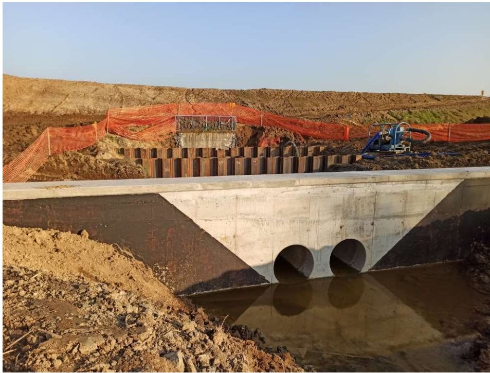
Photo. 22. Reconstruction of the embankment culvert at km 61+239 of the embankment of the Vistula River for Task 1, condition in the third decade of November 2020 (view from the embanked area).
