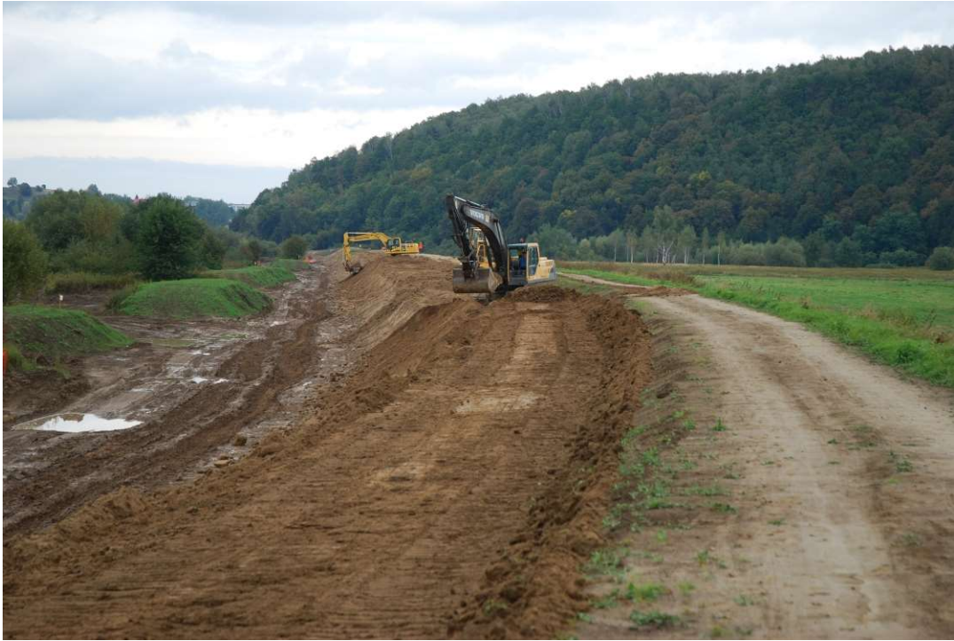
Photo. 28. Forming of slopes of flood protection embankment for Task 1, condition in the third decade of September 2020 (downstream view).
