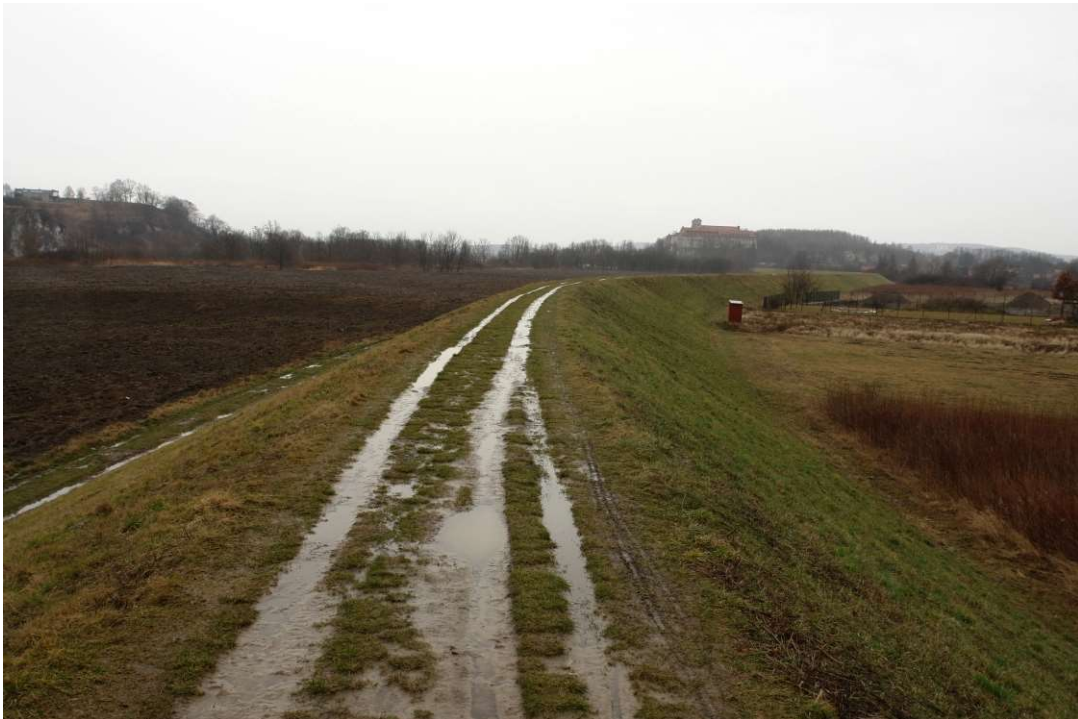
Photo. 6. Condition of the Construction Site before the start of works - the right embankment of the Vistula River planned for reconstruction for Task 2, the condition in the third decade of February 2020 (downstream view).
