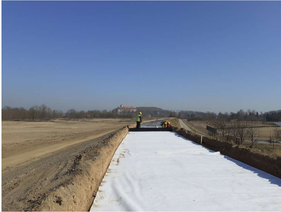
Photo. 34. Construction of the road on crest of the flood protection embankment for Task 2, condition in the third decade of March 2022 (downstream view).
