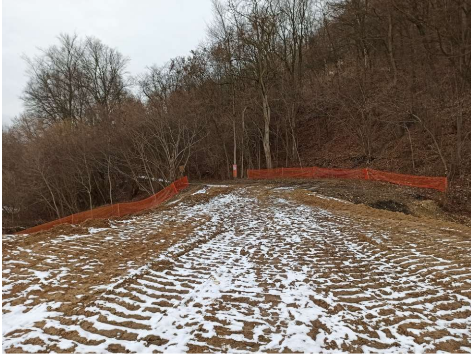
Photo. 15. Protection of trees and bushes not planned for removal for Task 1, condition in the third decade of January 2021 (downstream view).
