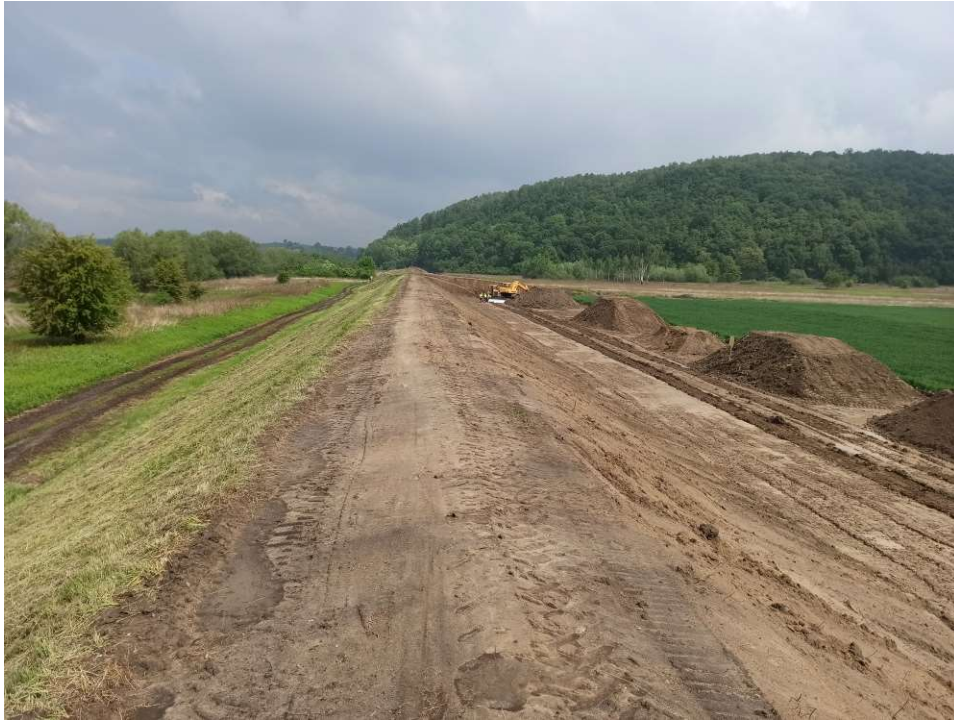
Photo. 20. Protection of the topsoil piles for Task 1, condition in the third decade of May 2020 (downstream view).
