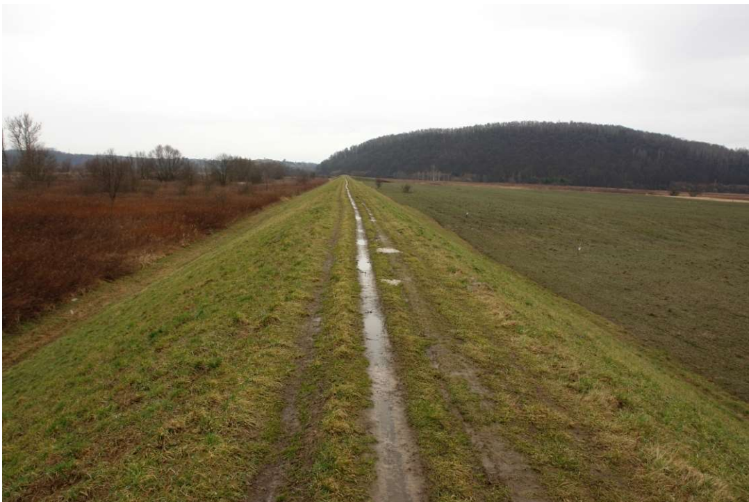
Photo. 2. Condition of the Construction Site before the start of works - the right embankment of the Vistula River planned for reconstruction for Task 1, the condition in the third decade of February 2020 (downstream view).
