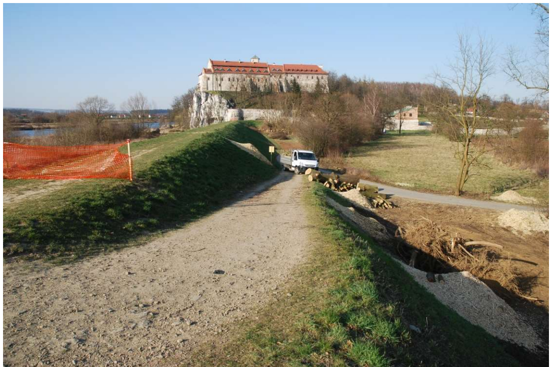
Photo. 10. Tidying-up of the area after removal of trees for Task 2, condition in the third decade of March 2020 (downstream view).
