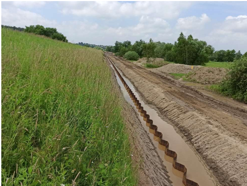
Photo. 25. Construction of the membrane made of sheet piles for Task 3, condition in the third decade of June 2020 (upstream view).
