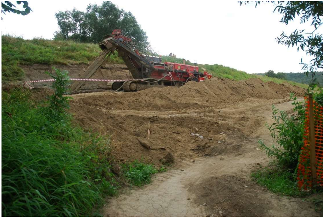
Photo. 26. Construction of the cement-bentonite membrane for Task 2, condition in the third decade of August 2020 (upstream view).
