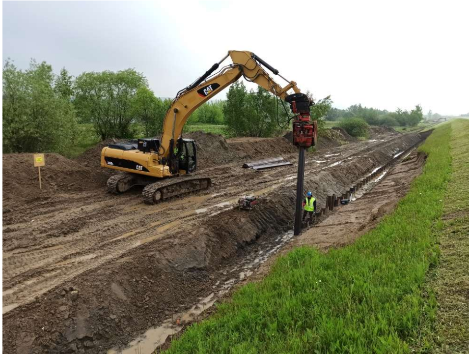
Photo. 24. Construction of the membrane made of sheet piles for Task 3, condition in the third decade of May 2020 (downstream view).
