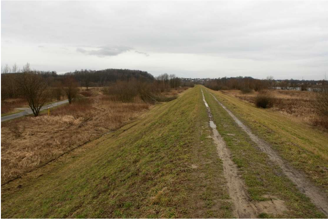
Photo. 7. Condition of the Construction Site before the start of works - the right embankment of the Vistula River planned for reconstruction for Task 3, the condition in the third decade of February 2020 (upstream view).
