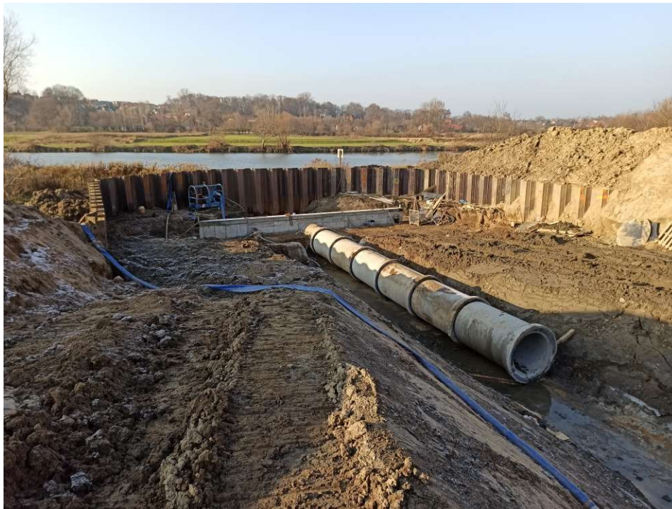
Photo. 23. Reconstruction of the embankment culvert at km 63+115 of the embankment of the Vistula River for Task 2, condition in the third decade of November 2020 (view towards the embanked area).
