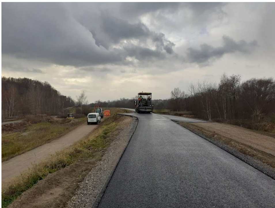
Photo. 35. Construction of the road on crest of the flood protection embankment for Task 3, condition in the third decade of November of 2021 (upstream view).
