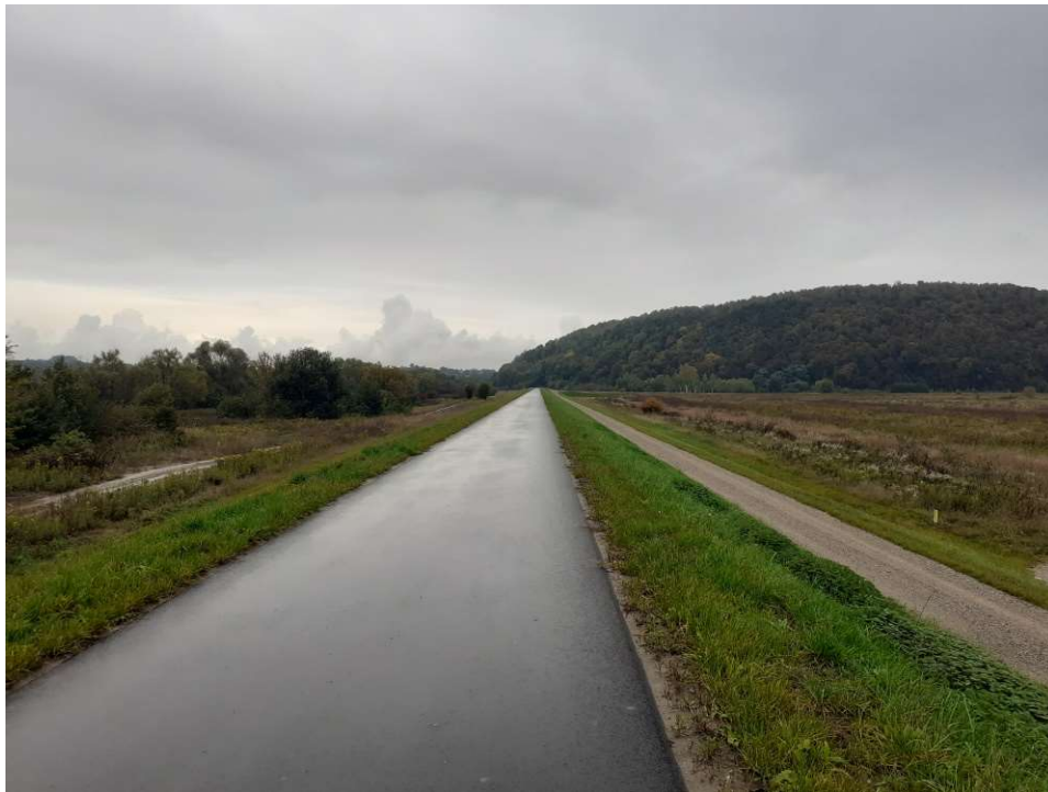
Photo. 39. Condition of the construction site in the last month of the period of execution of works – the right embankment of the Vistula River for Task 1, condition in the third decade of September 2022 (downstream view).
