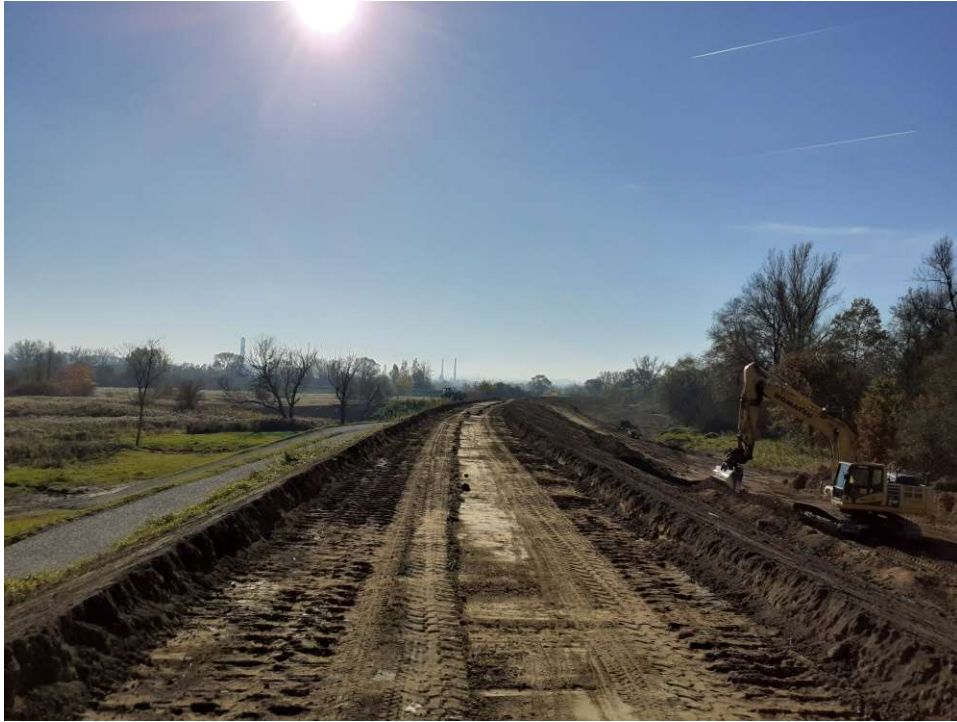
Photo. 32. Topsoiling of slopes of the flood protection embankment for Task 1, condition in the third decade of October 2021 (upstream view).
