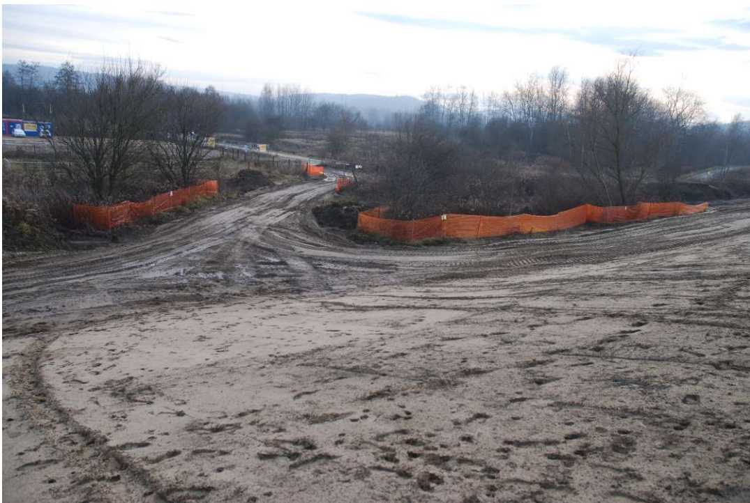
Photo. 17. Protection of trees and bushes not planned for removal for Task 3, condition in the third decade of December 2020 (view towards the area beyond the embankment).
