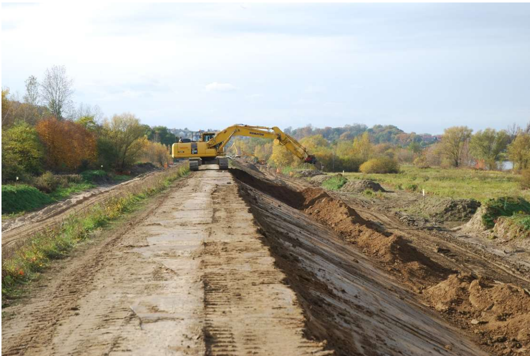
Photo. 29. Forming of slopes of flood protection embankment for Task 3, condition in the third decade of September 2020 (upstream view).
