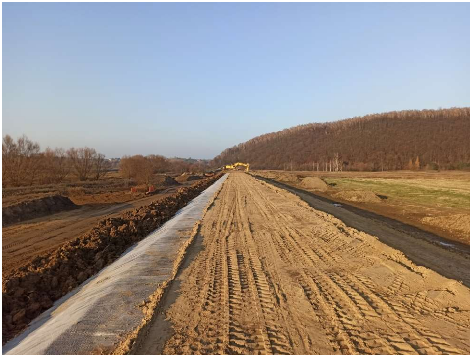
Photo. 31. Placement of bentonite mat on the flood protection embankment slope for Task 1, condition in the third decade of November 2020 (downstream view).
