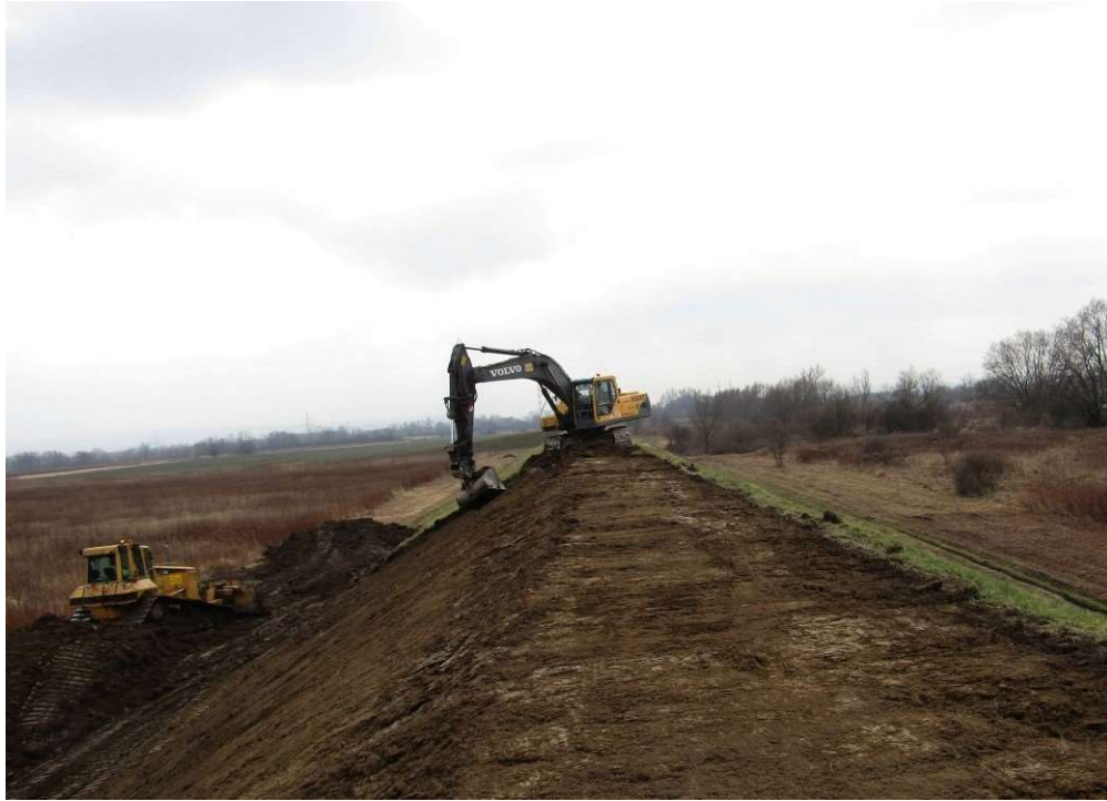
Photo. 18. Removal of the topsoil layer for Task 1, condition in the third decade of February 2020 (upstream view).
