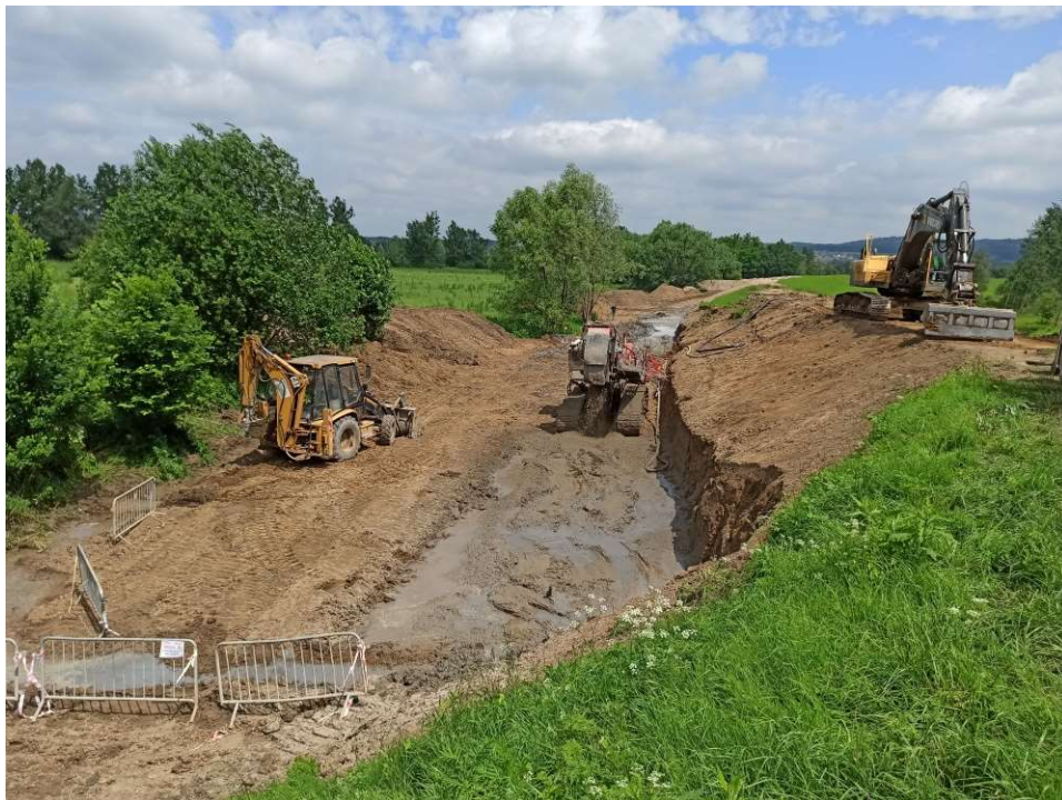
Photo. 27. Construction of the cement-bentonite for Task 3, condition in the third decade of June 2020 (downstream view).
