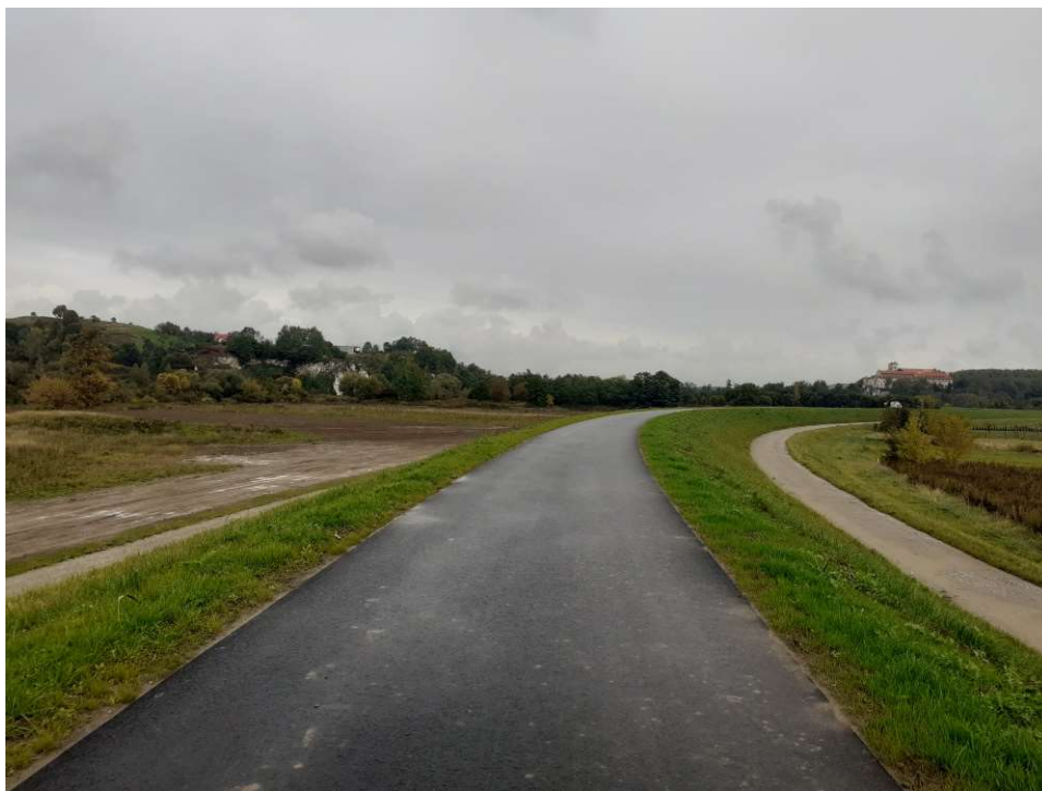
Photo. 41. Condition of the construction site in the last month of the period of execution of works – the right embankment of the Vistula River for Task 2, condition in the third decade of September 2022 (downstream view).
