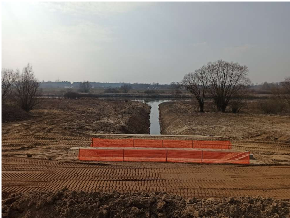
Photo. 14. Protection of hazardous places for Task 1, condition in the third decade of March 2021 (view towards the embanked area).
