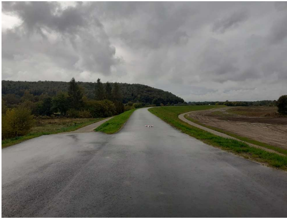
Photo. 40. Condition of the construction site in the last month of the period of execution of works – the right embankment of the Vistula River for Task 2, condition in the third decade of September 2022 (upstream view).
