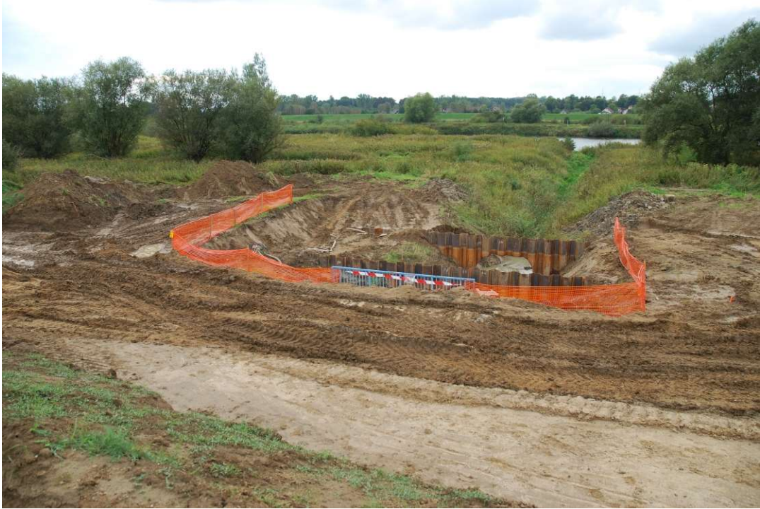
Photo. 13. Protection of hazardous places for Task 1, condition in the third decade of September 2020 (view towards the embanked area).
