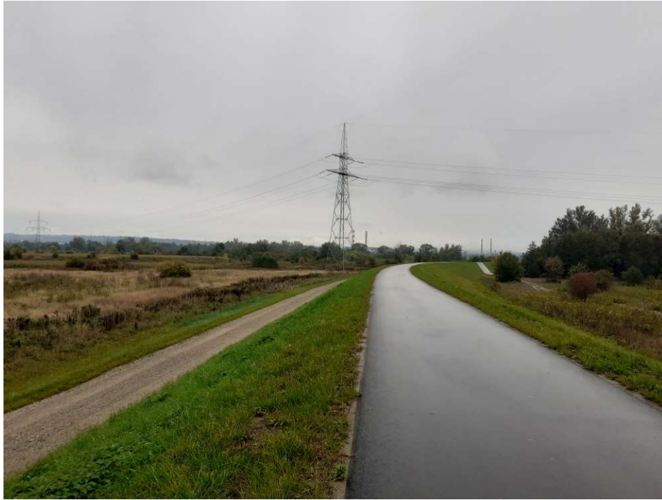
Photo. 38. Condition of the construction site in the last month of the period of execution of works – the right embankment of the Vistula River for Task 1, condition in the third decade of September 2022 (upstream view).
