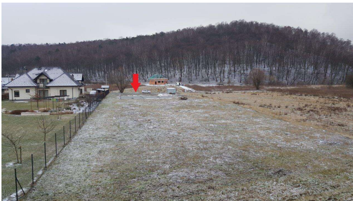
Photo. 4. Condition of the Construction Site before the start of works – foundations located on land property no. 197/6 (197/1 before split-up).
