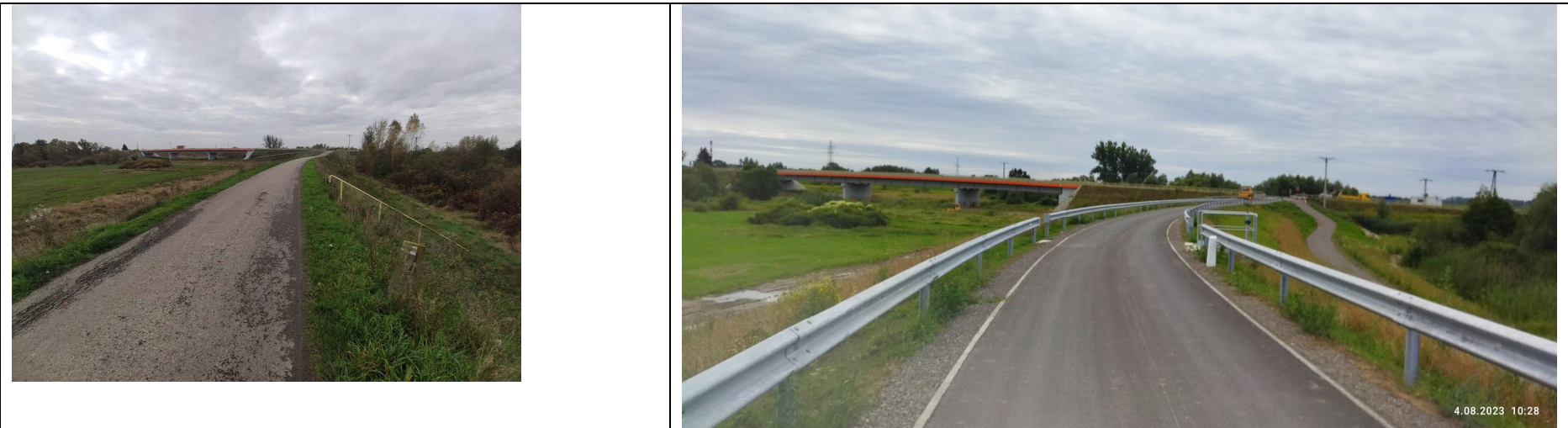
Photo no. 5: Culvert, gate valve on the watercourse running through the embankment, with a view of the bridge over the Łęg river in the background, DK 77 (Sandomierska Street)
