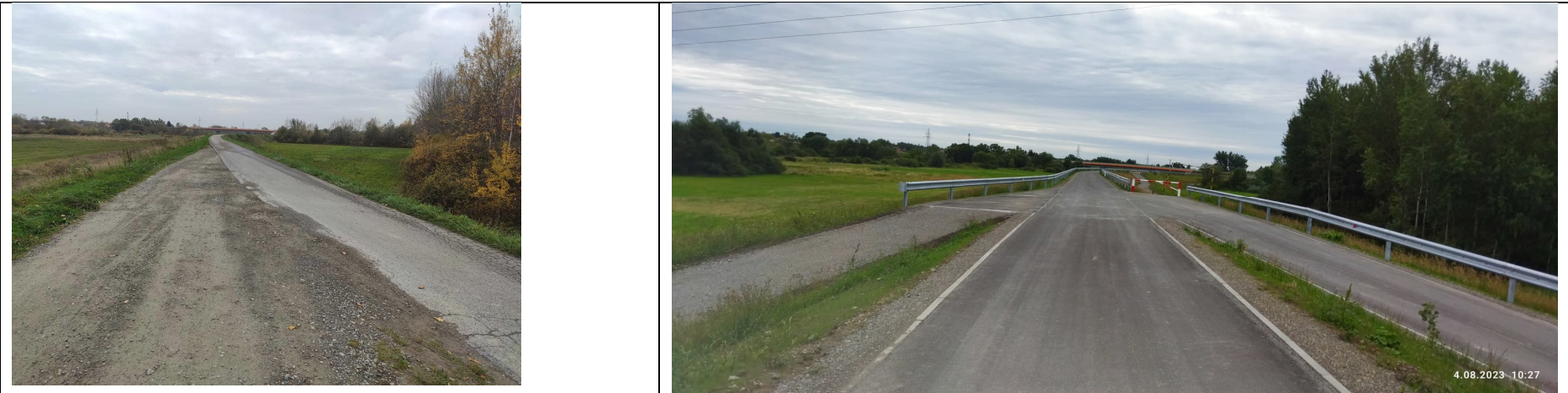
Photo no. 4: Crossroad – gravel road and asphalt road, running along the top of the embankments.
