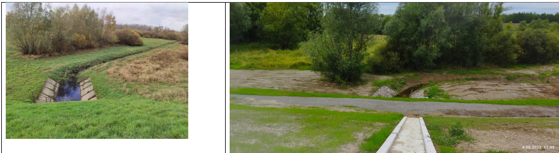
Photo no. 17: Drainage from the culvert on the side of the embanked area (Podwale Street).
