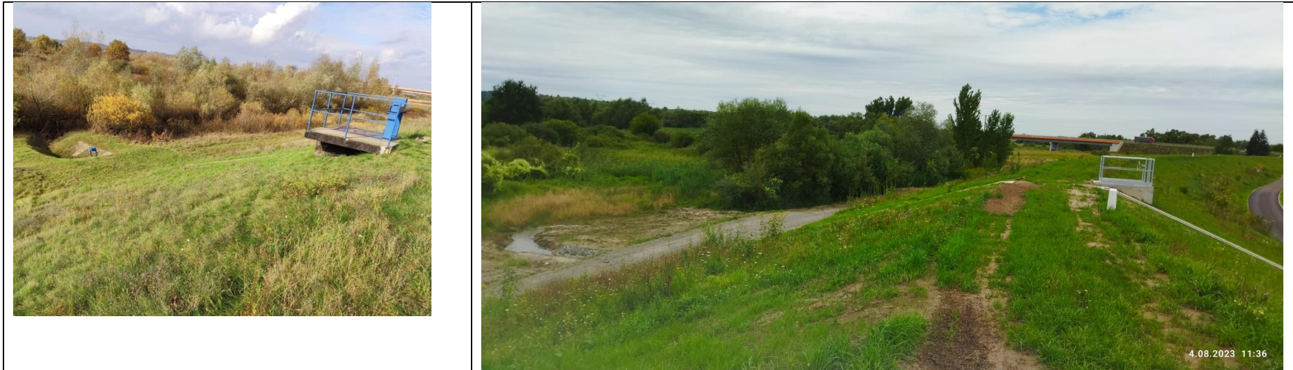
Photo no. 11: Embankment culvert, gate valve.
