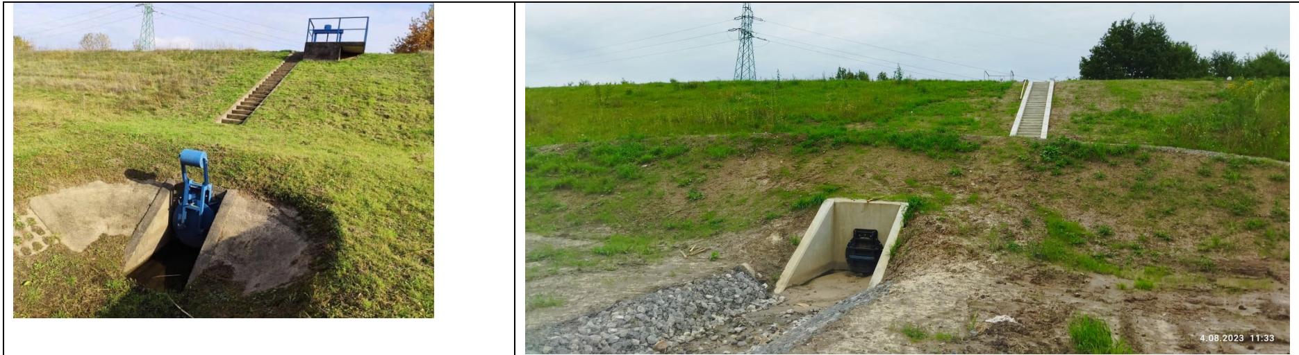
Photo no. 12: Culvert on the side of the embanked area, gate valve, HV line to be reconstructed in the distance.
