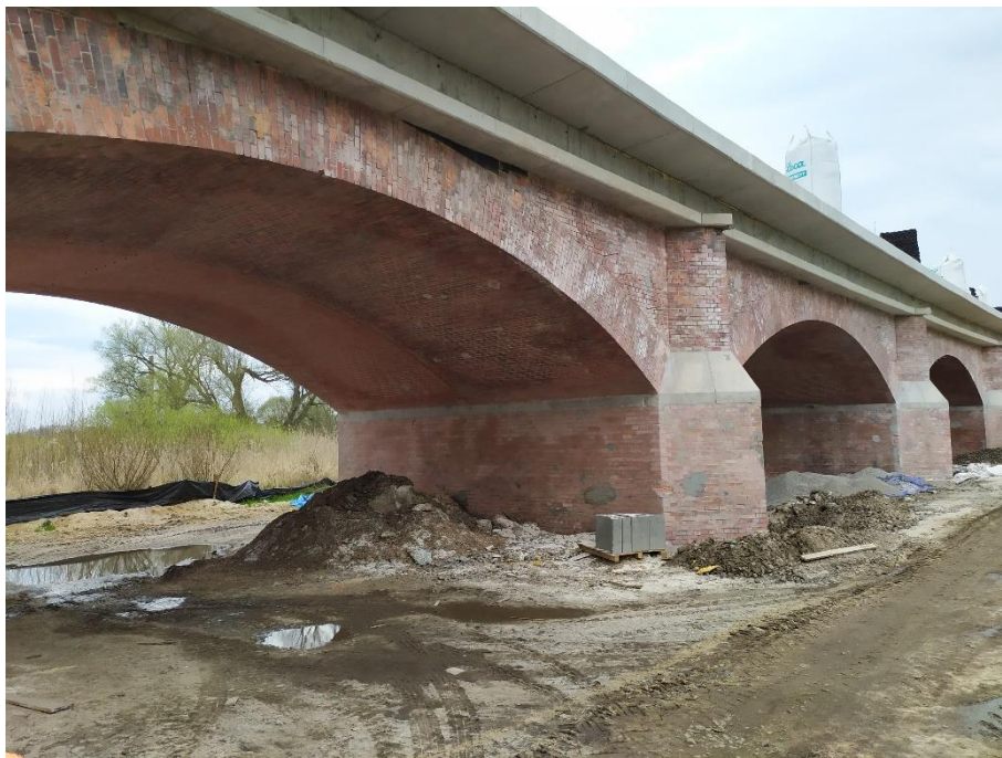
Photo 10. Bridge over Suchodół – an object included in the provincial records of monuments.
