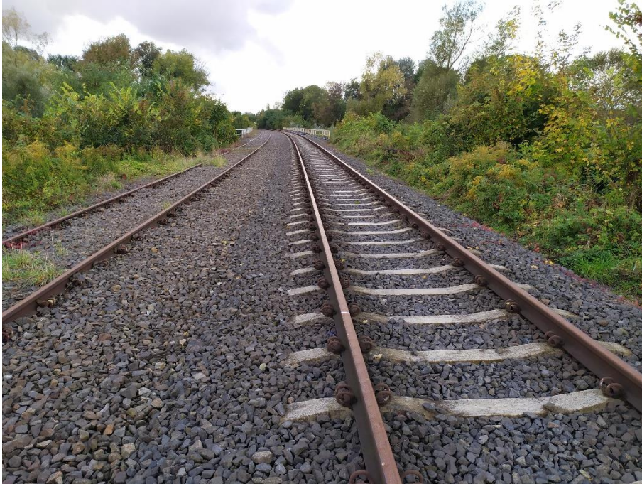
Photo 1. Track in the central part of the Task prior to the start of works.
