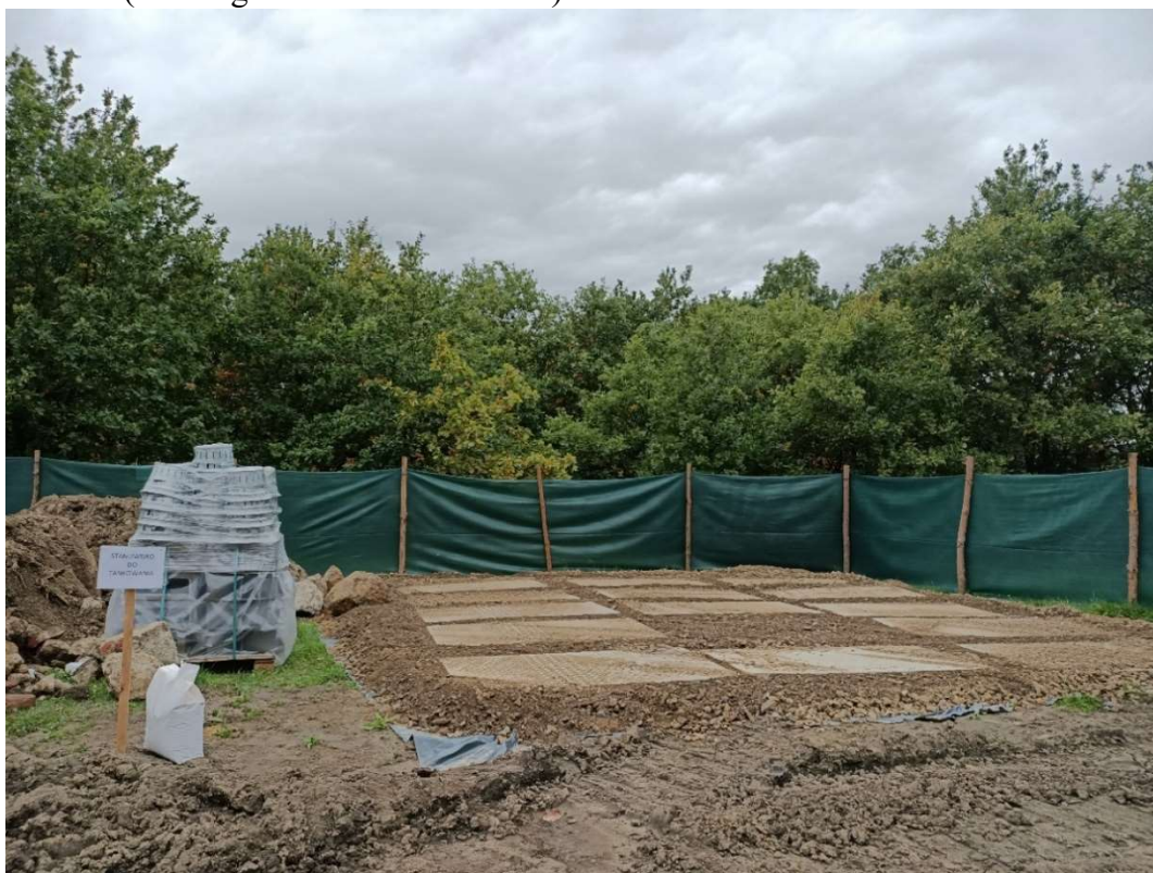
Foto. 2. Służowjskie Street , first decade of October 2022 (place for refueling vehicles in the back-up area of the Construction Site).
