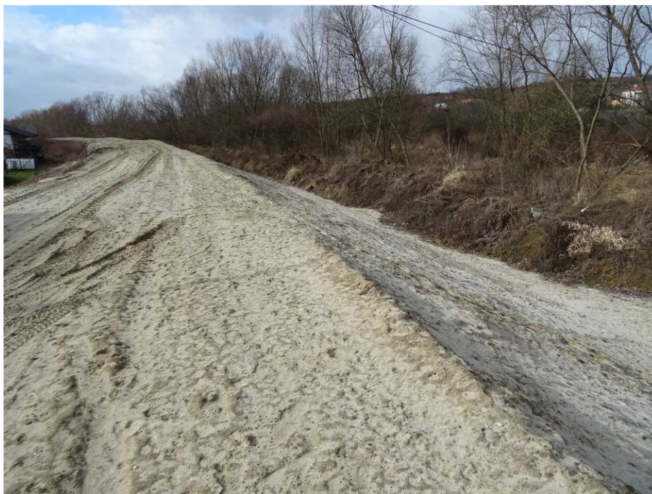
Fig. 7. Site condition in the first quarter of the works implementation period on Task 4 – right bank of Koprzywnianka river upstream of the footbridge in Koprzywnica, status in the third decade of February 2020 (upstream view).
