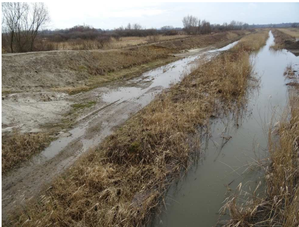
Fig. 5. Site condition in the first quarter of the works implementation period on Task 4 – right bank of Koprzywianka river upstream of the bridge on the road Szewce-Skotniki, status in the third decade of February 2020 (upstream view).
