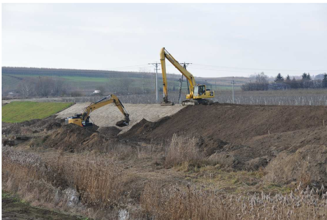
Fig. 40. Covering slopes of the flood embankment with a top-soil layer – left bank of Koprzywianka river upstream of the bridge on the road Samborzec-Zajeziórze, status in the first decade of December 2020 (upstream view).
