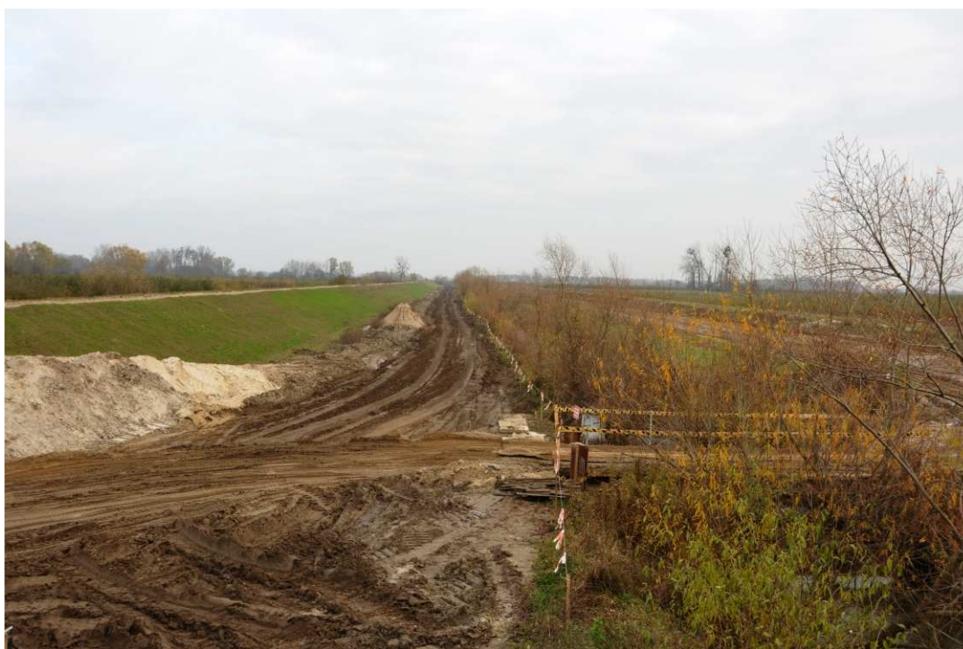
Fig. 18. Protection of trees and shrubs not intended to felling – left bank of Koprzywianka river downstream of the bridge on the road Sośniczany-Skotniki, status in the second decade of November 2020 (downstream view).
