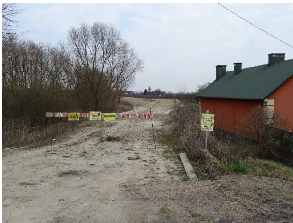
Fig. 12. Marking of the construction site – right bank of Koprzywnianka river downstream of the bridge on the road no. 758 in Koprzywnica, status in the second decade of March 2020 (downstream view).
