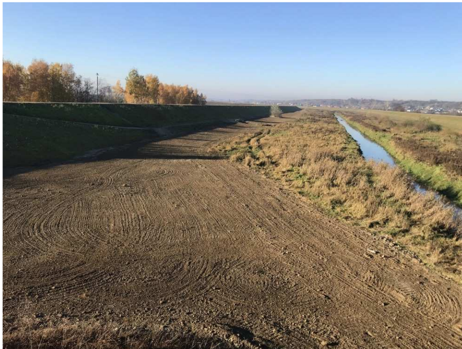
Fig. 45. Reclamation of the area between the Koprzywianka embankments – right bank of Koprzywianka river upstream of the bridge on the road Andruszkowice-Koćmierzów, status in the third decade of October 2021 (upstream view).
