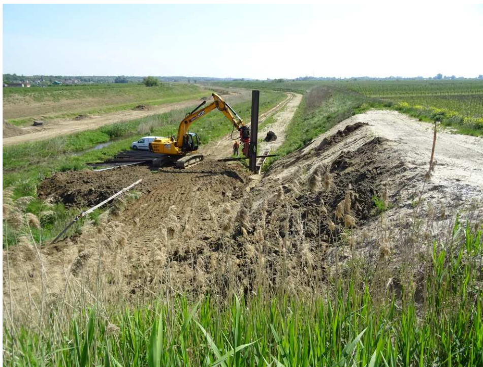
Fig. 27. Driving the sheet piles at the base of the embankment – right bank of Koprzywianka river downstream of the bridge on the road Złota-Zawierzbie, status in the second decade of May 2020 (downstream view).
