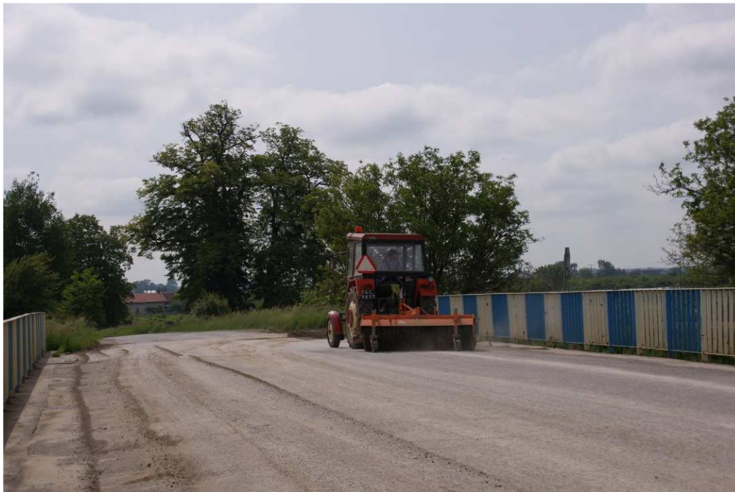
Fig. 21. Keeping public roads clean in the vicinity of the construction site – bridge on the road Samborzec-Zajeziorko, status in the second decade of June 2020 (view towards the south-east).
