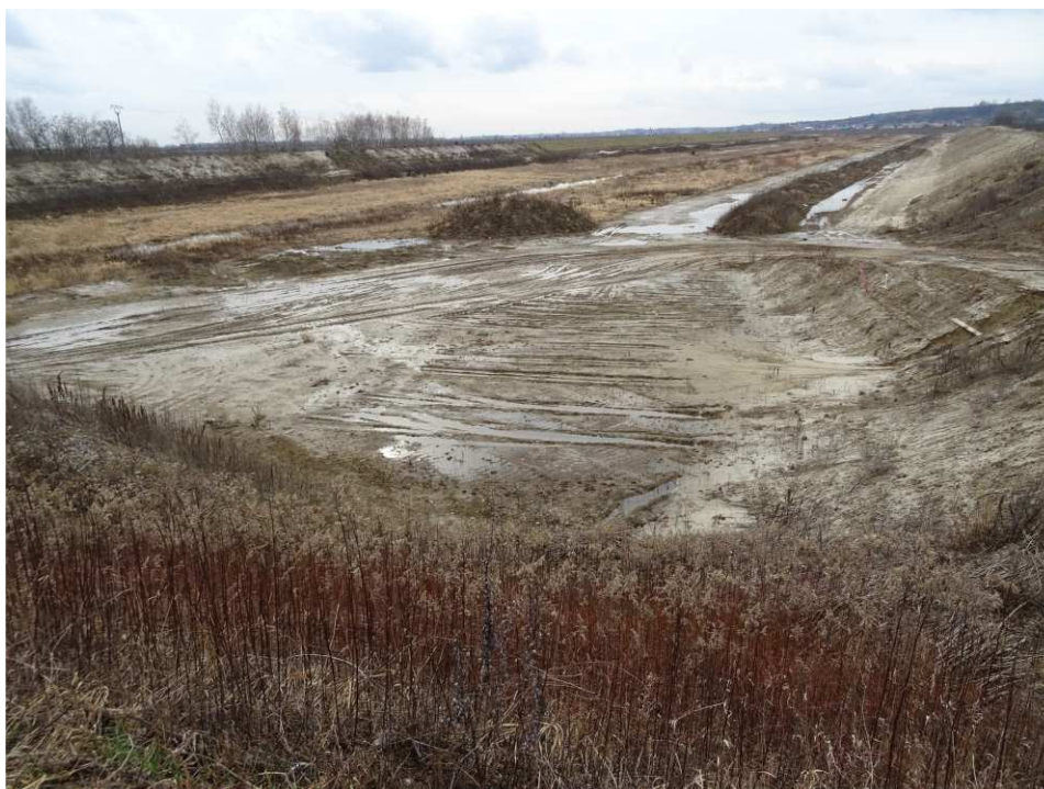
Fig. 2. Site condition in the first quarter of the works implementation period on Task 4 – banks of Koprzywianka river upstream of the bridge on the road Andruszkowice-Koćmierzów, status in the third decade of February 2020 (upstream view).
