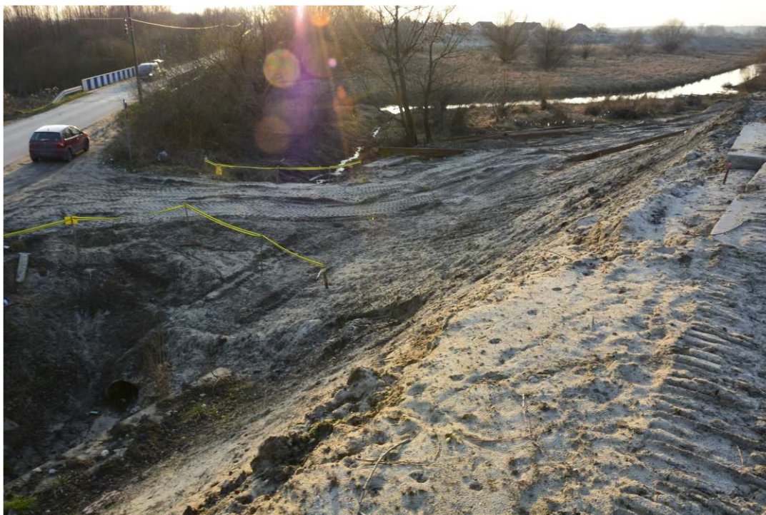
Fig. 15. Protection of hazardous sites – left bank of Koprzywianka river upstream of the bridge on the road Sandomierz-Zawisielcze, status in the second decade of January 2021 (upstream view).
