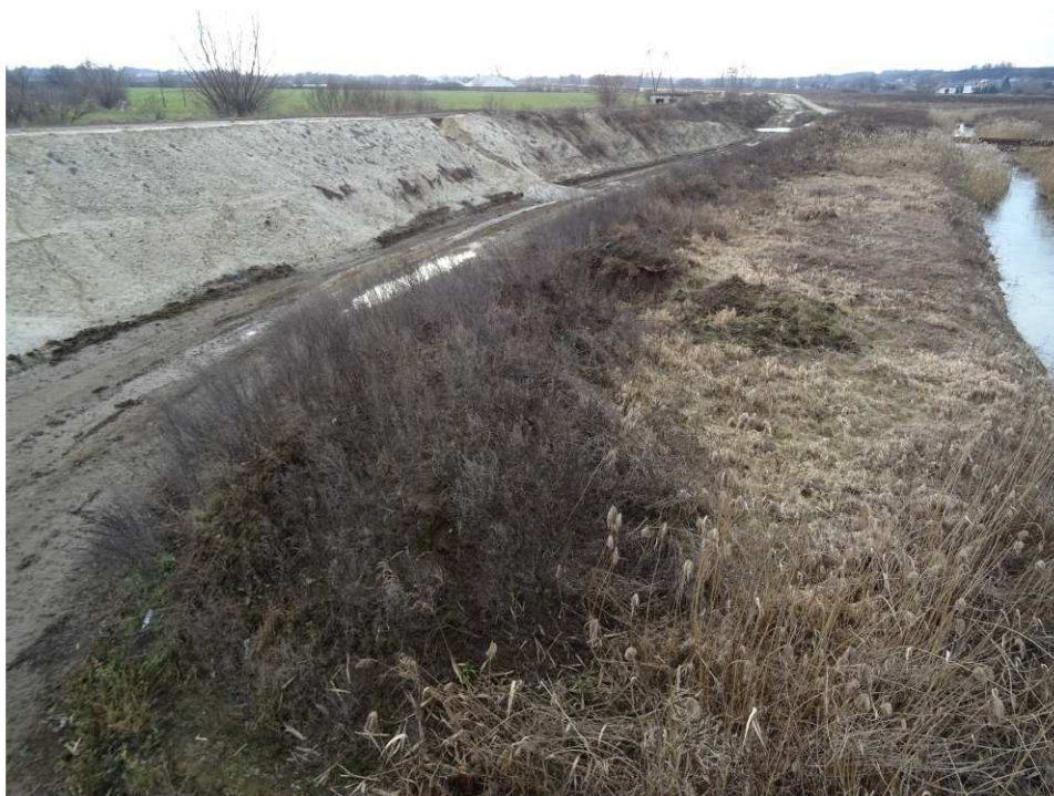
Fig. 4. Site condition in the first quarter of the works implementation period on Task 4 – right bank of Koprzywianka river upstream of the bridge on the road Samborzec-Zajeziorsze, status in the third decade of February 2020 (upstream view).
