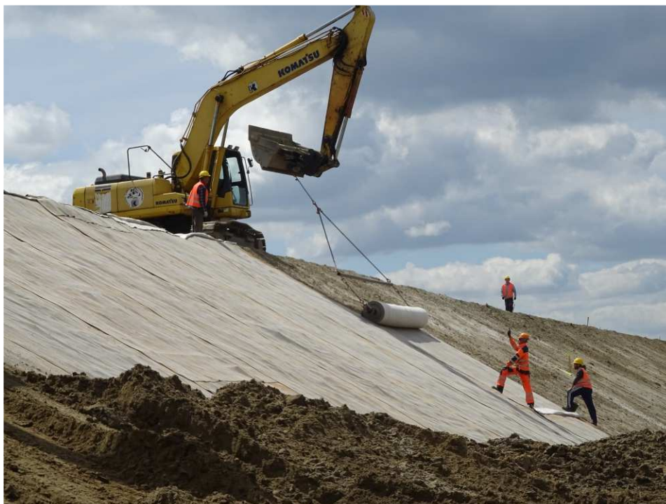
Fig. 37. Placement of bentomat on the slope of the flood embankment – left bank of Koprzywianka river downstream of the bridge on the road Andruszkowice-Koćmierzów, status in the second decade of May 2020 (downstream view).
