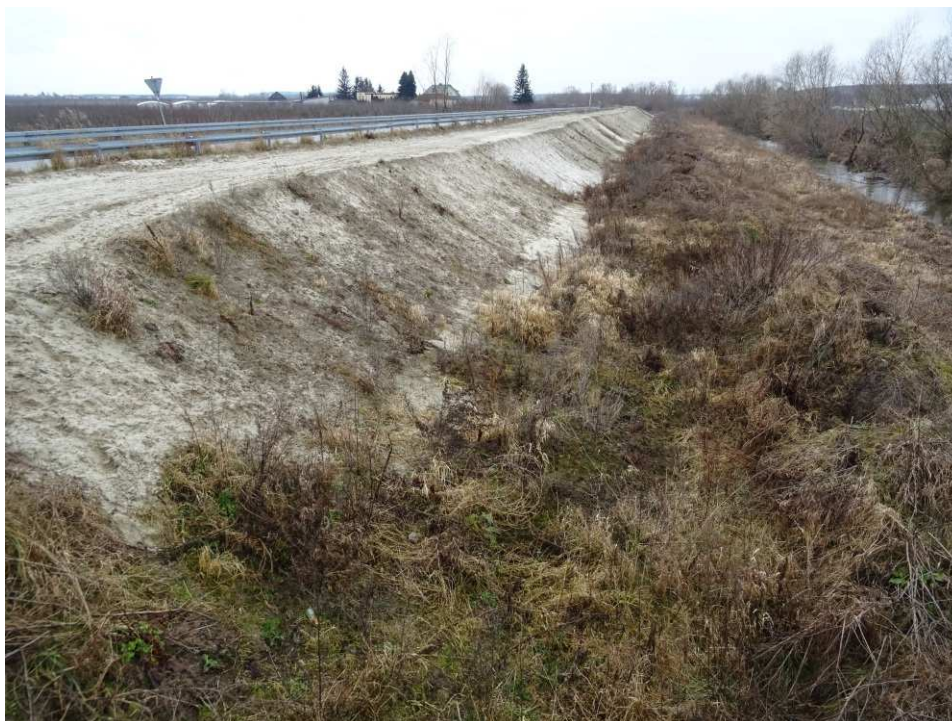
Fig. 6. Site condition in the first quarter of the works implementation period on Task 4 – right bank of Koprzywianka river upstream of the bridge on the road Sośniczany-Skotniki, status in the third decade of February 2020 (upstream view).
