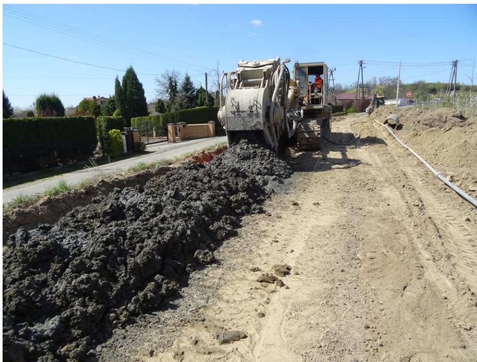
Fig. 25. Construction of a cement-bentonite barrier – right bank of Polanówka stream downstream of the bridge on the road Kraków-Sandomierz, status in the third decade of April 2020 (upstream view).
