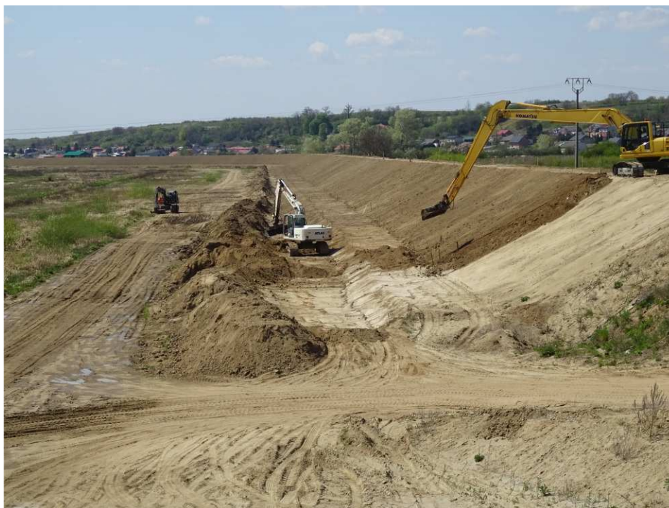
Fig. 39. Covering slopes of the flood embankment with a top-soil layer – left bank of Koprzywianka river upstream of the bridge on the road Andruszkowice-Koćmierzów, status in the third decade of April 2020 (upstream view).
