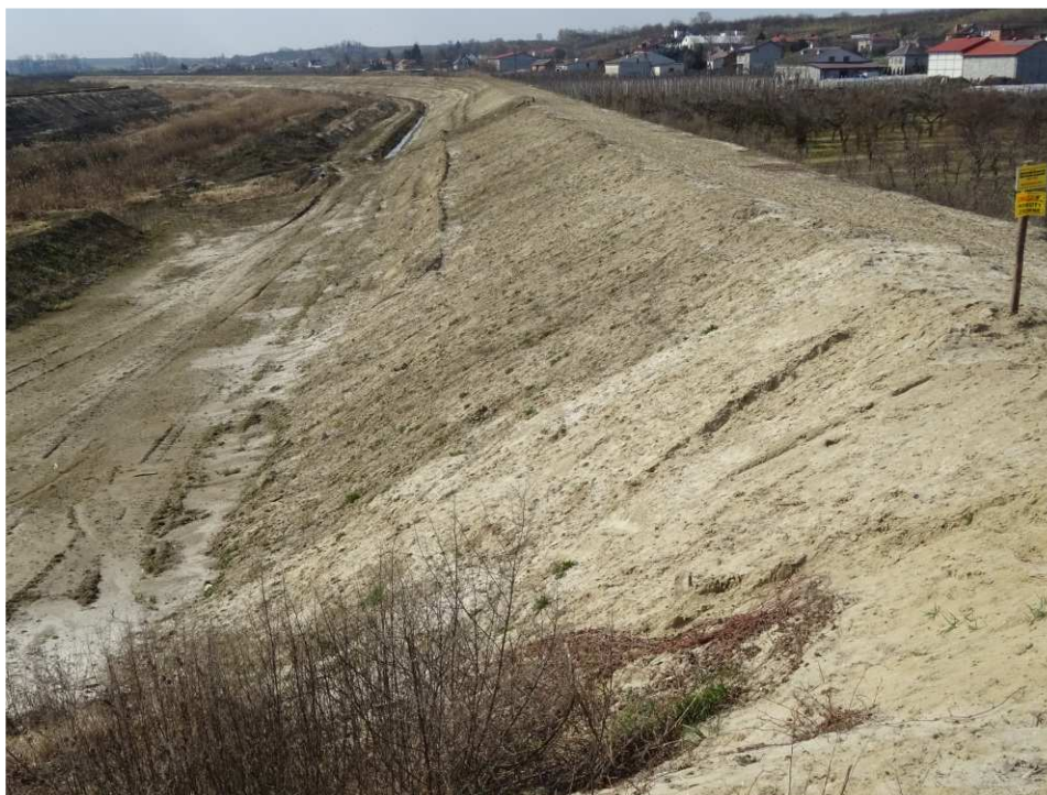
Fig. 3. Site condition in the first quarter of the works implementation period on Task 4 – left bank of Koprzywianka river upstream of the bridge on the road Złota-Zawierzbie, status in the third decade of March 2020 (upstream view).
