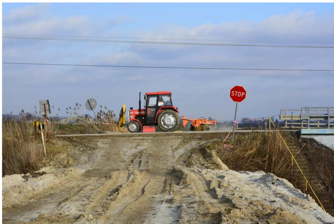
Fig. 22. Keeping public roads clean in the vicinity of the construction site – access road to the bridge on the road Szewce-Skotniki, status in the second decade of January 2021 (downstream view).
