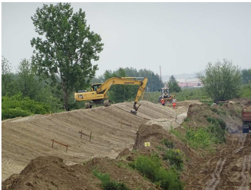
Fig. 36. Compaction of the body of the flood embankment – left bank of Koprzywianka river downstream of the bridge on the road Sośniczany-Skotniki, status in the third decade of May 2020 (downstream view).
