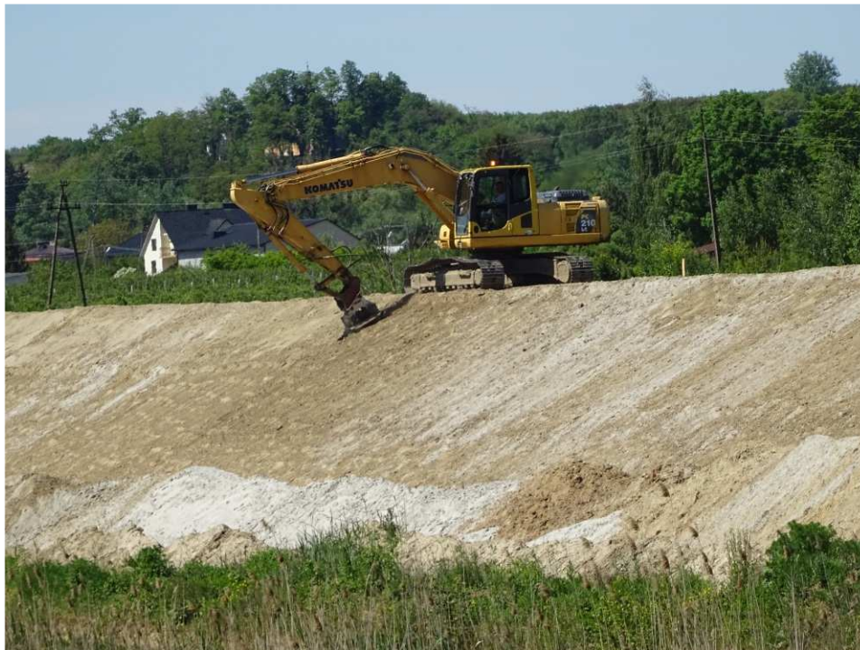
Fig. 35. Compaction of the body of the flood embankment – left bank of Koprzywianka river upstream of the bridge on the road Złota-Zawierzbie, status in the third decade of May 2020 (upstream view).
