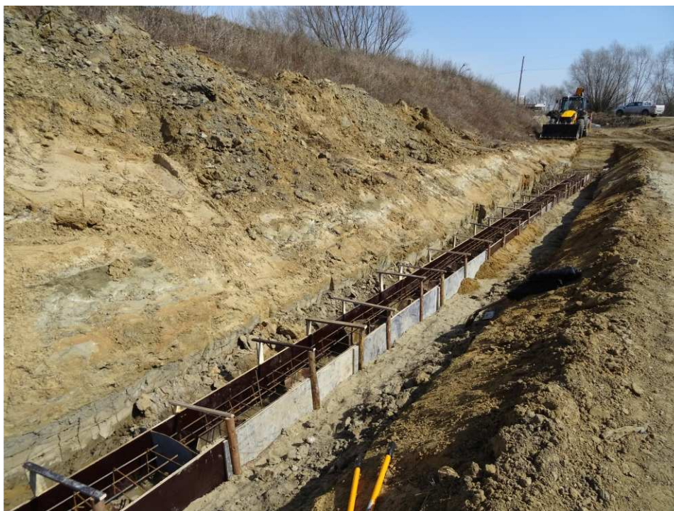
Fig. 28. Making a cap on the sheet pilings at the base of the embankment – left bank of Koprzywianka river upstream of the bridge on the road Sandomierz-Zawisielcze, status in the third decade of March 2020 (downstream view).
