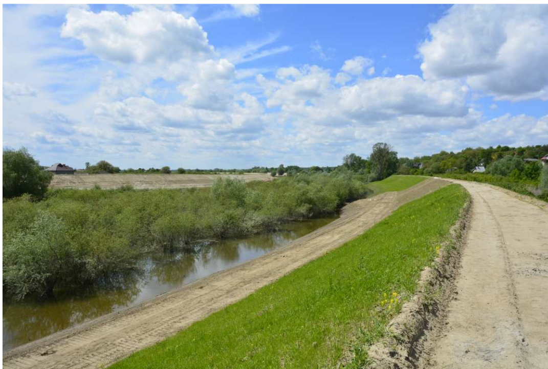
Fig. 43. Growth of grasses sown on the slope of the flood embankment – left bank of Koprzywianka river upstream of the bridge on the road Sandomierz-Zawisielcze, status in the third decade of May 2021 (upstream view).
