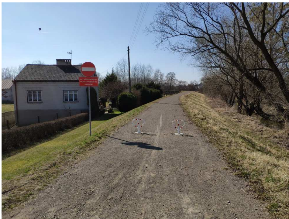
Fig. 56. Site condition in the last quarter of the works implementation period on Task 4 – right bank of Koprzywianka river upstream of the bridge on the road no. 758 in Koprzywnica, status in the third decade of March 2022 (upstream view).
