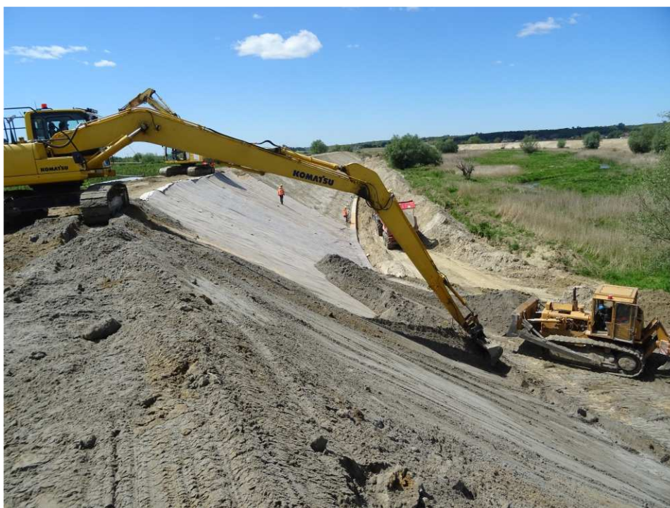
Fig. 38. Placement of bentomat on the slope of the flood embankment – right bank of Koprzywianka river downstream of the bridge on the road Andruszkowice-Koćmierzów, status in the third decade of May 2020 (upstream view).
