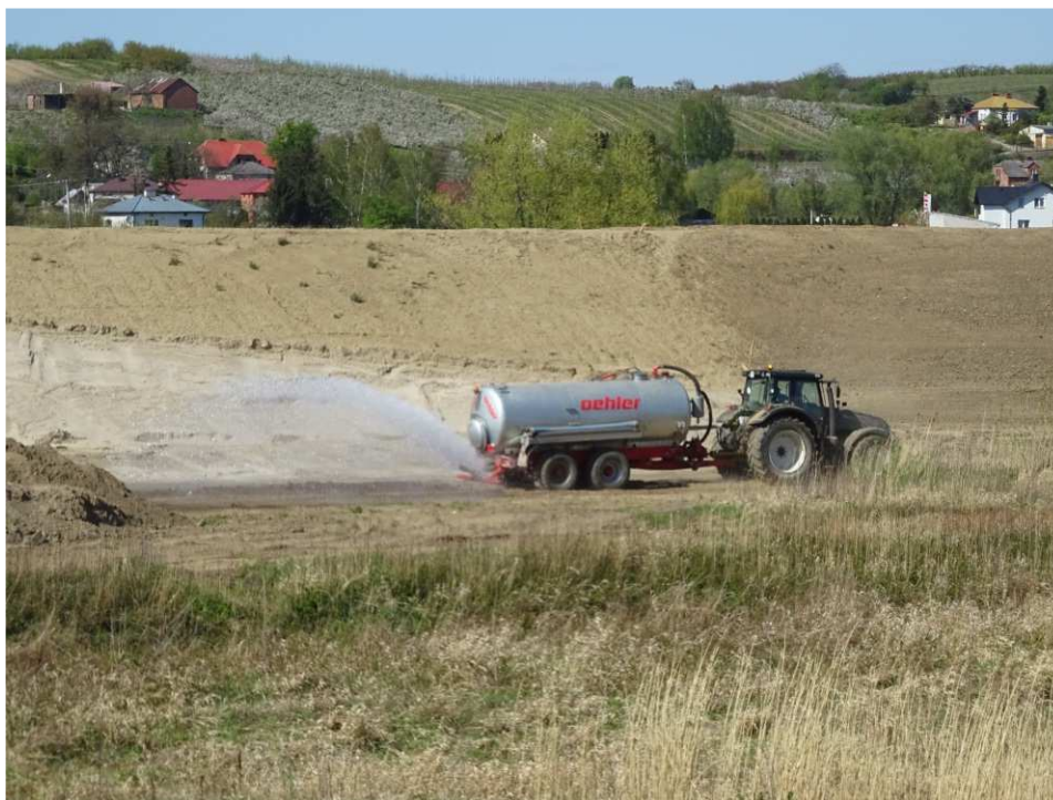
Fig. 19. Sprinkling technological roads in order to reduce dusting – left bank of Koprzywianka river downstream of the bridge on the road Andruszkowice-Koćmierzów, status in the third decade of April 2020 (downstream view).
