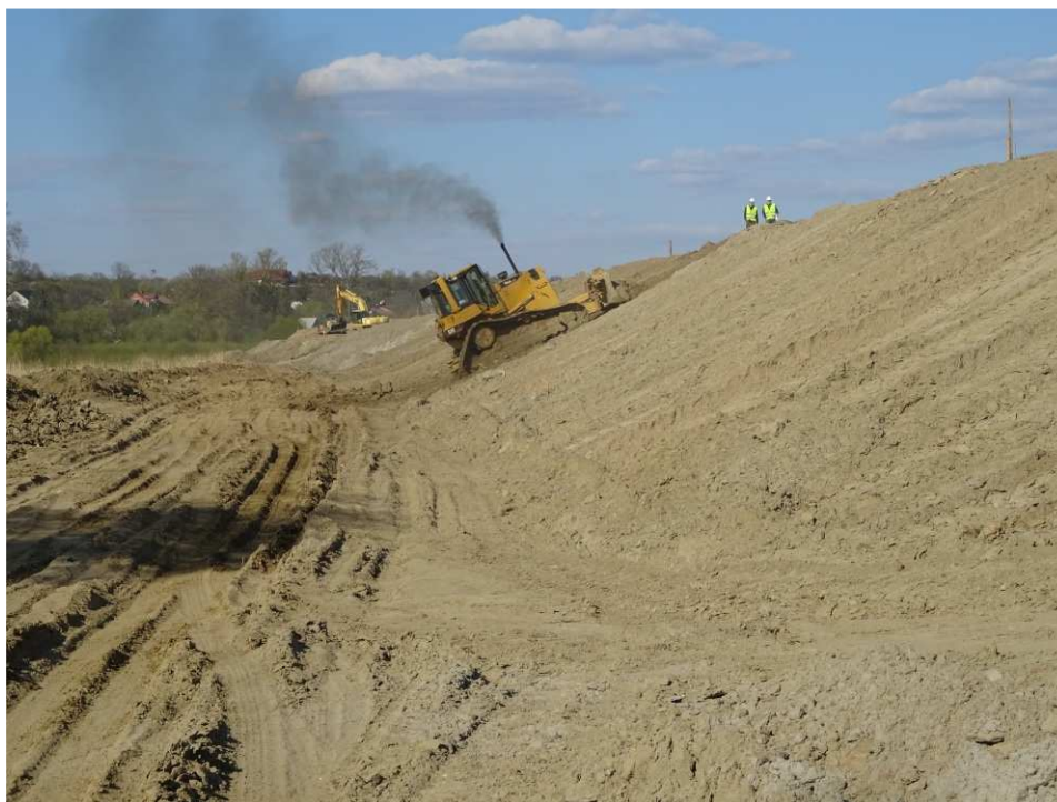
Fig. 33. Shaping the slopes of the flood embankment – right bank of Koprzywianka river downstream of the bridge on the road Andruszkowice-Koćmierzów, status in the second decade of April 2020 (downstream view).
