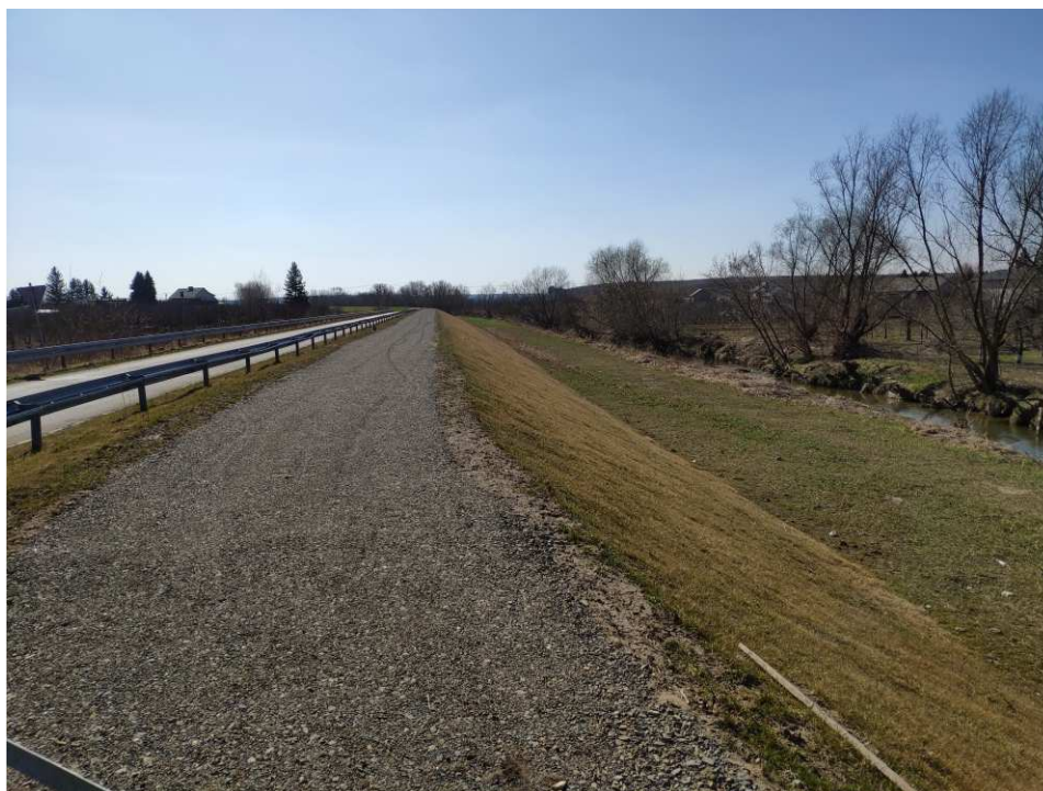
Fig. 54. Site condition in the last quarter of the works implementation period on Task 4 – right bank of Koprzywianka river upstream of the bridge on the road Sośniczany-Skotniki, status in the third decade of March 2022 (upstream view).
