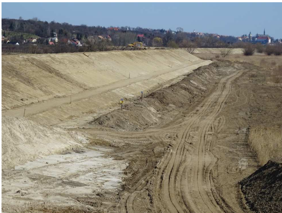
Fig. 23. Protection of top-soil piles – left bank of Koprzywianka river downstream of the bridge on the road Andruszkowice-Koćmierzów, status in the third decade of March 2020 (downstream view).
