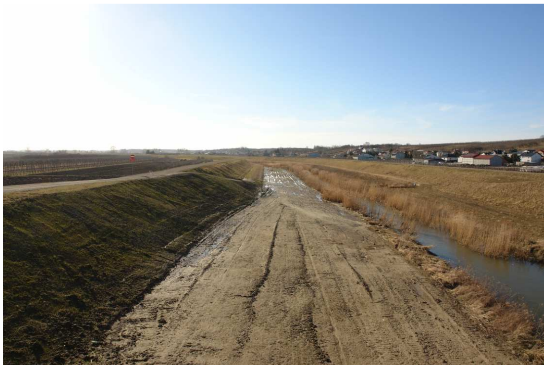
Fig. 51. Site condition in the last quarter of the works implementation period on Task 4 – banks of Koprzywianka river upstream of the bridge on the road Złota-Zawierzbie, status in the third decade of February 2022 (upstream view).
