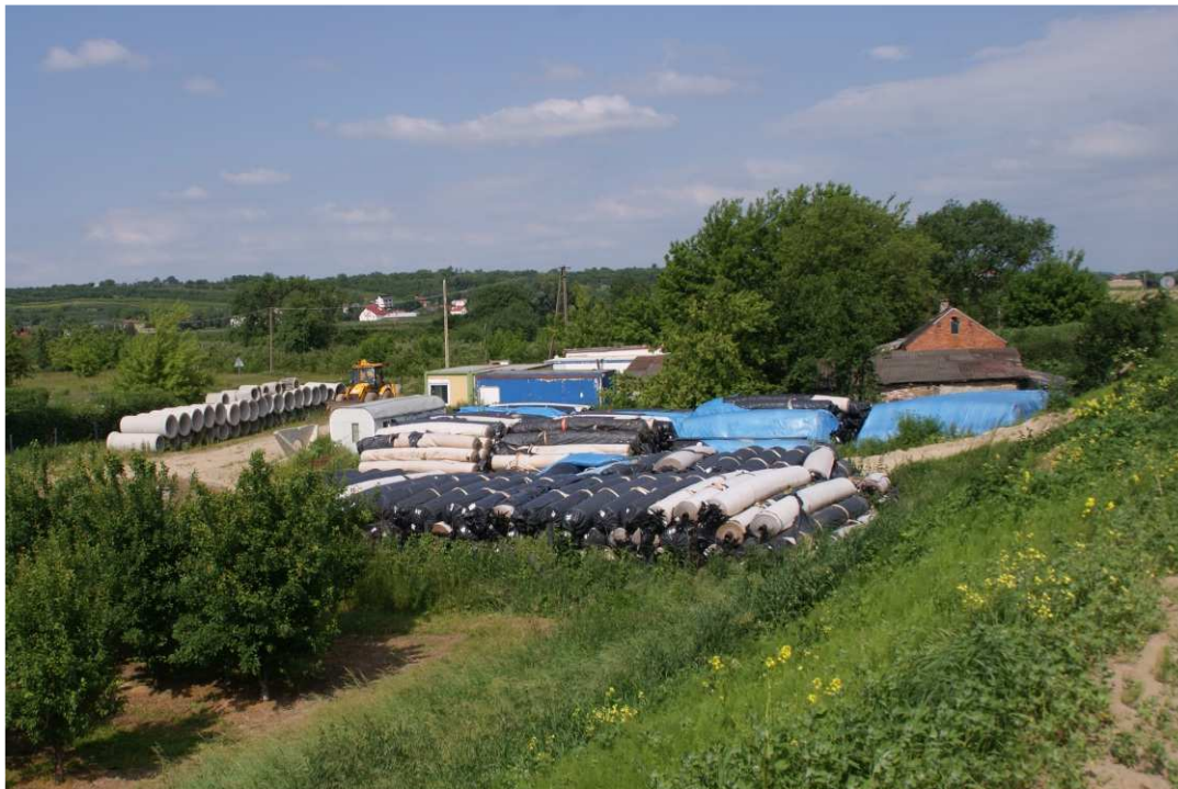
Fig. 9. Site facilities in the area beyond the left Koprzywianka embankment – left bank of Koprzywianka river upstream of the bridge on the road Andruszkowice-Koćmierzów, status in the second decade of June 2020 (downstream view).
