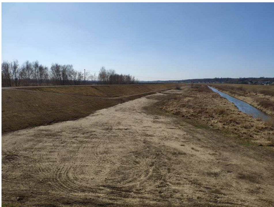
Fig. 50. Site condition in the last quarter of the works implementation period on Task 4 – banks of Koprzywianka river upstream of the bridge on the road Andruszkowice-Koćmierzów, status in the third decade of March 2022 (upstream view).
