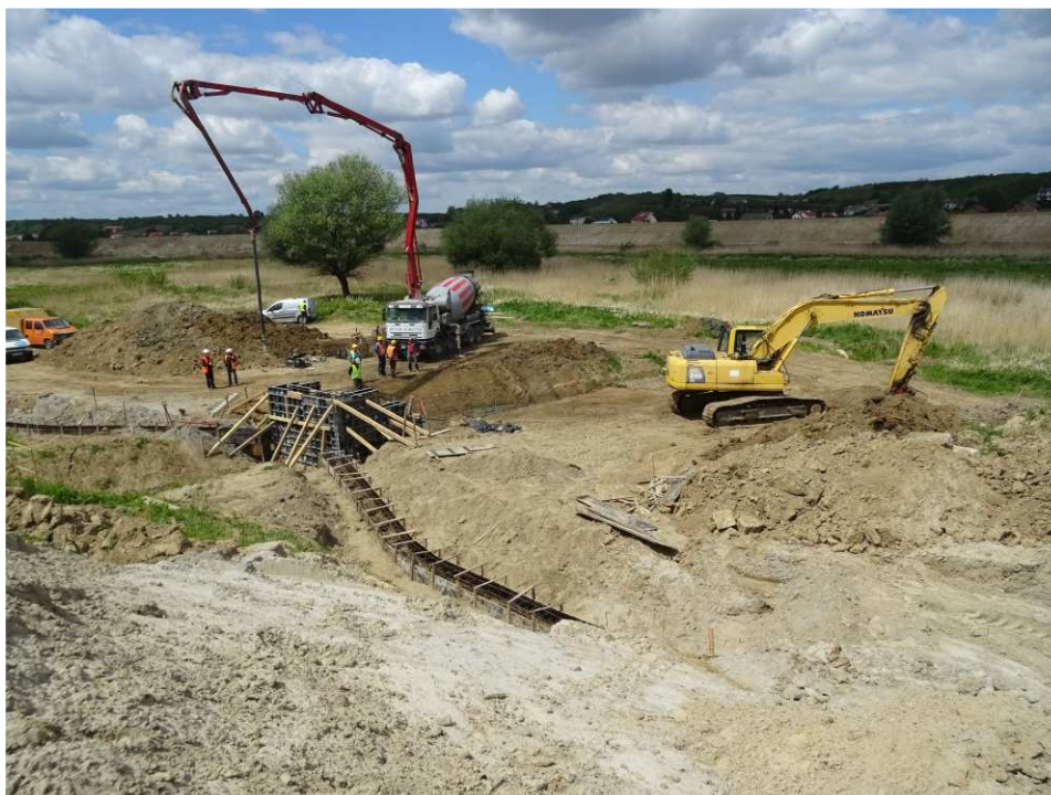
Fig. 29. Reconstruction of the embankment culvert – right bank of Koprzywianka river downstream of the bridge on the road Andruszkowice-Koćmierzów, status in the second decade of May 2020 (upstream view).
