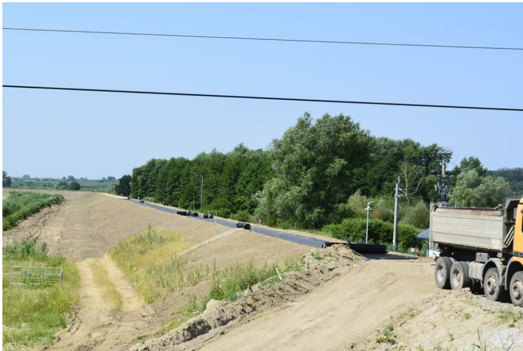
Fig. 41. Construction of a road on the crown of the flood embankment – left bank of Koprzywianka river upstream of the bridge on the road Szewce-Skotniki, status in the second decade of June 2021 (upstream view).
