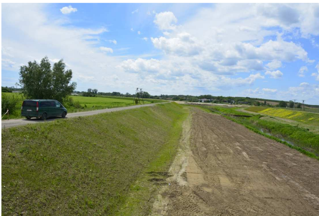
Fig. 46. Reclamation of the area between the Koprzywianka embankments – banks of Koprzywianka river upstream of the bridge on the road Samborzec-Zajeziorko, status in the third decade of May 2021 (upstream view).
