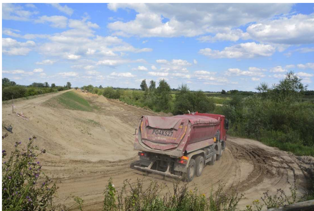
Fig. 32. Transport of earth masses for the construction of a flood embankment – left bank of Koprzywianka river downstream of the bridge on the road Sośniczany-Skotniki, status in the third decade of July 2020 (downstream view).
