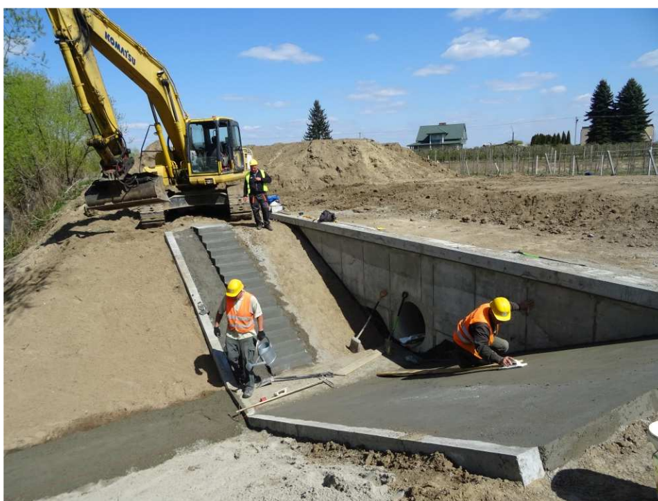
Fig. 30. Reconstruction of the embankment culvert – right bank of Koprzywianka river upstream of the bridge on the road Sońniczany-Skotniki, status in the second decade of April 2020 (downstream view).
