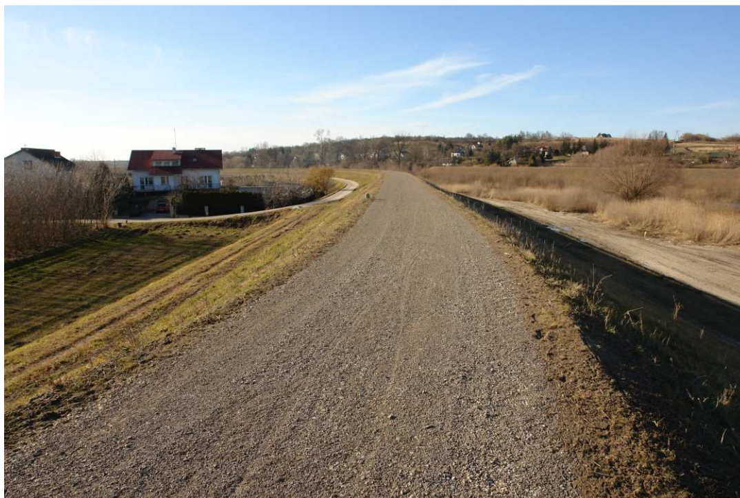
Fig. 49. Site condition in the last quarter of the works implementation period on Task 4 – banks of Koprzywianka river upstream of the bridge on the road Sandomierz-Zawisłe, status in the third decade of February 2022 (upstream view).
