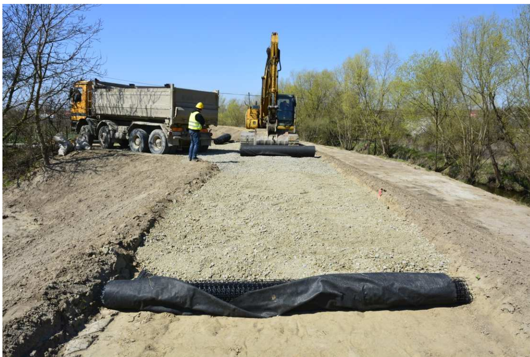
Fig. 42. Construction of a road on the crown of the flood embankment – right bank of Koprzywianka river upstream of the footbridge in Koprzywnica, status in the third decade of April 2021 (upstream view).
