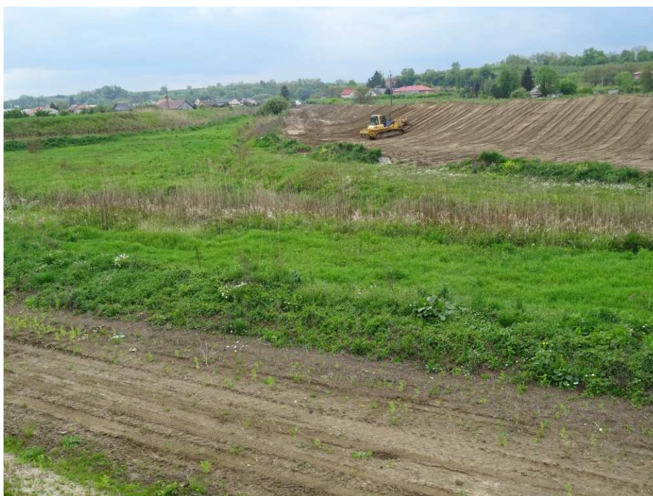
Fig. 34. Shaping the slopes of the flood embankment – left bank of Koprzywianka river downstream of the mouth of Polanówka stream, status in the second decade of May 2020 (upstream view).
