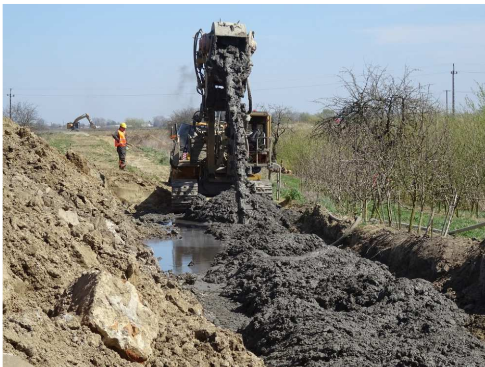
Fig. 26. Construction of a cement-bentonite barrier – left bank of Polanówka stream downstream of the bridge on the road Kraków-Sandomierz, status in the second decade of April 2020 (downstream view).
