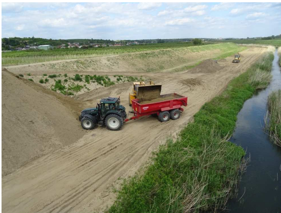
Fig. 31. Transport of earth masses for the construction of a flood embankment – left bank of Koprzywianka river downstream of the bridge on the road Złota-Zawierzbie, status in the second decade of May 2020 (downstream view).
