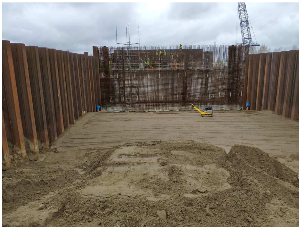
Fig. 43. Construction of a flood gate on the port channel in Sandomierz, status in the third decade of April 2022 (view towards the south-east).
