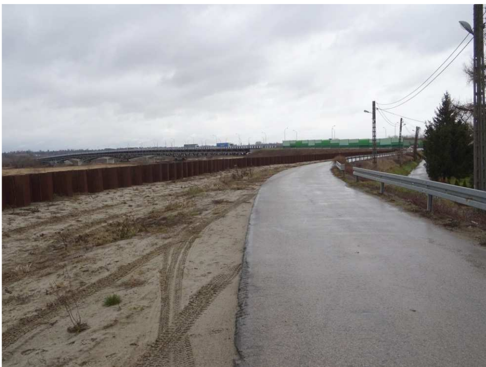
Fig. 2. Site condition in the first quarter of the works implementation period on Task 3 – band embankment within the artery of Mostowa Street, status in the second decade of February 2020 (view towards the north-east).
