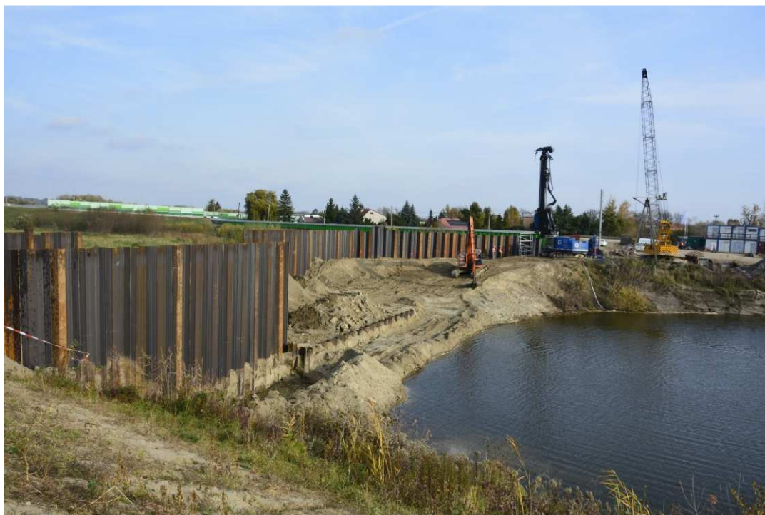
Fig. 45. Works in a bed of the port channel carried out under the cover of sheet piling – flood gate on the port channel in Sandomierz, status in the third decade of October 2021 (view towards the south-east).
