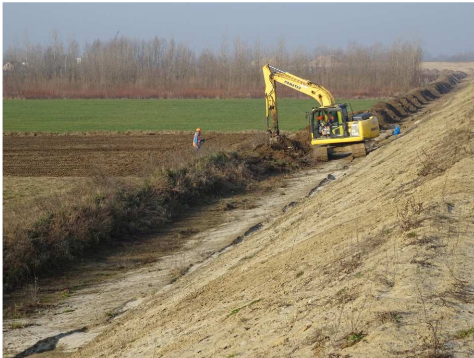
Fig. 21. Protection of top-soil piles – band embankment between Zarzekowice Street and the right embankment of Vistula, status in the second decade of March 2020 (view towards the south-west).
