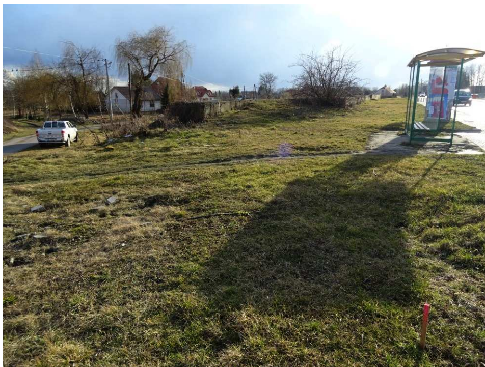
Fig. 4. Site condition in the first quarter of the works implementation period on Task 3 – band embankment within the artery of Portowa Street, status in the second decade of February 2020 (view towards the south-west).
