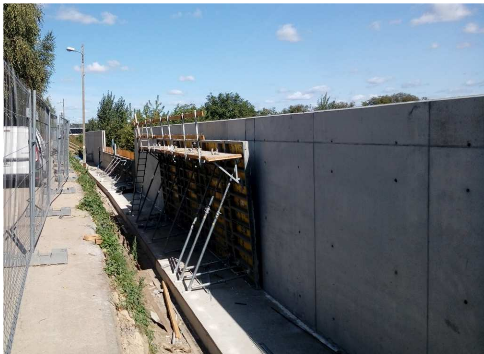
Fig. 27. Construction of a reinforced concrete retaining wall – band embankment within the artery of Mostowa Street, status in the second decade of September 2020 (view towards the north-east).
