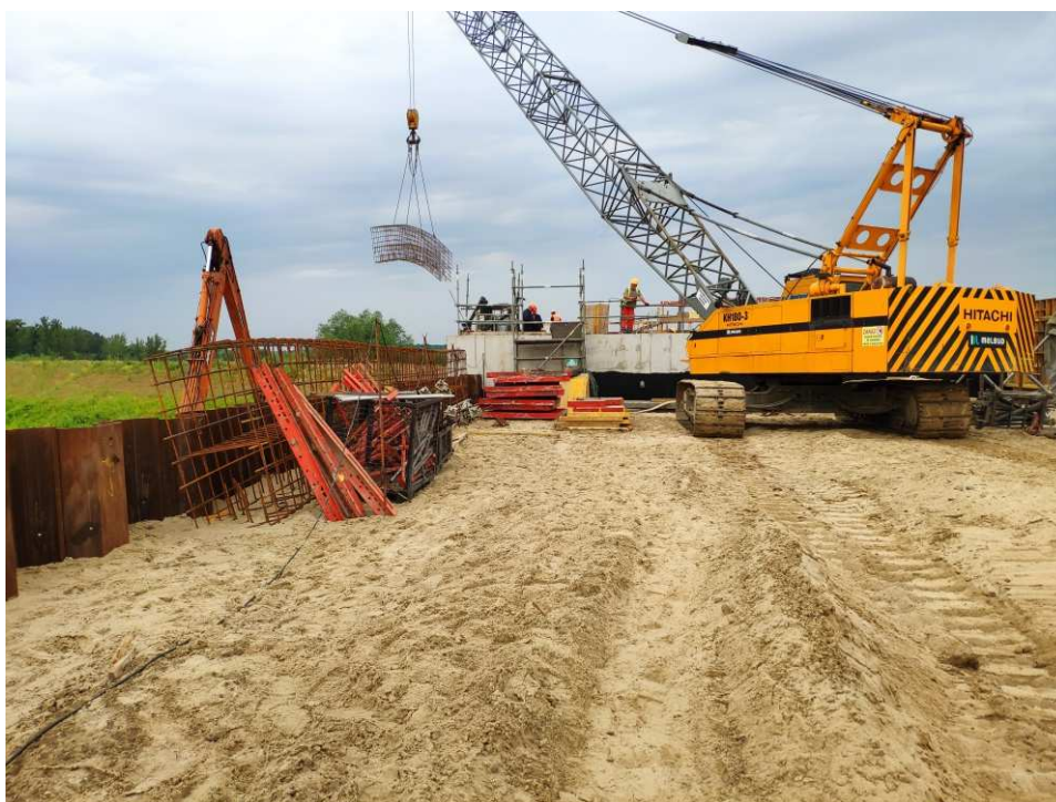
Fig. 44. Construction of a flood gate on the port channel in Sandomierz, status in the first decade of July 2022 (view towards the north-west).
