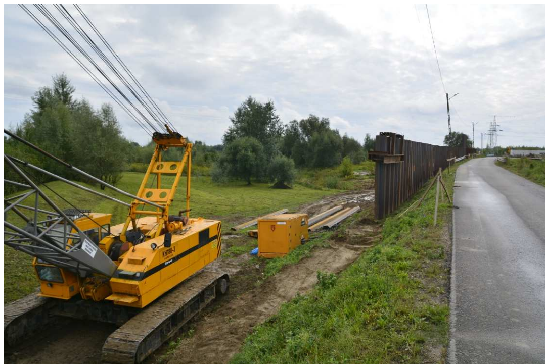
Fig. 26. Construction of a retaining wall made of steel sheet piles – band embankment within the artery of Zarzekowice Street, status in the first decade of September 2020 (view towards the south-west).
