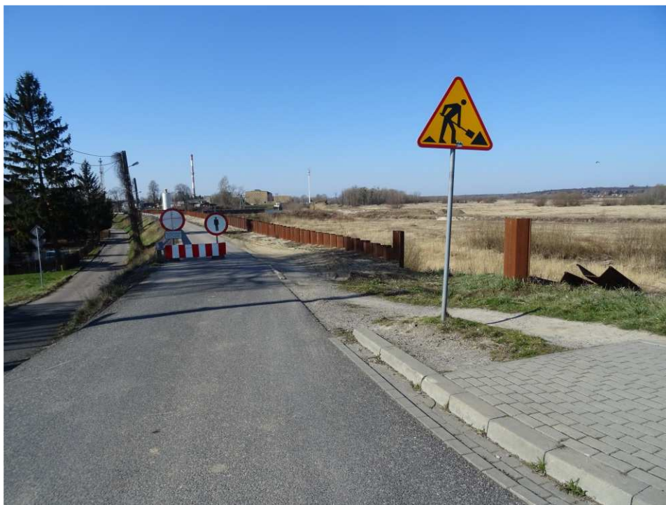
Fig. 15. Marking of public road near the exit from the construction site – band embankment within the artery of Mostowa Street, status in the third decade of March 2020 (view towards the south-west).
