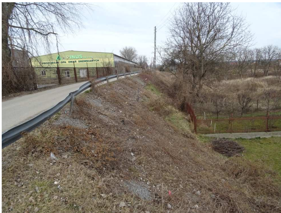
Fig. 3. Site condition in the first quarter of the works implementation period on Task 3 – band embankment within the artery of Mostowa Street, status in the second decade of February 2020 (view towards the north-east).
