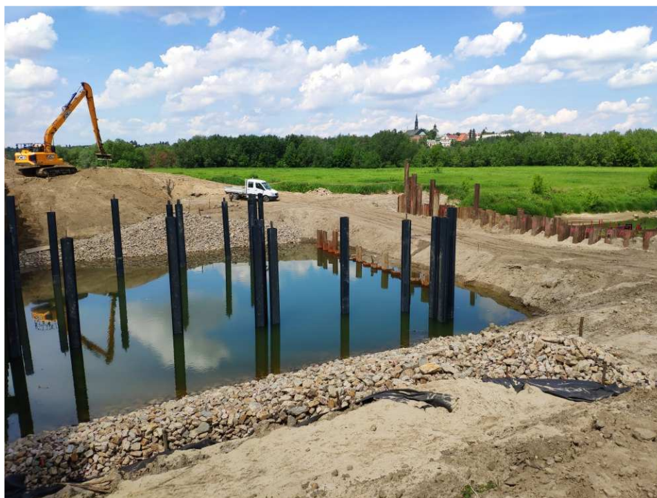
Fig. 46. Works in a bed of the port channel carried out under the cover of sheet piling – flood gate on the port channel in Sandomierz, status in the third decade of May 2022 (view towards the north-west).
