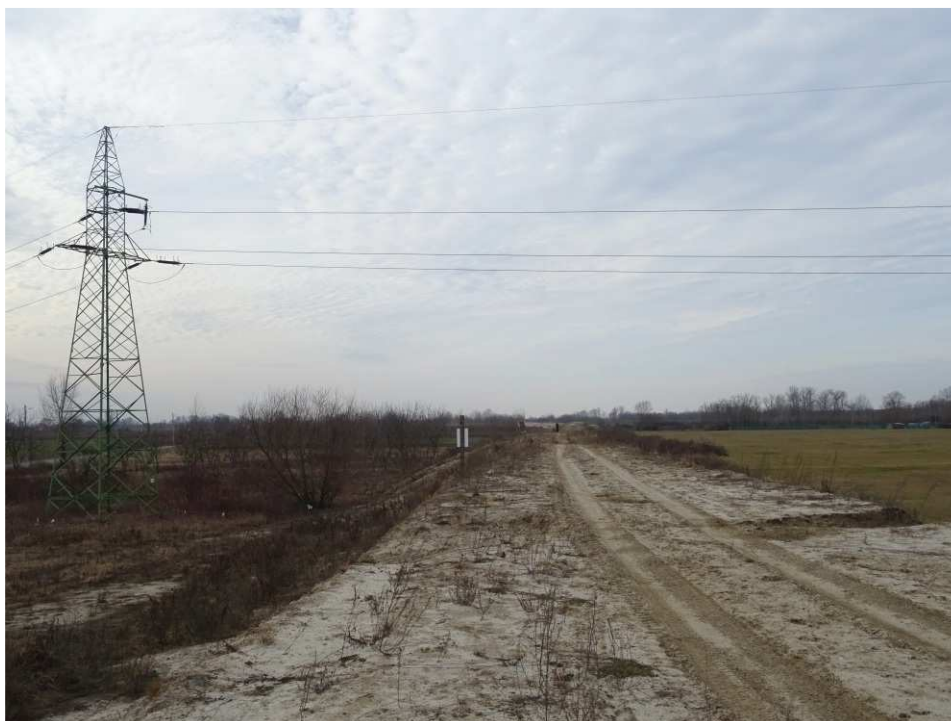
Fig. 6. Site condition in the first quarter of the works implementation period on Task 3 – band embankment between Zarzekowice Street and the right embankment of Vistula, status in the second decade of February 2020 (view towards the south-west).
