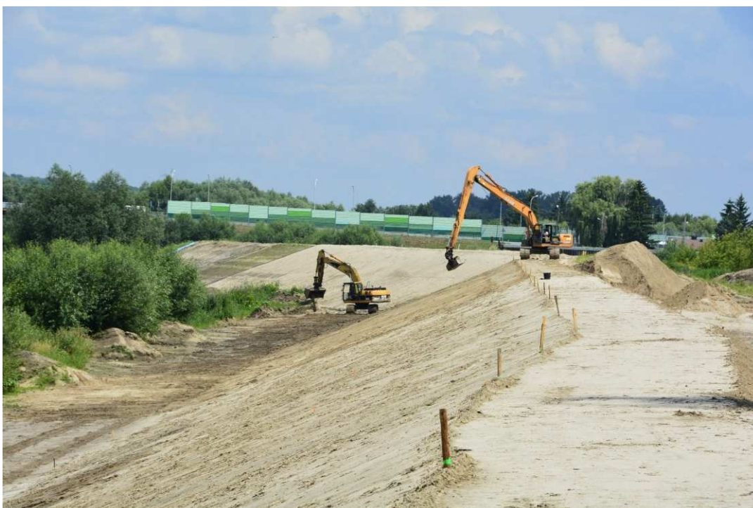
Fig. 36. Covering slopes of the flood embankment with a top-soil layer – right-bank Vistula embankment along the bank of the port channel, status in the first decade of July 2021 (view towards the north-east).
