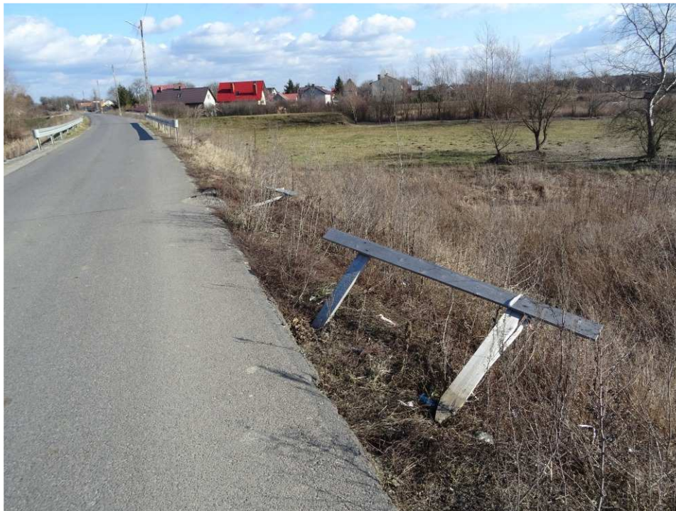
Fig. 5. Site condition in the first quarter of the works implementation period on Task 3 – band embankment within the artery of Zarzekowice Street, status in the second decade of February 2020 (view towards the north-east).
