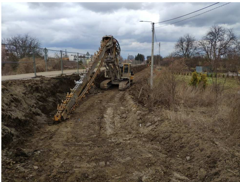
Fig. 24. Construction of a cement-bentonite barrier – band embankment within the artery of Zarzekowice Street, status in the first decade of April 2022 (view towards the north-east).
