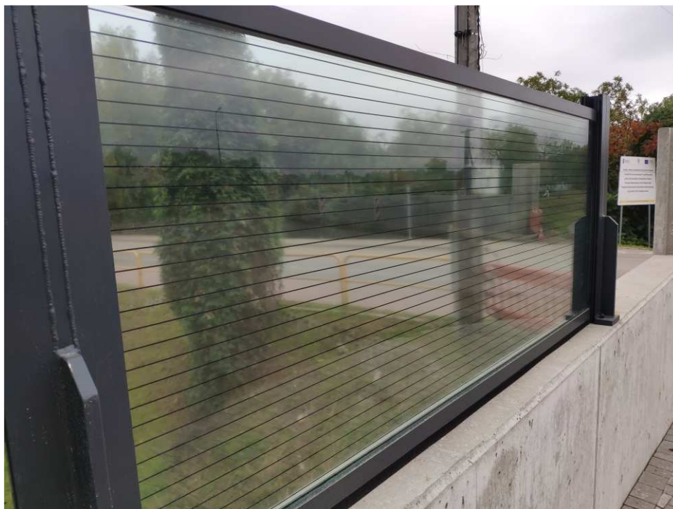
Fig. 29. Protection against birds crashing against the glass – band embankment within the artery of Mostowa Street, status in the third decade of September 2022 (view towards the south-west).
