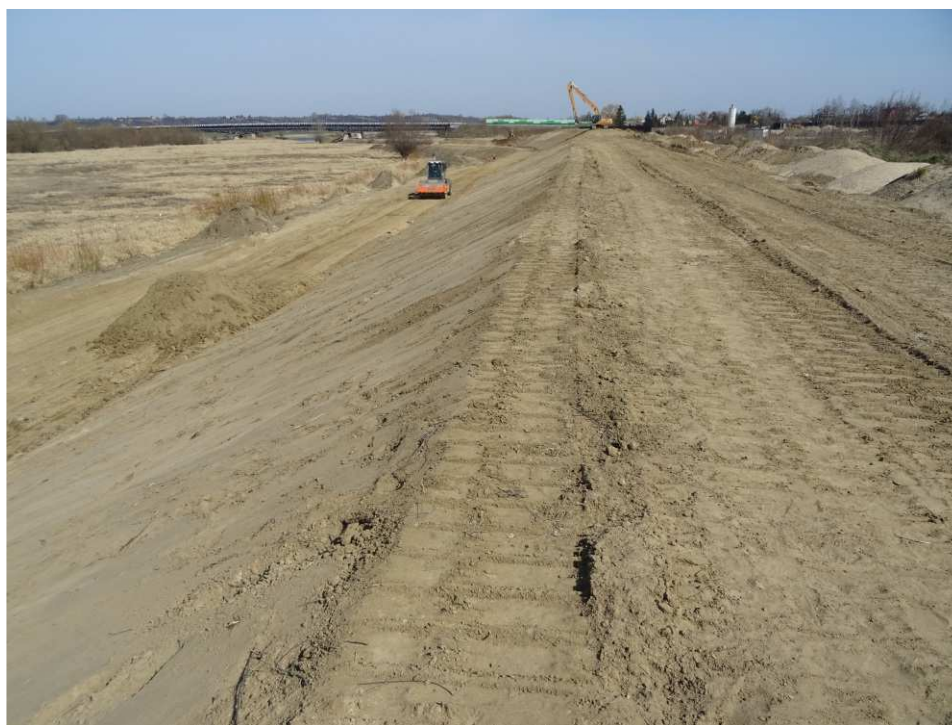
Fig. 32. Shaping the slopes of the flood embankment – right-bank Vistula embankment along the bank of the port channel, status in the third decade of March 2020 (view towards the north-east).
