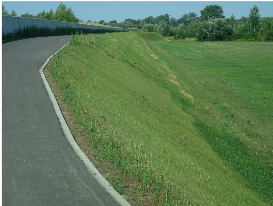
Fig. 39. Growth of grasses sown on the slope of the flood embankment – band embankment between Zarzekowice Street and the right embankment of Vistula, status in the third decade of July 2022 (view towards the south-west).
