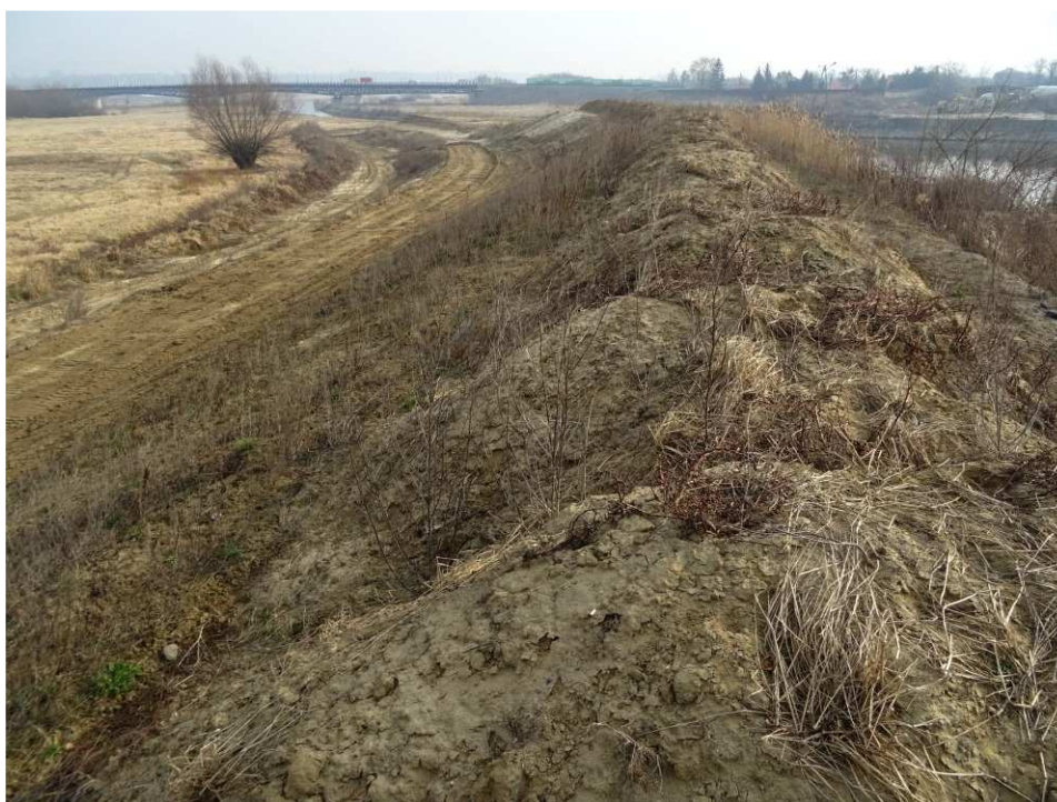
Fig. 8. Site condition in the first quarter of the works implementation period on Task 3 – right-bank Vistula embankment along the bank of the port channel, status in the second decade of March 2020 (view towards the north-east).
