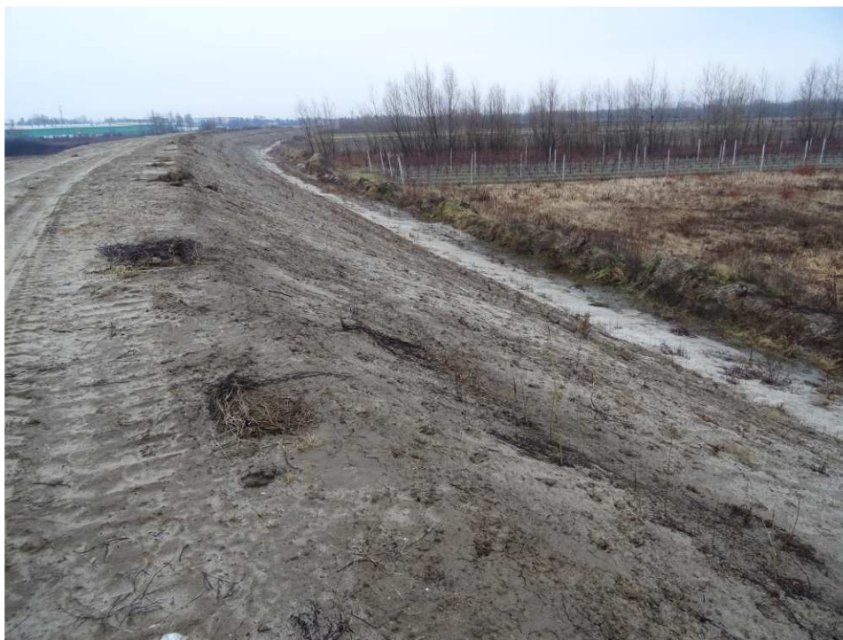
Fig. 7. Site condition in the first quarter of the works implementation period on Task 3 – band embankment between Zarzekowice Street and the right embankment of Vistula, status in the second decade of February 2020 (view towards the north-east).
