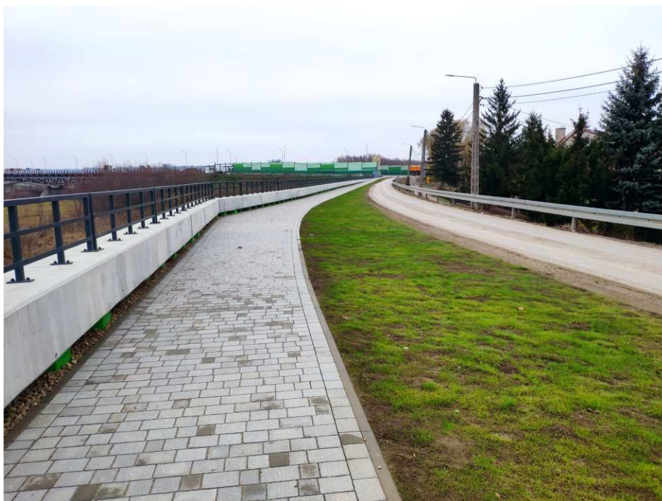
Fig. 50. Site condition in the last quarter of the works implementation period on Task 3 – band embankment within the artery of Mostowa Street, status in the third decade of November 2022 (view towards the north-east).
