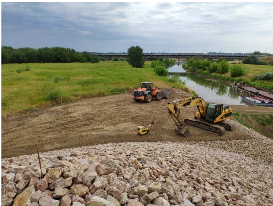
Fig. 48. No impact on Natura 2000 site beyond the boundaries of the works site – flood gate on the port channel in Sandomierz, status in the first decade of July 2022 (view towards the north-east).
