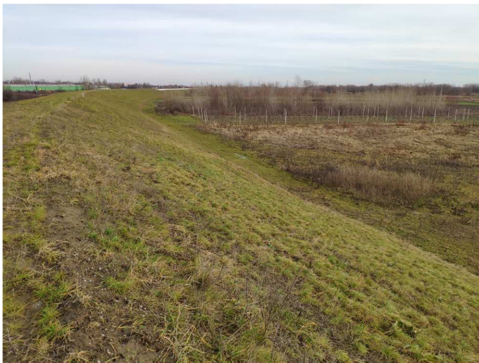
Fig. 55. Site condition in the last quarter of the works implementation period on Task 3 – band embankment between Zarzekowice Street and the right embankment of Vistula, status in the third decade of December 2022 (view towards the north-east).
