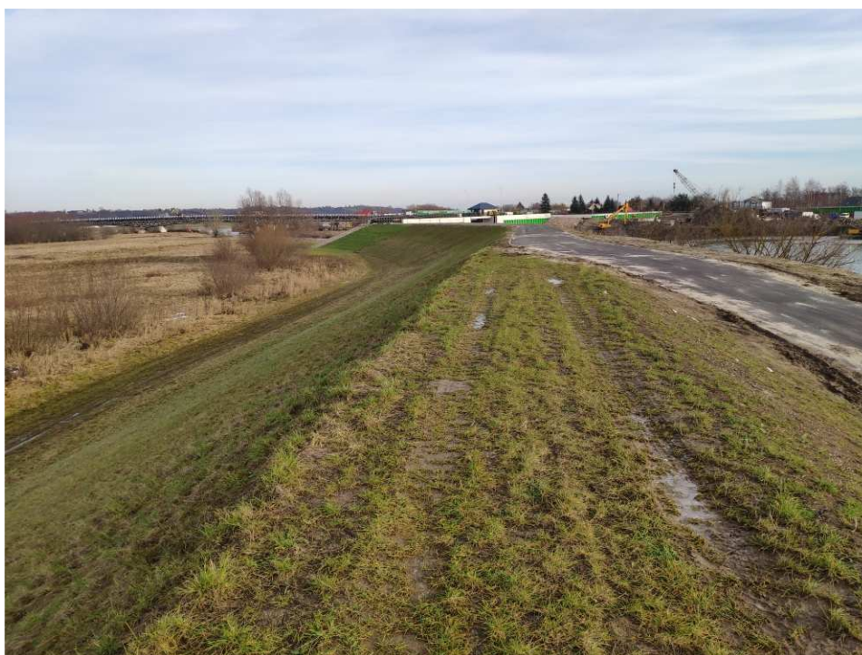
Fig. 56. Site condition in the last quarter of the works implementation period on Task 3 – right-bank Vistula embankment along the bank of the port channel, status in the third decade of December 2022 (view towards the north-east).
