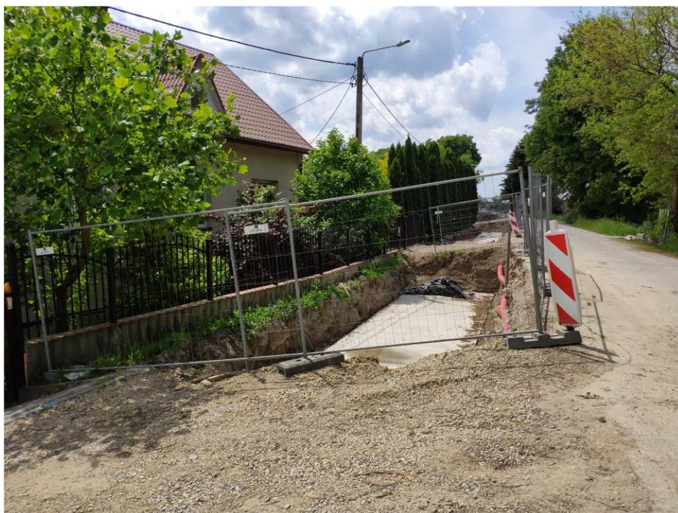
Fig. 14. Protection of hazardous sites – band embankment within the artery of Zarzekowice Street, status in the third decade of May 2022 (view towards the south-west).
