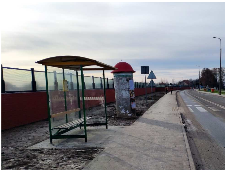
Fig. 52. Site condition in the last quarter of the works implementation period on Task 3 – band embankment within the artery of Portowa Street, status in the third decade of December 2022 (view towards the south-west).
