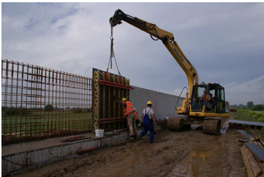
Fig. 28. Construction of a reinforced concrete retaining wall – band embankment between Zarzekowice Street and the right embankment of Vistula, status in the third decade of June 2020 (view towards the south-west).
