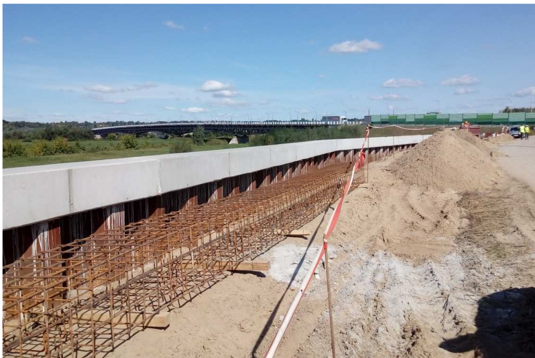
Fig. 25. Construction of a retaining wall made of steel sheet piles – band embankment within the artery of Mostowa Street, status in the second decade of September 2020 (view towards the north-east).
