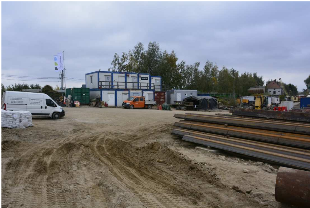
Fig. 9. Site facilities at the flood gate on the port channel in Sandomierz, status in the third decade of July 2020 (view towards the south-east).
