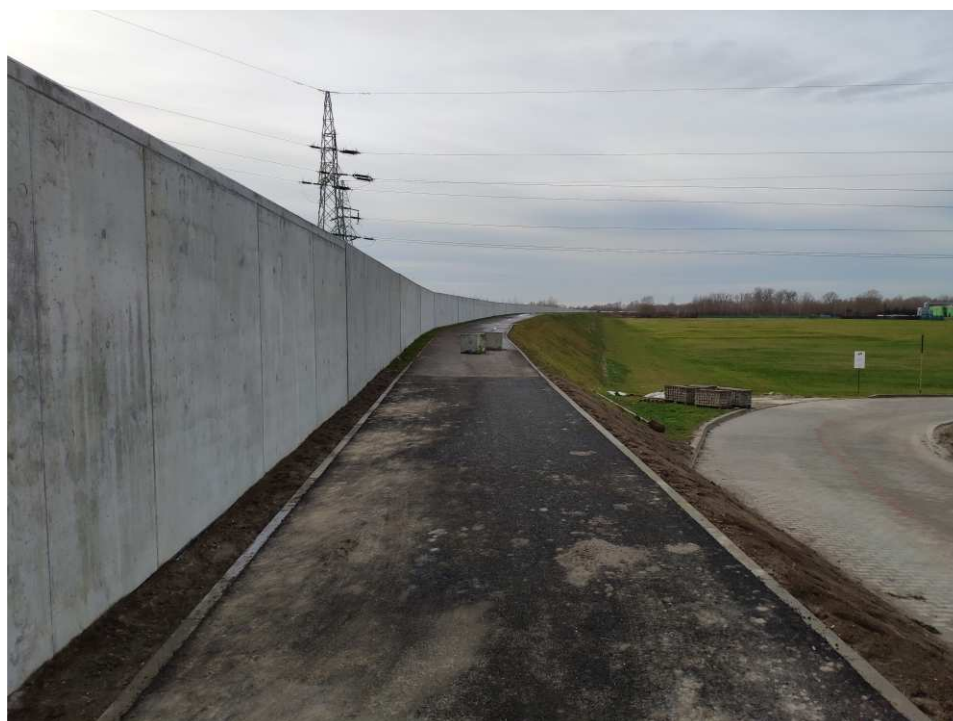
Fig. 54. Site condition in the last quarter of the works implementation period on Task 3 – band embankment between Zarzekowice Street and the right embankment of Vistula, status in the third decade of December 2022 (view towards the south-west).
