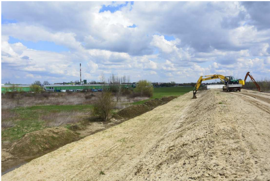
Fig. 33. Compaction of the body of the flood embankment – band embankment between Zarzekowice Street and the right embankment of Vistula, status in the third decade of April 2021 (view towards the north-east).
