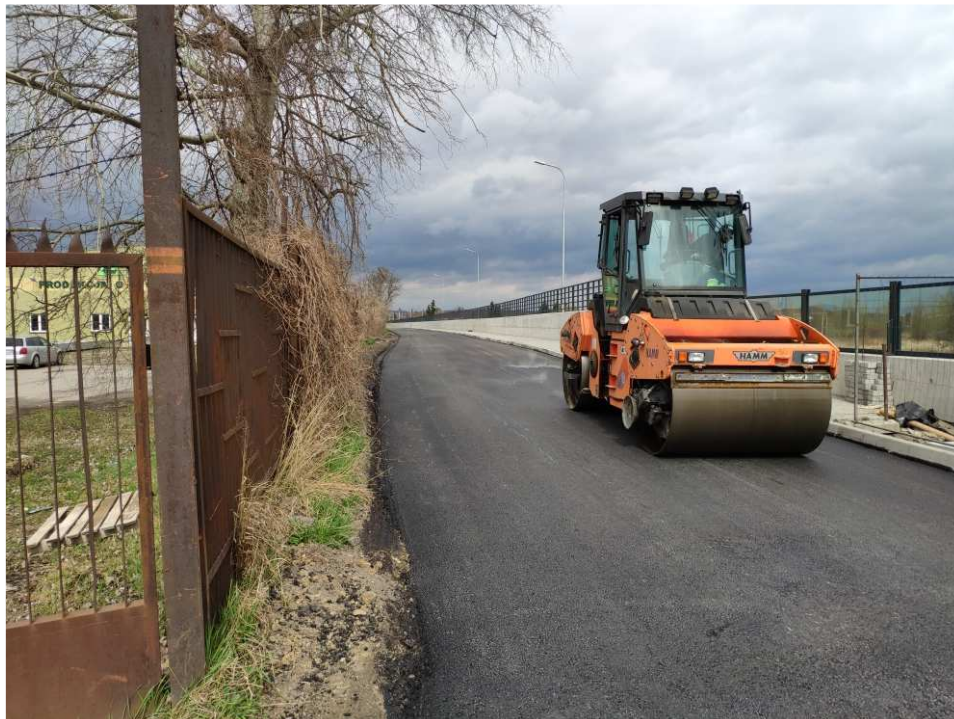
Fig. 37. Construction of a road on the band embankment – band embankment within the artery of Mostowa Street, status in the first decade of April 2022 (view towards the north-east).
