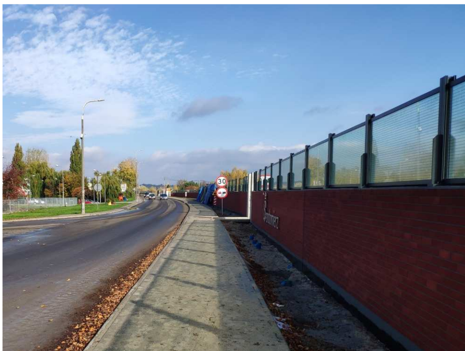
Fig. 30. Protection against birds crashing against the glass – band embankment within the artery of Zarzekowice Street, status in the third decade of October 2022 (view towards the north-east).
