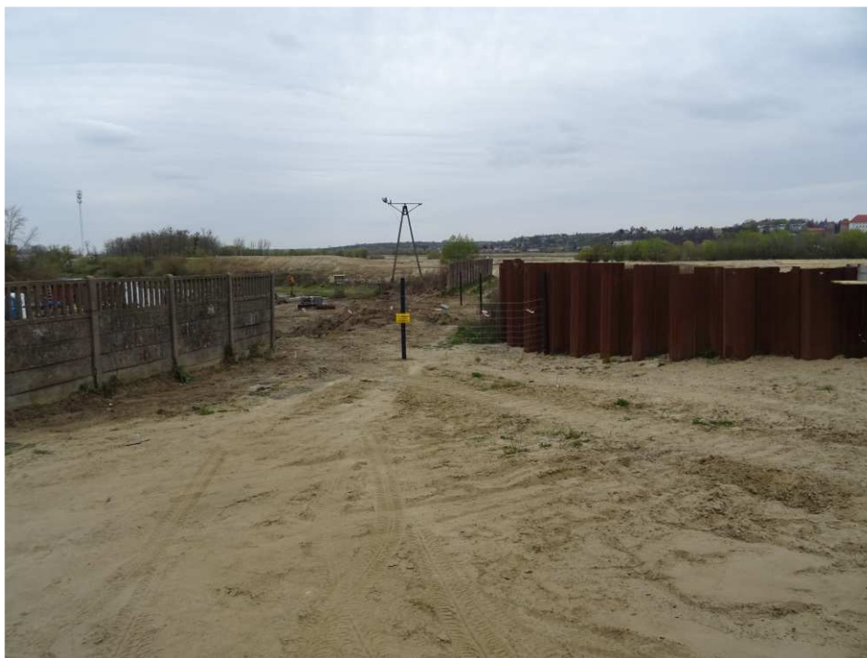
Fig. 11. Marking of the construction site – flood gate on the port channel in Sandomierz, status in the second decade of April 2020 (view towards the west).
