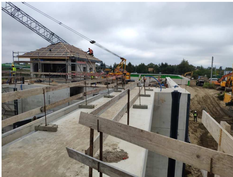
Fig. 13. Protection of hazardous sites – flood gate on the port channel in Sandomierz, status in the third decade of September 2022 (view towards the south-west).
