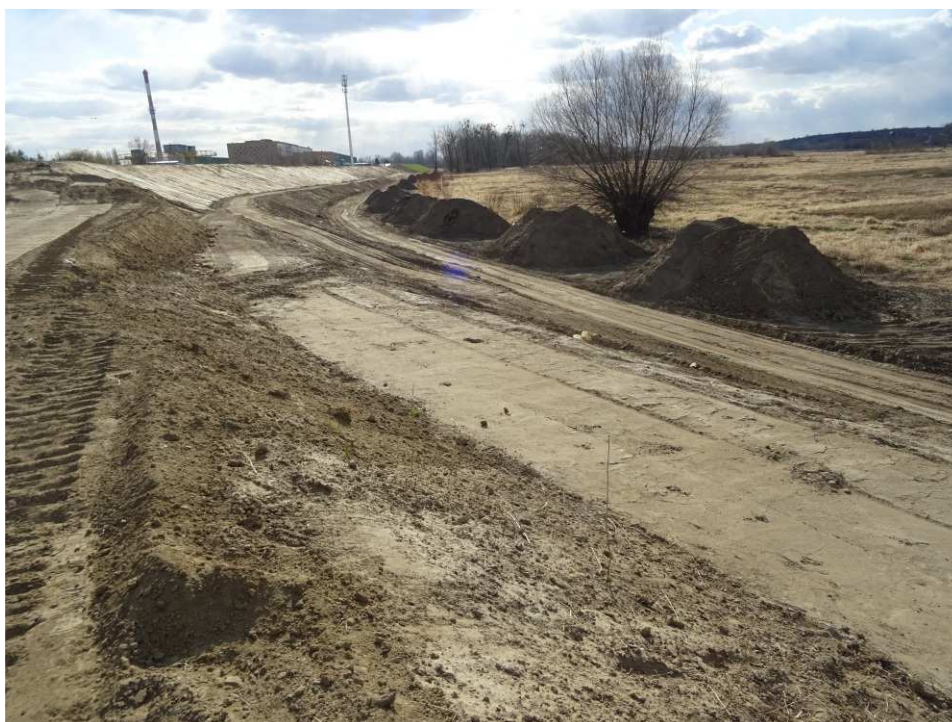
Fig. 22. Protection of top-soil piles – right-bank Vistula embankment along the bank of the port channel, status in the third decade of March 2020 (view towards the south-west).
