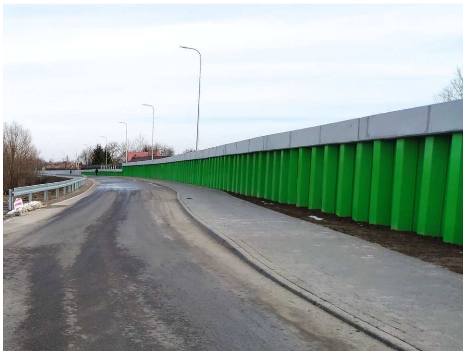
Fig. 53. Site condition in the last quarter of the works implementation period on Task 3 – band embankment within the artery of Zarzekowice Street, status in the third decade of December 2022 (view towards the north-east).
