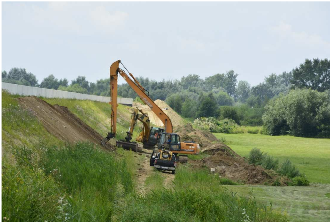
Fig. 35. Covering slopes of the flood embankment with a top-soil layer – band embankment between Zarzekowice Street and the right embankment of Vistula, status in the second decade of July 2021 (view towards the south-west).
