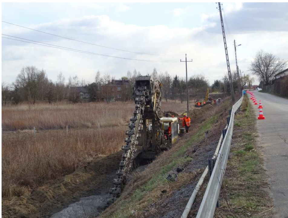
Fig. 23. Construction of a cement-bentonite barrier – band embankment within the artery of Mostowa Street, status in the third decade of March 2020 (view towards the south-west).
