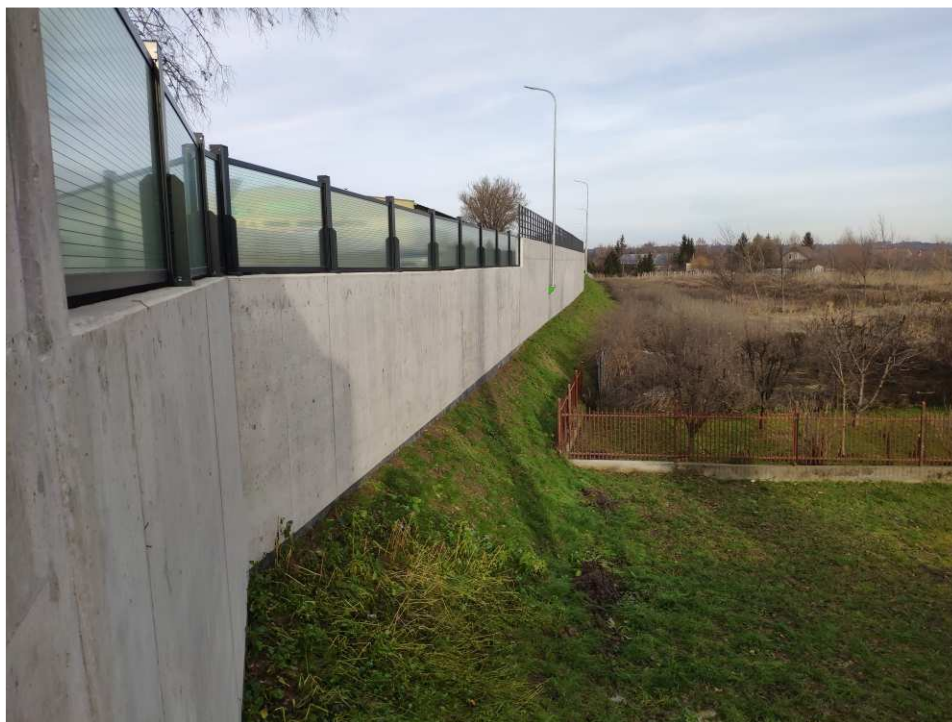
Fig. 51. Site condition in the last quarter of the works implementation period on Task 3 – band embankment within the artery of Mostowa Street, status in the third decade of December 2022 (view towards the north-east).
