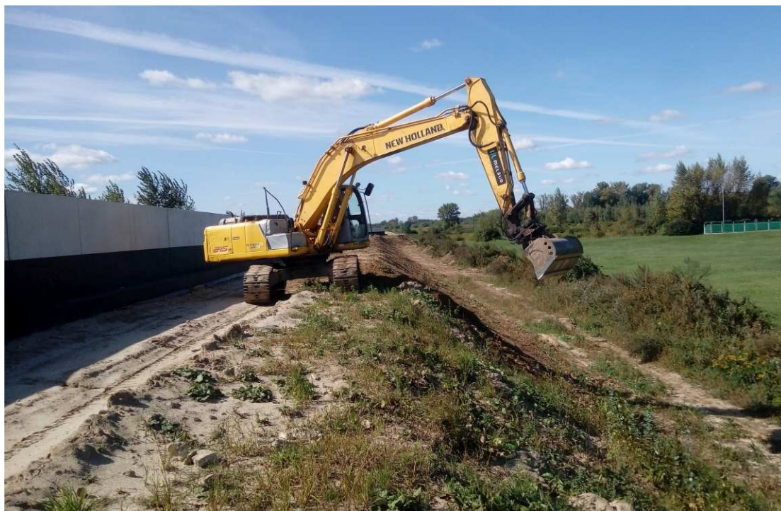
Fig. 31. Shaping the slopes of the flood embankment – band embankment between Zarzekowice Street and the right embankment of Vistula, status in the second decade of September 2020 (view towards the south-west).
