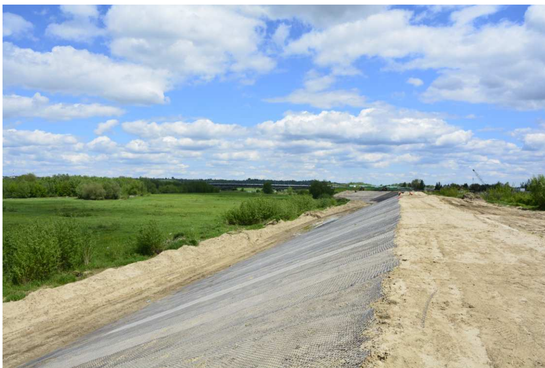
Fig. 34. Securing the slope of the flood embankment with a net against beavers – right-bank Vistula embankment along the bank of the port channel, status in the second decade of May 2021 (view towards the north-east).
