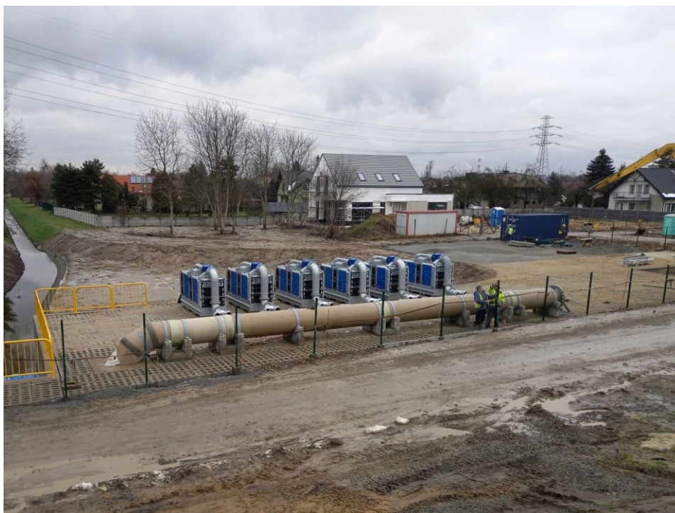
Fig. 51. Site condition in the last month of the works implementation period – construction area of a pumping station for mobile pumps and a site flood storage reservoir upstream of the embankment lock, status in the third decade of January 2023 (view towards the north).
