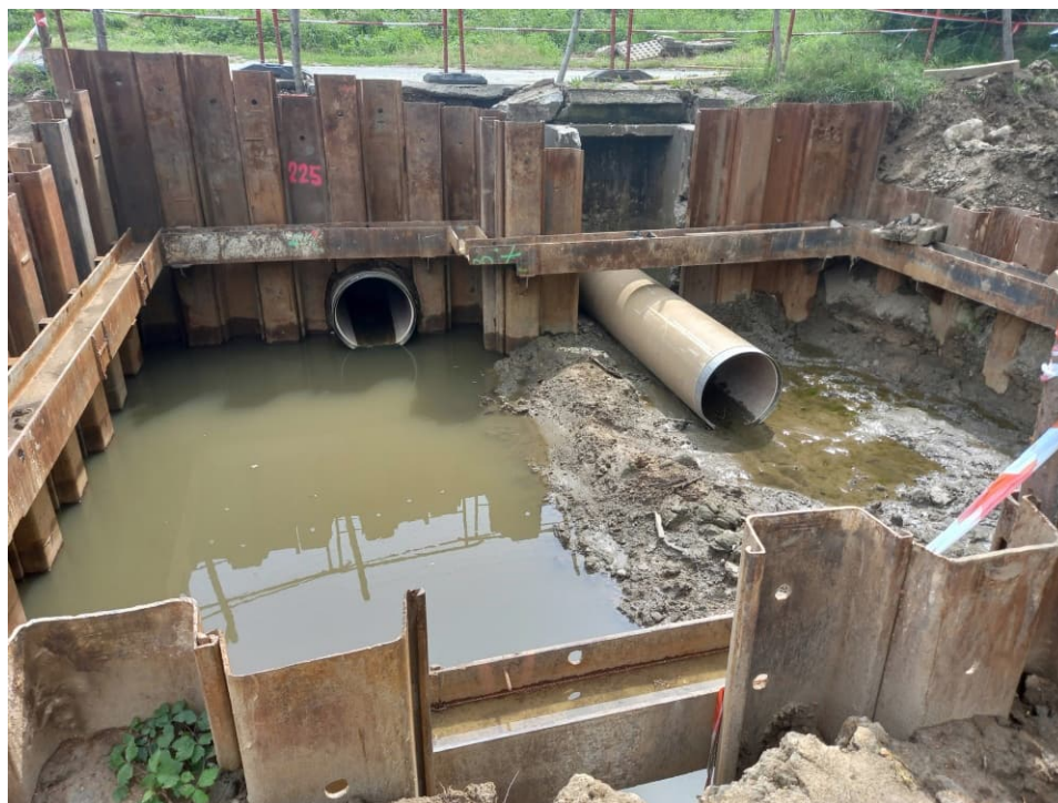
Fig. 33. Redeveloped gravity pipeline (right) and new pressure pipeline (left) on the construction area of embankment lock on the Ditch 2a, status in the third decade of July 2022 (view towards the south).
