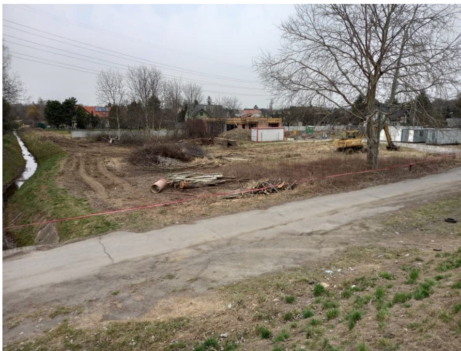
Fig. 3. Site condition in the first month of the works implementation period – construction area of a pumping station for mobile pumps and a site flood storage reservoir upstream of the embankment lock status in the third decade of March 2022 (view towards the north).
