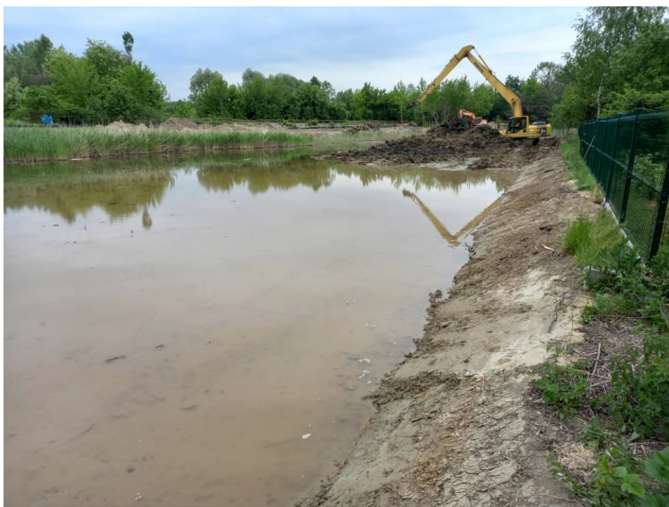
Fig. 46. Earthworks on the southern bank of the redeveloped reservoir on the Ditch 2, status in the third decade of May 2022 (view towards the east).
