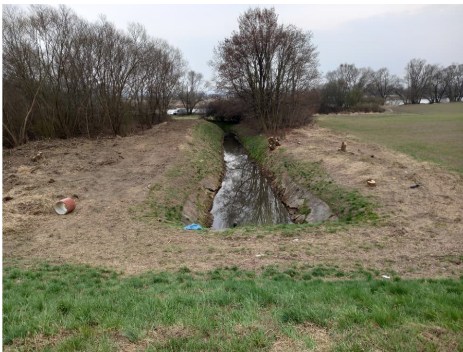
Fig. 1. Site condition in the first month of the works implementation period – construction area of an embankment lock on the Ditch 2a on the embanked area of the Vistula River, status in the third decade of March 2022 (view towards the south).
