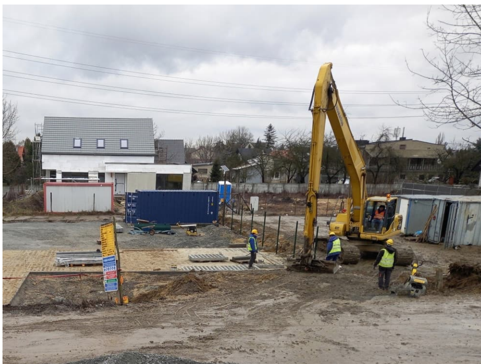
Fig. 40. Land reclamation in the vicinity of maneuvering yard and pumping station for mobile pumps on the Ditch 2a, status in the third decade of January 2023 (view towards the north).
