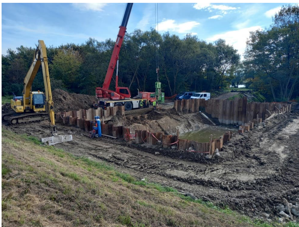
Fig. 32. Removal of sheet piling on the construction area of embankment lock on the Ditch 2a within the embanked area of the Vistula River, status in the third decade of September 2022 (view towards the south).
