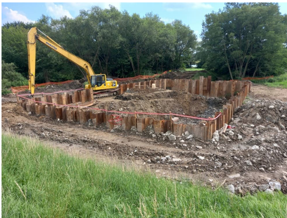
Fig. 31. Earthworks on the construction area of embankment lock on the Ditch 2a within the embanked area of the Vistula River, status in the third decade of July 2022 (view towards the south).
