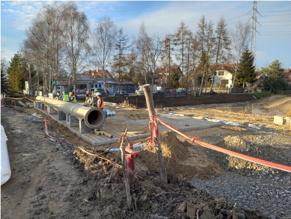
Fig. 38. Construction of a pumping station for mobile pumps on the Ditch 2a, status in the third decade of December 2022 (view towards the west).
