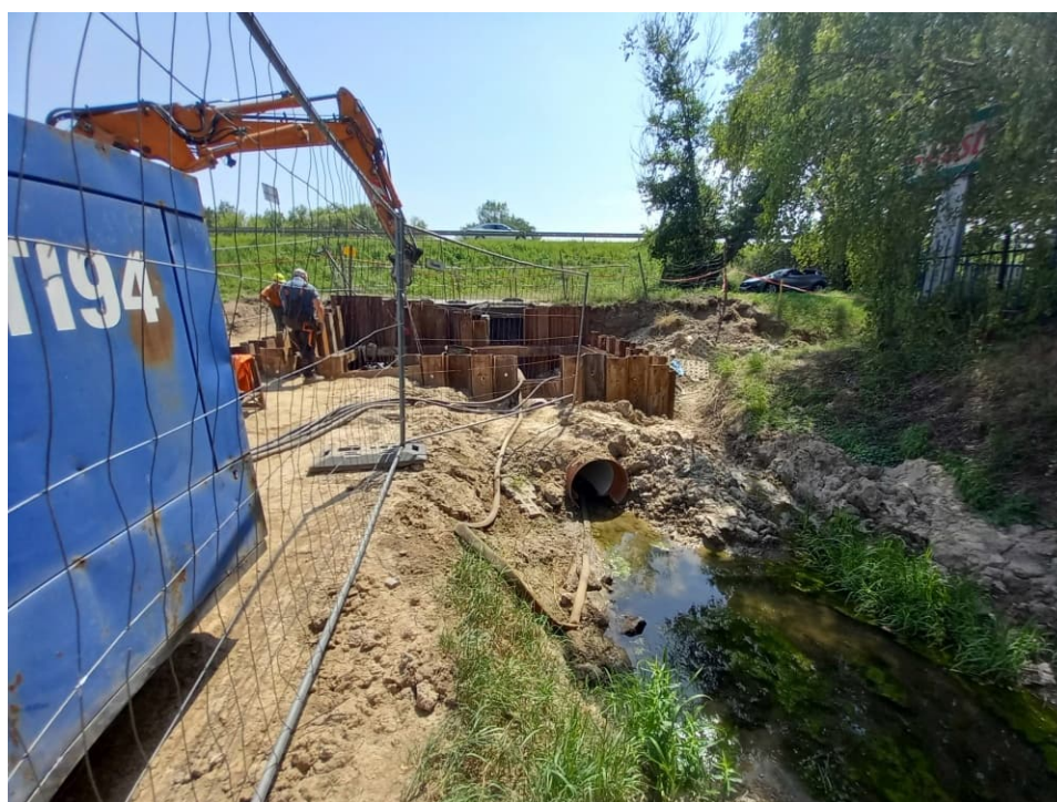
Fig. 34. Ensuring water flow in the Ditch 2a during works at the embankment lock, status in the third decade of June 2022 (view towards the south).
