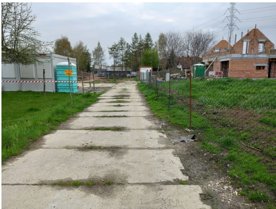
Fig. 17. Marking of the entrance to the construction site from the Klasztorna Street, status in the third decade of April 2022 (view towards the west).
