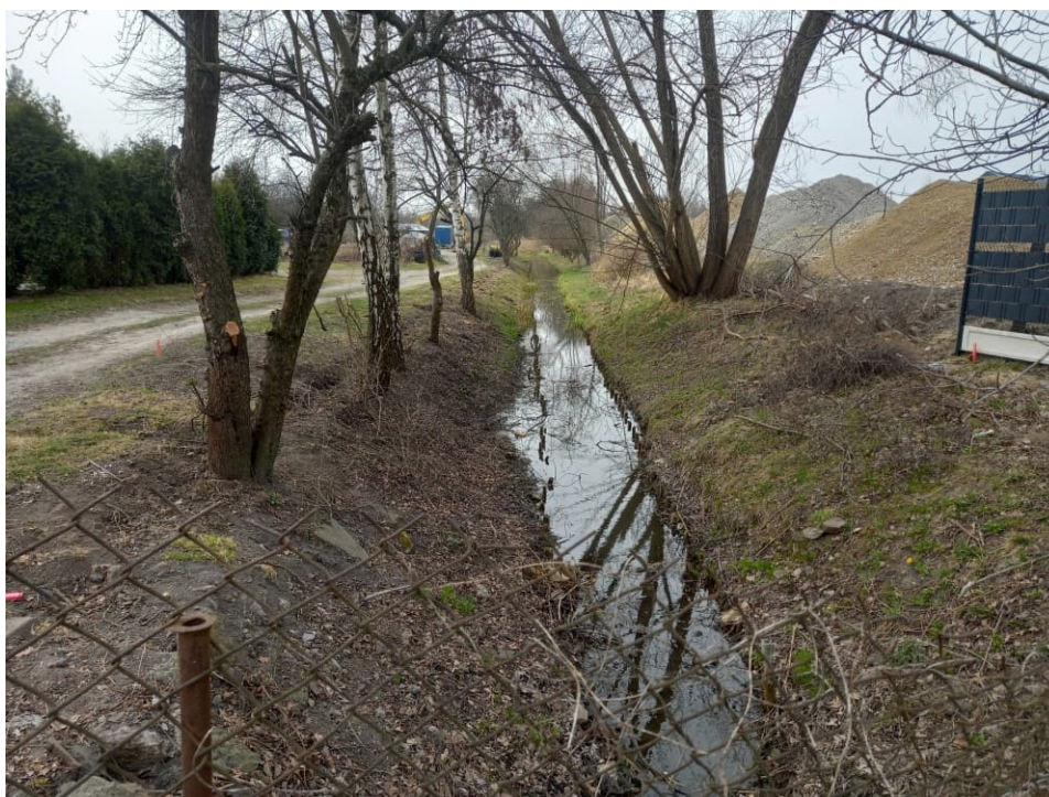
Fig. 8. Site condition in the first month of the works implementation period – redeveloped section of the Ditch 2 – upstream part, status in the third decade of March 2022 (view towards the west).
