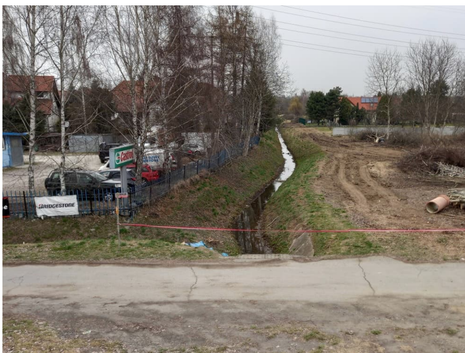
Fig. 2. Site condition in the first month of the works implementation period – construction area of an embankment lock on the Ditch 2a on the area beyond the Vistula River embankment, status in the third decade of March 2022 (view towards the north).
