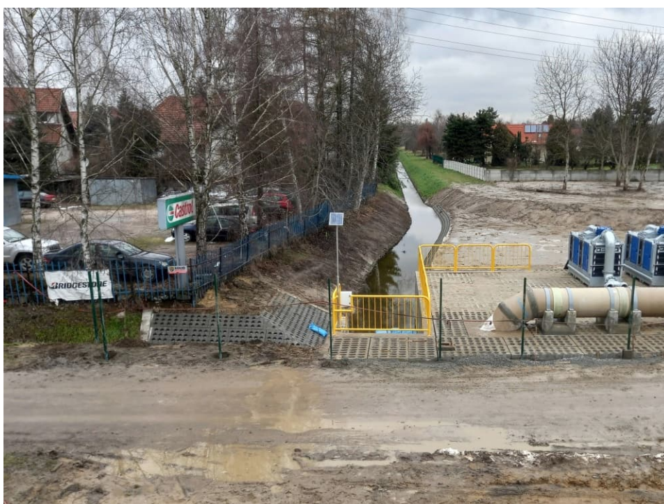
Fig. 50. Site condition in the last month of the works implementation period – construction area of an embankment lock on the Ditch 2a on the area beyond the Vistula River embankment, status in the third decade of January 2023 (view towards the north).
