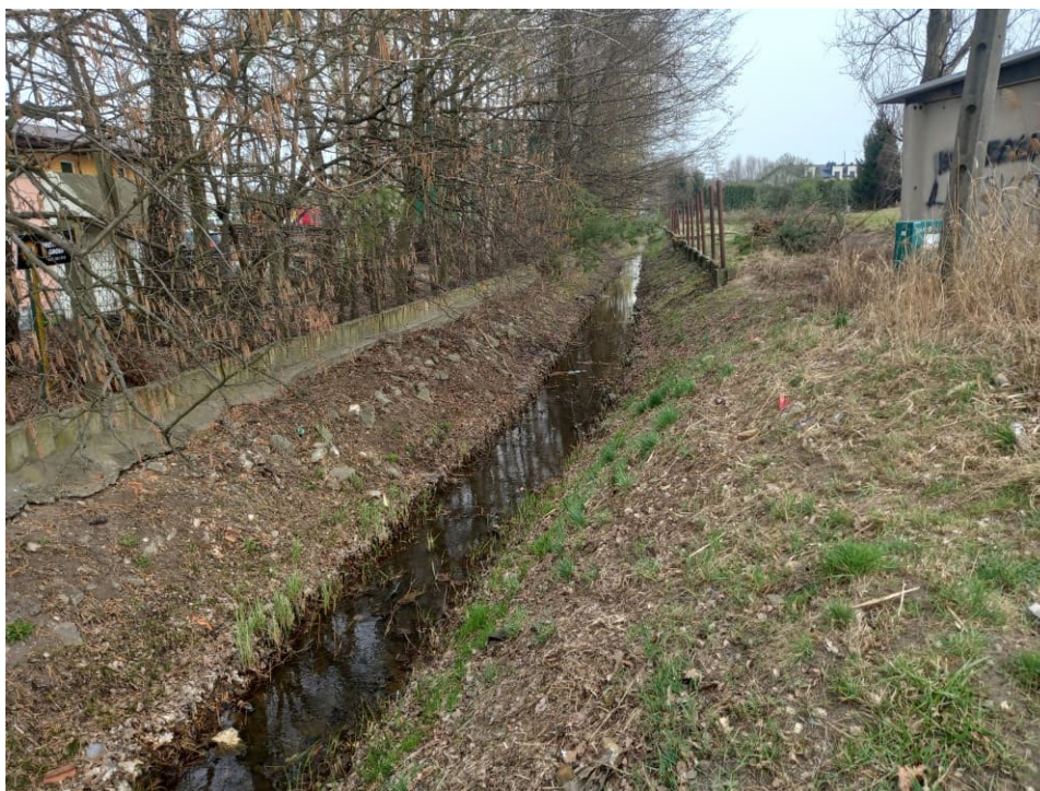
Fig. 7. Site condition in the first month of the works implementation period – redeveloped section of the Ditch 2 – downstream part, status in the third decade of March 2022 (view towards the east).
