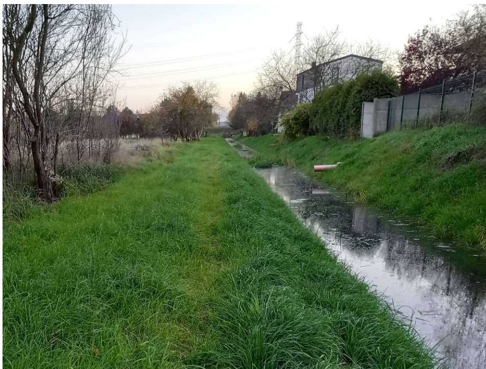
Fig. 43. Growth of grasses sown on the bank slopes on the Ditch 2a, status in the third decade of October 2022 (view towards the south).
