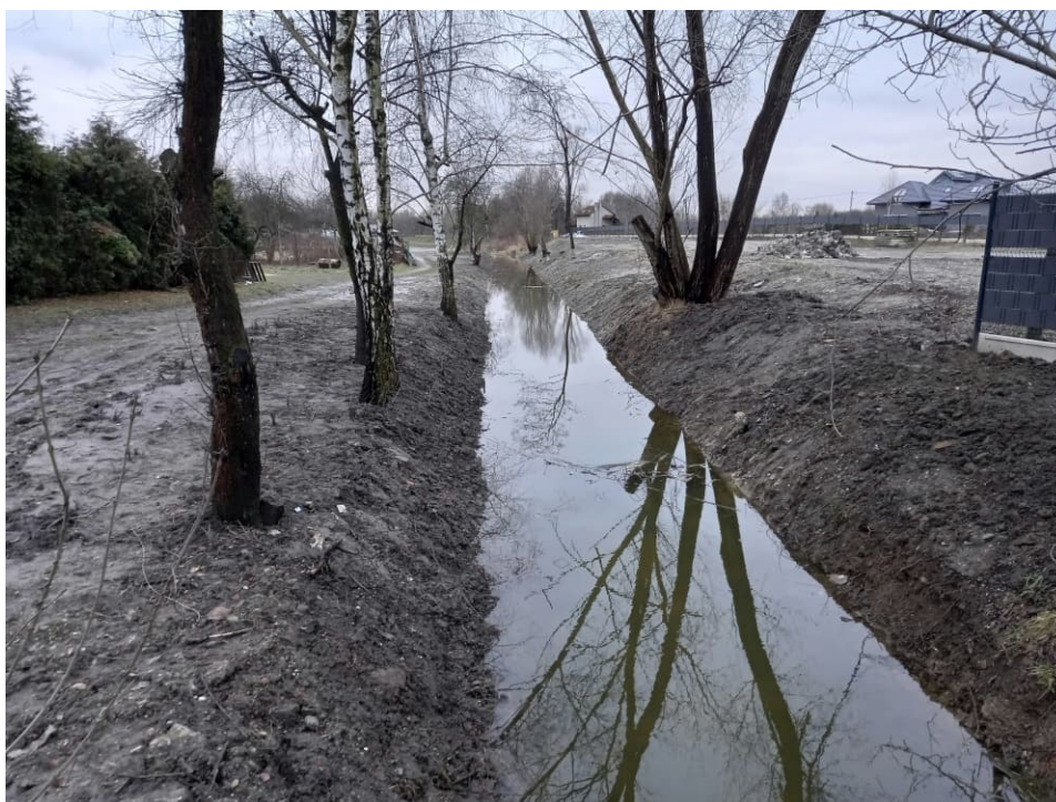
Fig. 56. Site condition in the last month of the works implementation period – redeveloped section of the Ditch 2 – upstream part, status in the third decade of January 2023 (view towards the west).
