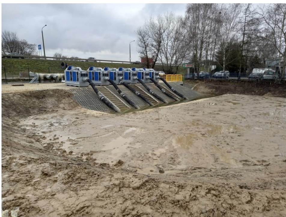
Fig. 52. Site condition in the last month of the works implementation period – construction area of a site flood storage reservoir upstream of the embankment lock and a pumping station for mobile pumps, status in the third decade of January 2023 (view towards the south).
