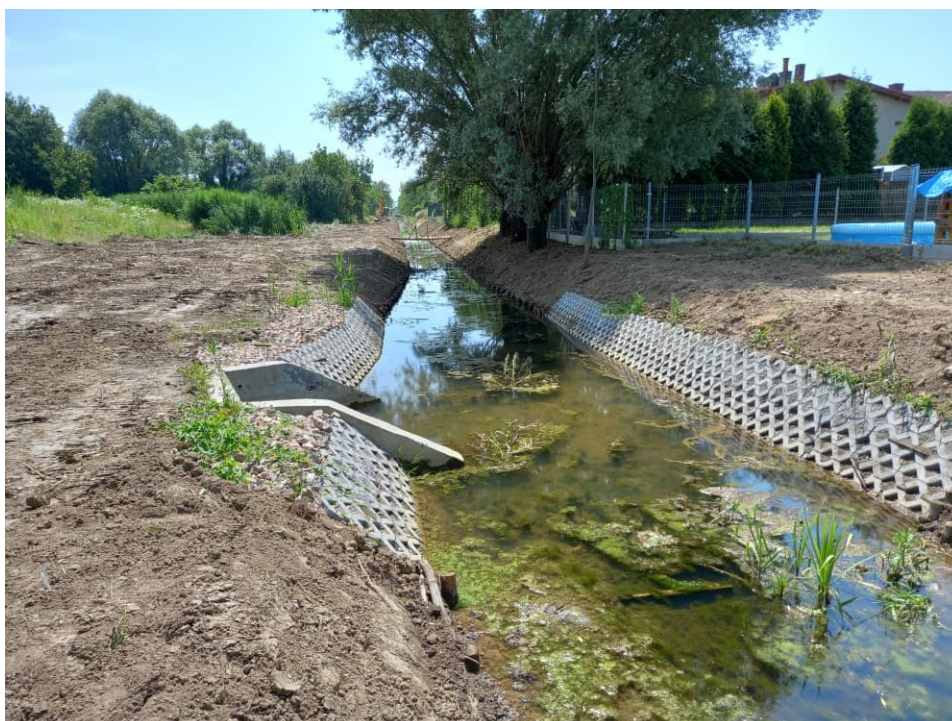
Fig. 42. Bank slopes insurance on the Ditch 2a, status in the third decade of September 2022 (view towards the south).
