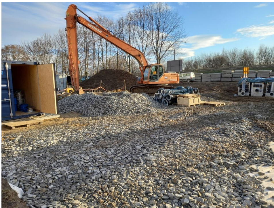
Fig. 39. Construction of a maneuvering yard at pumping station for mobile pumps on the Ditch 2a, status in the third decade of December 2022 (view towards the south-east).
