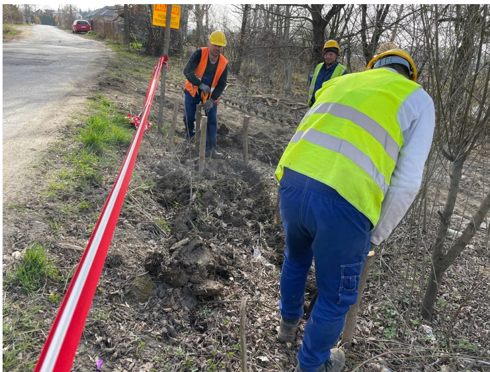
Fig. 29. Construction of herpetological fence on the northern bank of the redeveloped reservoir on the Ditch 2, status in the second half of April 2022 (view towards the east).
