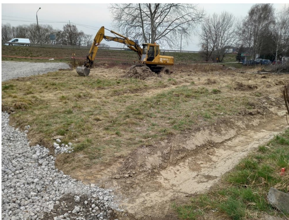
Fig. 4. Site condition in the first month of the works implementation period – construction area of a site flood storage reservoir upstream of the embankment lock and a pumping station for mobile pumps, status in the third decade of March 2022 (view towards the south).
