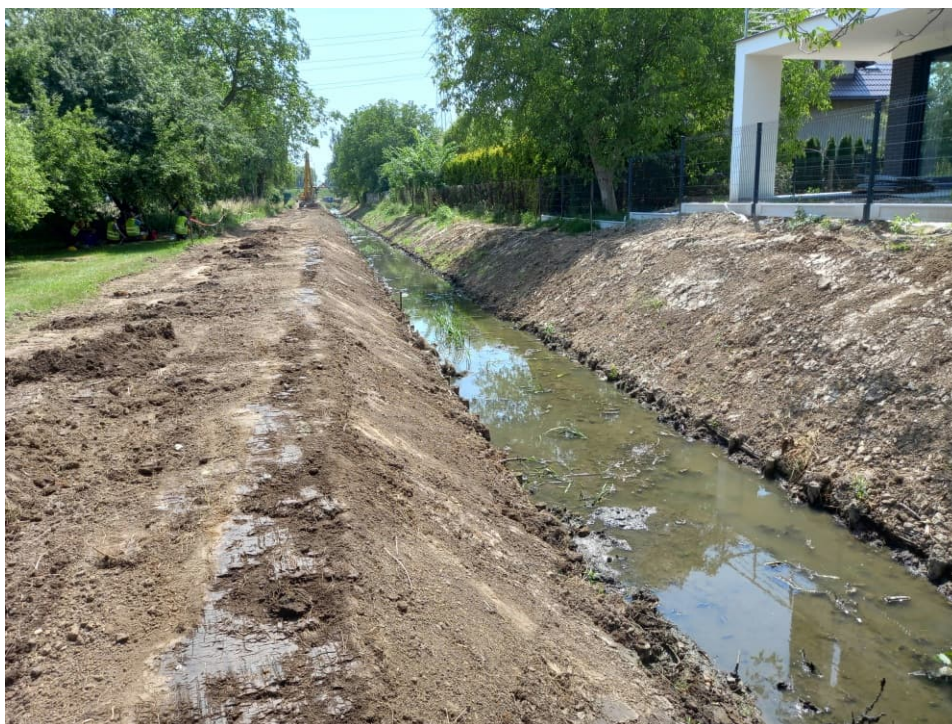
Fig. 41. Formation of bank slopes on the Ditch 2a, status in the third decade of June 2022 (view towards the south).
