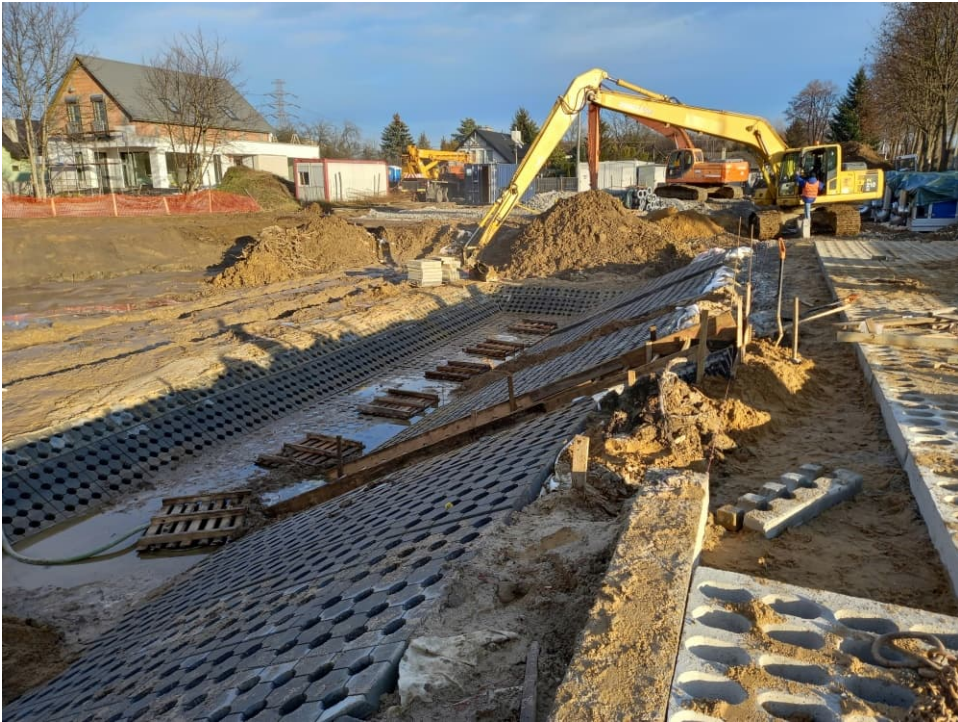
Fig. 37. Construction of a pumping station for mobile pumps on the Ditch 2a, status in the third decade of December 2022 (view towards the east).
