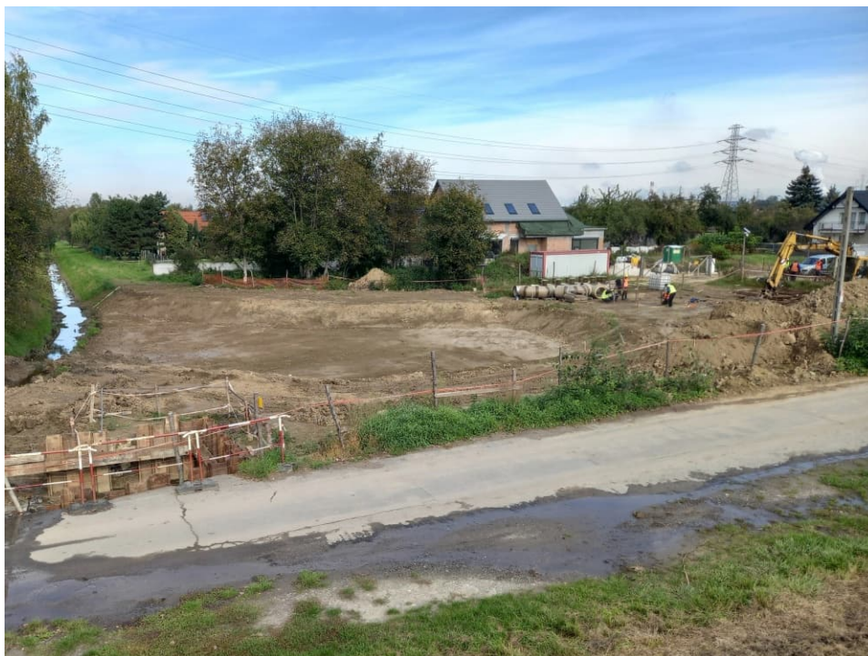
Fig. 36. Formation of slopes of flood storage reservoir on the Ditch 2a, status in the third decade of September 2022 (view towards the north).
