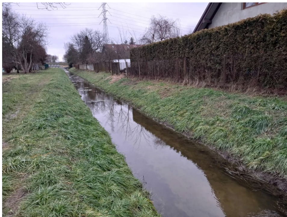
Fig. 53. Site condition in the last month of the works implementation period – redeveloped section of the Ditch 2a – downstream part, status in the third decade of January 2023 (view towards the south).
