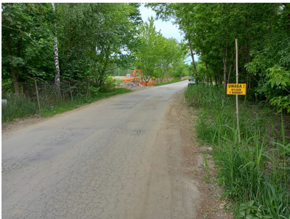
Fig. 18. Marking of the entrance to the construction site from the Odmetowa Street, status in the third decade of April 2022 (view towards the west).
