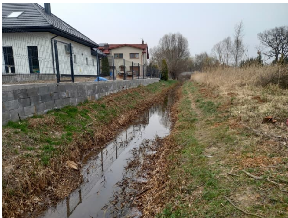
Fig. 6. Site condition in the first month of the works implementation period – redeveloped section of the Ditch 2a – upstream part, status in the third decade of March 2022 (view towards the north).
