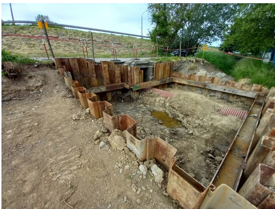
Fig. 22. Protection of hazardous sites on the construction area of embankment lock on the Ditch 2a within the area beyond the Vistula River embankment, status in the third decade of July 2022 (view towards the north).
