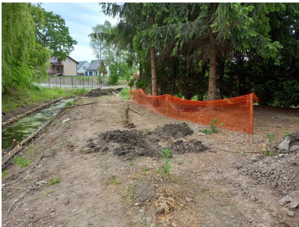
Fig. 25. Protection of trees not intended to felling in the vicinity of construction area on the Ditch 2, status in the third decade of May 2022 (view towards the east).
