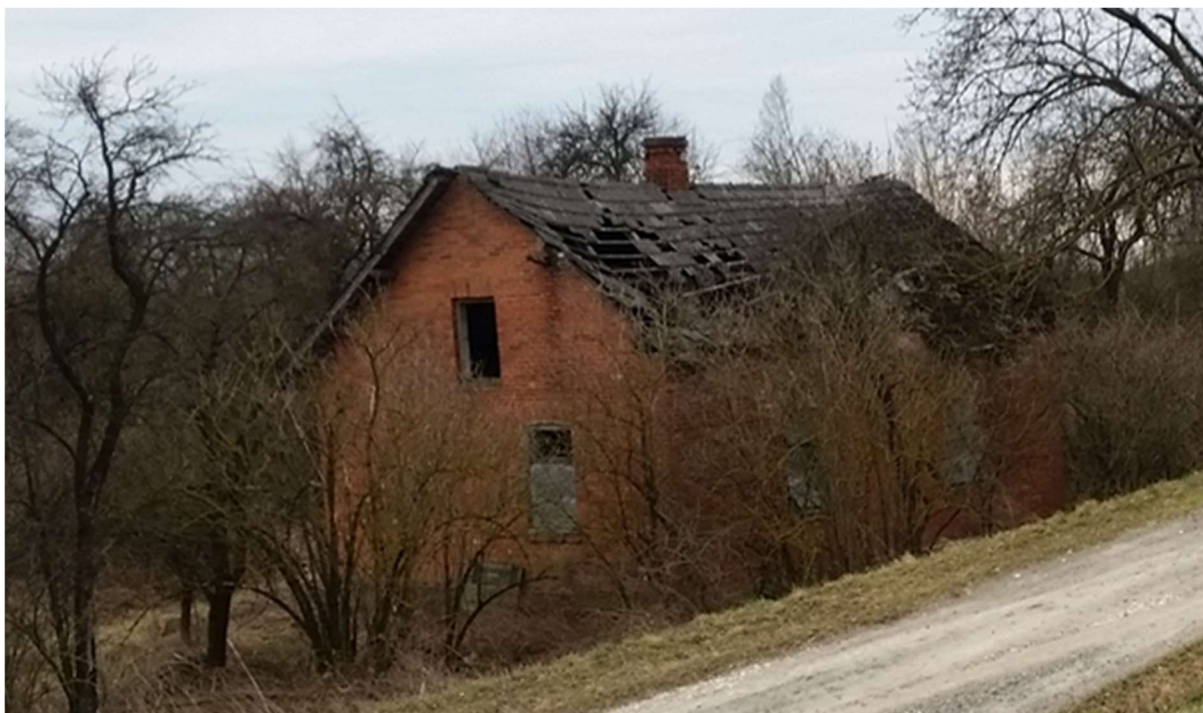
Photo no. 1. Ruin of a building (plot 975, Wrzawa precinct) - the ruin, the condition of which posed a threat to the safety of people, was demolished - km 1 + 730 Section II.
