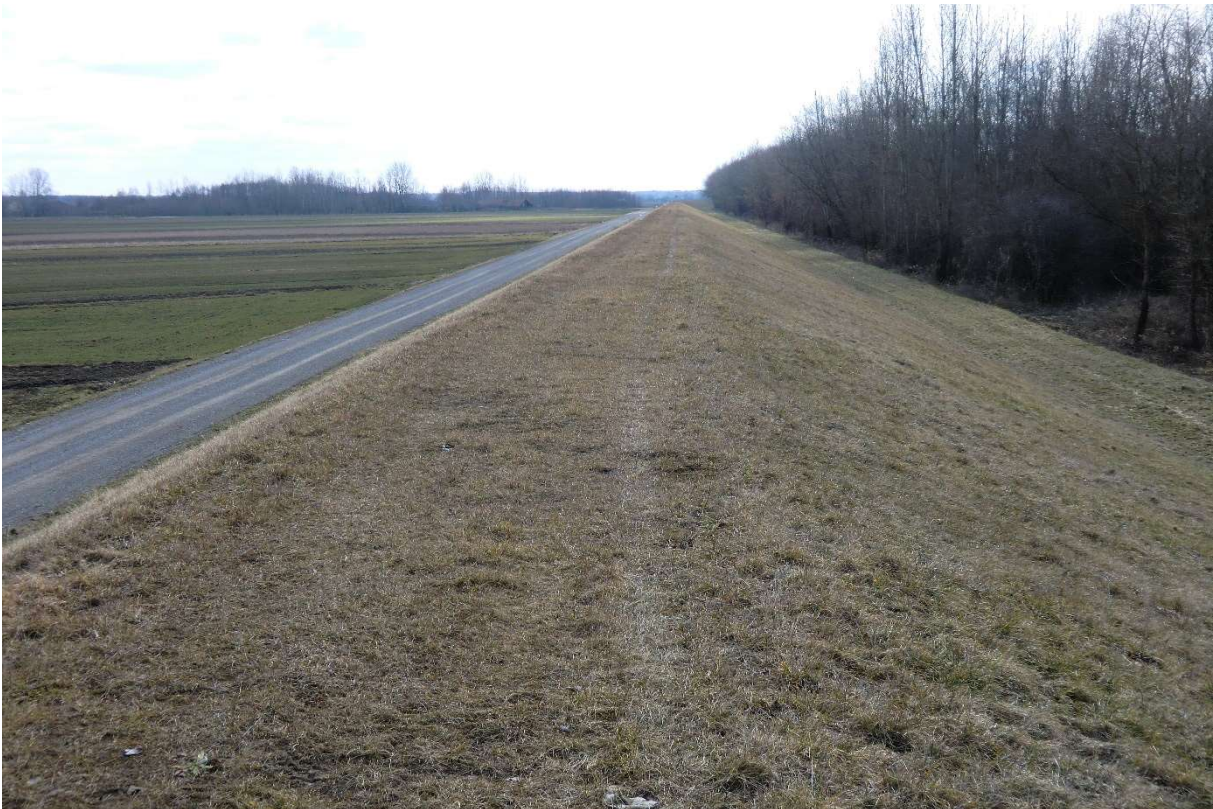
Photo no. 14. Extended San embankment (Section San 1+000) (source: own materials of AECOM Polska Sp. z o.o.).
