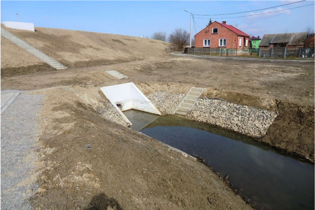
Photo no. 3. Completed embankment culvert redevelopment (Section I km 2+520 inlet to the lock) (source: own materials of AECOM Polska Sp. z o.o.).
