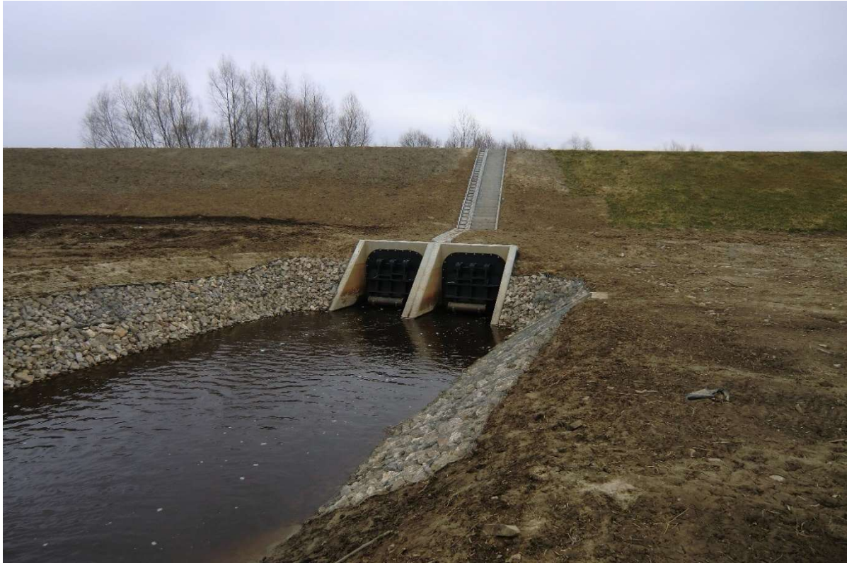
Photo no. 5. Part of the crest and of the landside embankment slope, with an inlet to the embankment lock (Section I km 6+200) (source: own materials of AECOM Polska Sp. z o.o.).
