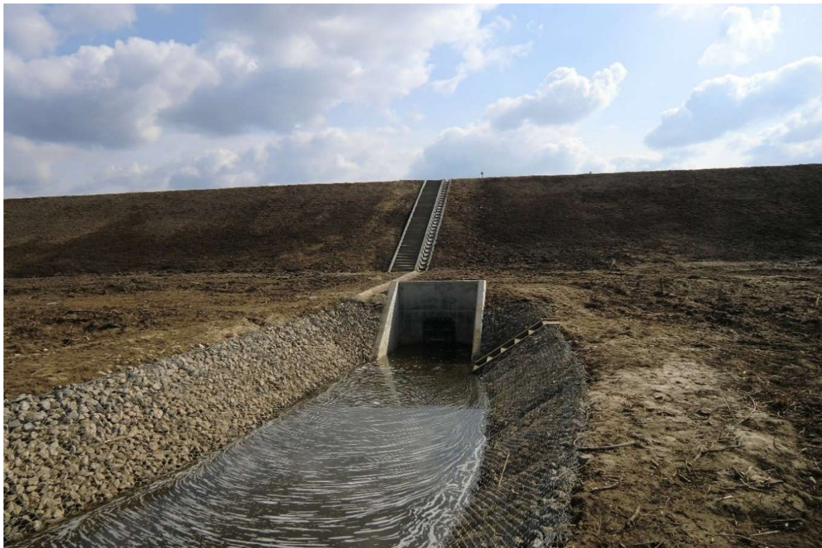
Photo no. 4. Part of the crest and of the landside embankment slope, with an inlet to the embankment lock (Section I km 4+093 inlet to the lock) (source: own materials of AECOM Polska Sp. z o.o.).
