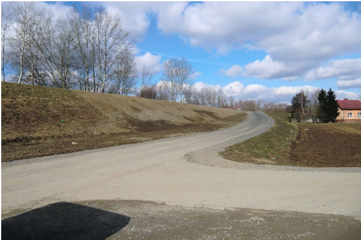
Photo no. 8. Extended embankment (Section II km 2+425) (source: own materials of AECOM Polska Sp. z o.o.).
