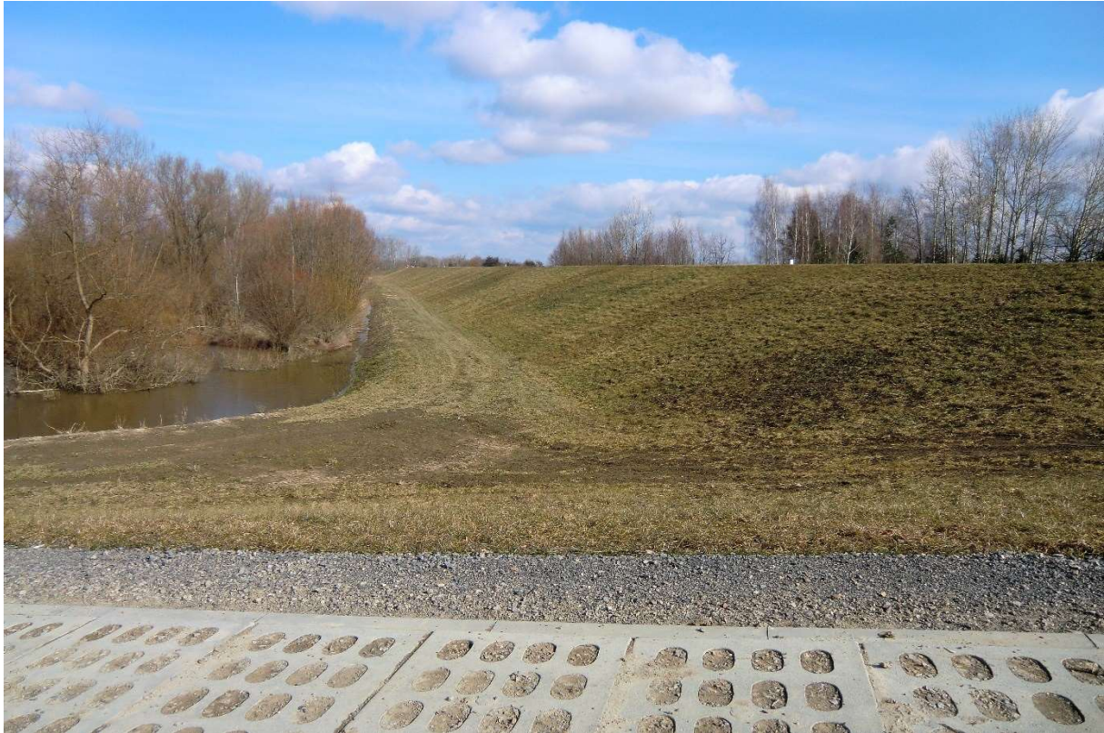
Photo no. 7. Part of the embankment (Section II km 2+149) (source: own materials of AECOM Polska Sp. z o.o.).
