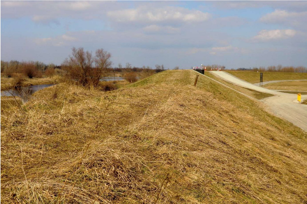
Photo no. 9. Extended embankment – connection with the Łęg embankment (Section II km 4+900) (source: own materials of AECOM Polska Sp. z o.o.).
