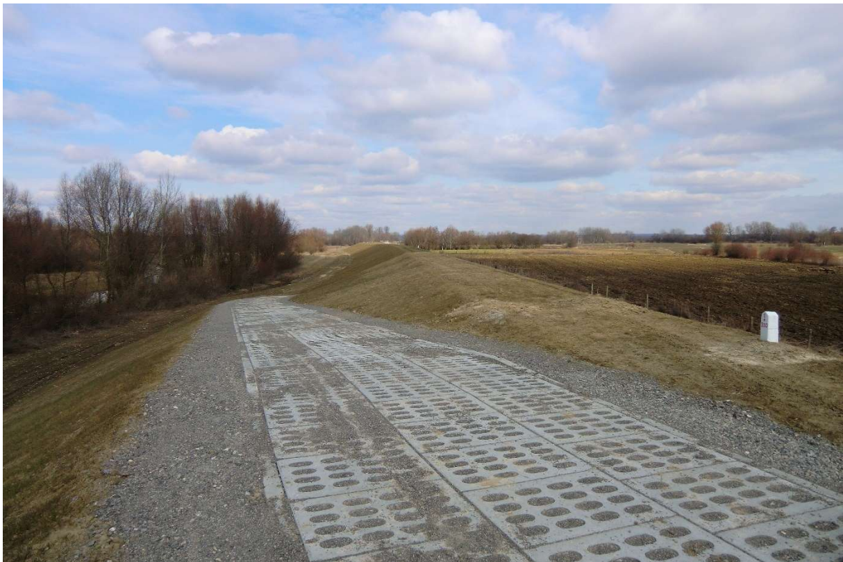
Photo no. 2. Completed embankment redevelopment (Section I km 1+310, embankment crossing) (source: own materials of AECOM Polska Sp. z o.o.).
