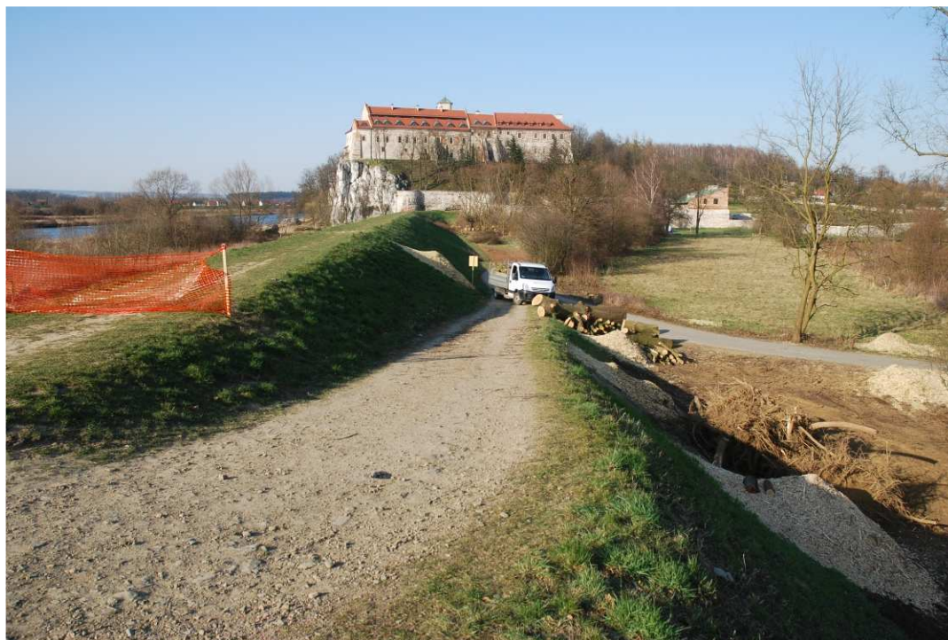
Fig. 8. Cleaning up after felling trees within Task 2 , status in the third decade of March 2020 (downstream view).
