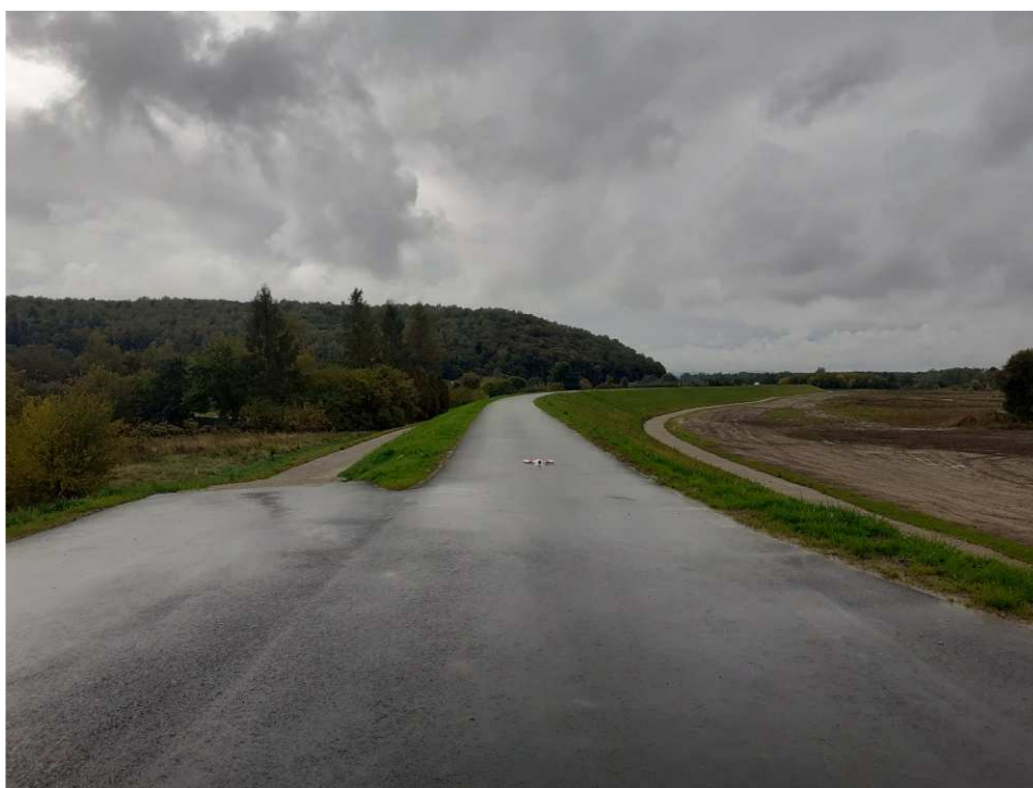
Fig. 43. Site condition in the last month of the works implementation period – the right Vistula embankment within Task 2 , status in the third decade of September 2022 (upstream view).
