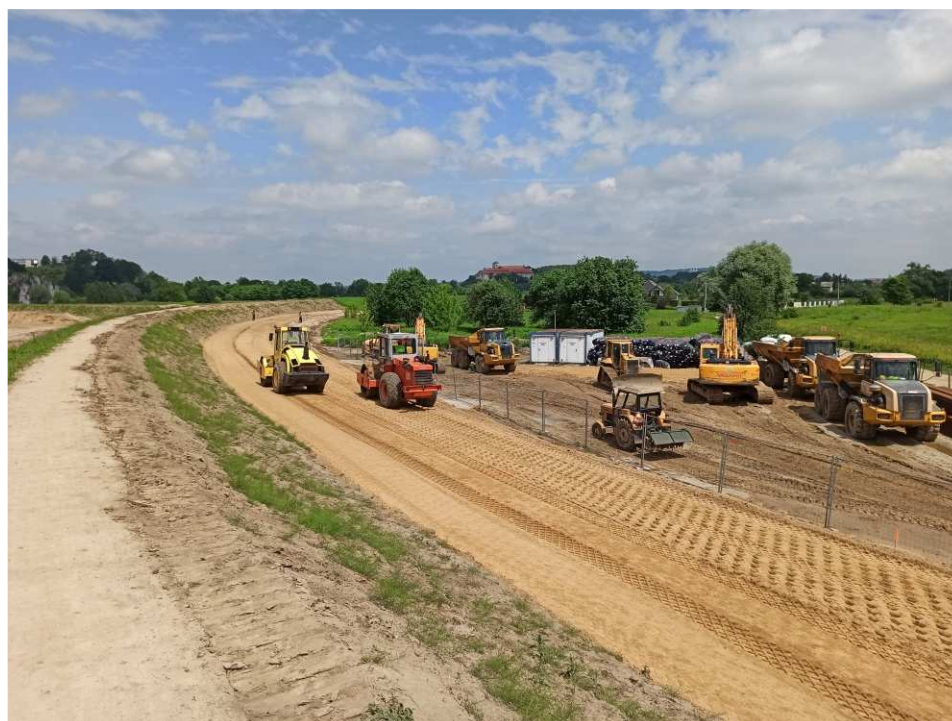
Fig. 10. Site facilities in the area beyond the right Vistula embankment at the height of Task 2 , status in the third decade of June 2020 (downstream view).
