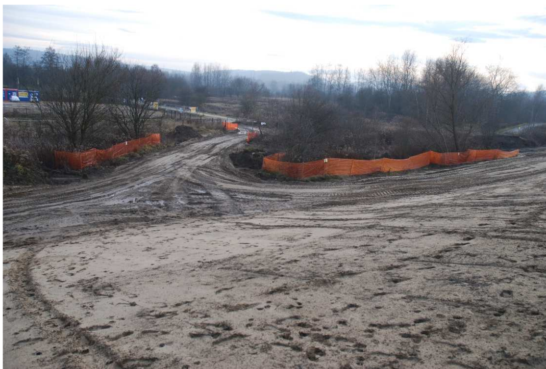
Fig. 20. Protection of trees and shrubs not intended to felling within Task 3 , status in the third decade of December 2020 (view towards the area beyond the embankment).
