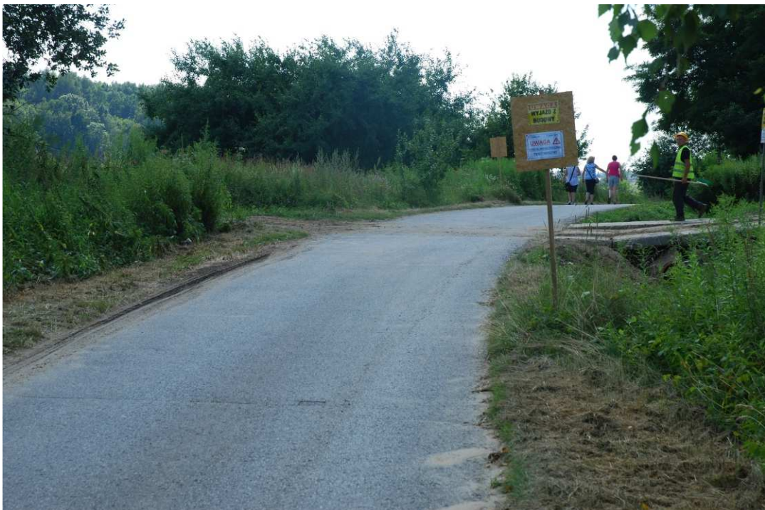
Fig. 12. Marking and keeping the public road clean near the exit from the construction site within Task 3 , status in the third decade of July 2020 (upstream view).
