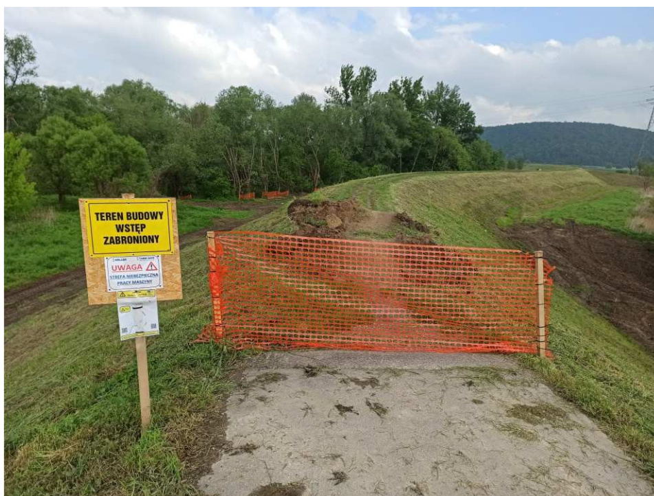
Fig. 13. Marking of the construction site within Task 1 , status in the third decade of May 2020 (downstream view).
