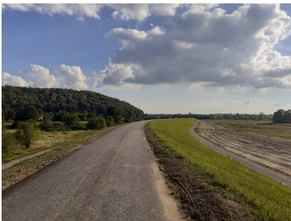
Fig. 40. Growth of grasses sown on the slope of the flood embankment within Task 2 , status in the third decade of August 2022 (upstream view).
