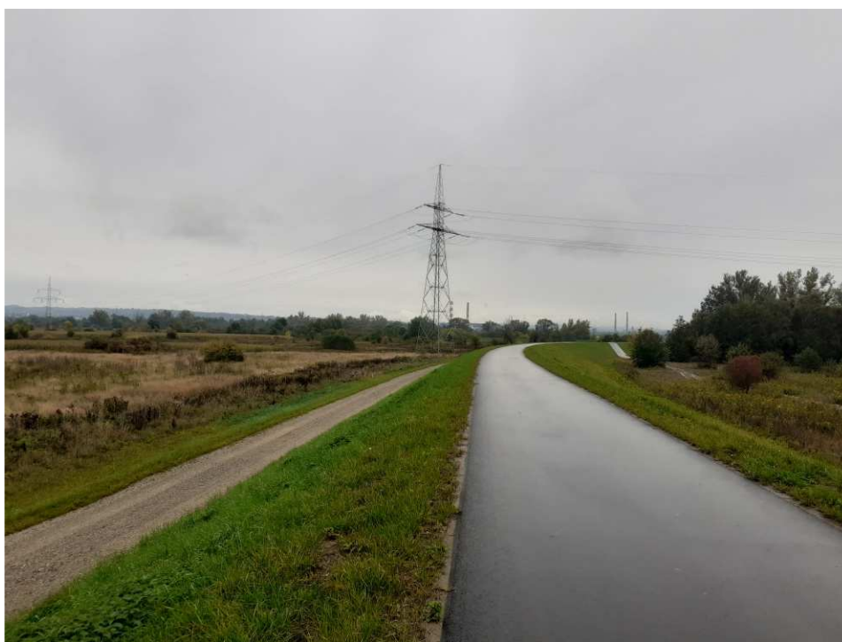
Fig. 41. Site condition in the last month of the works implementation period – the right Vistula embankment within Task 1 , status in the third decade of September 2022 (upstream view).
