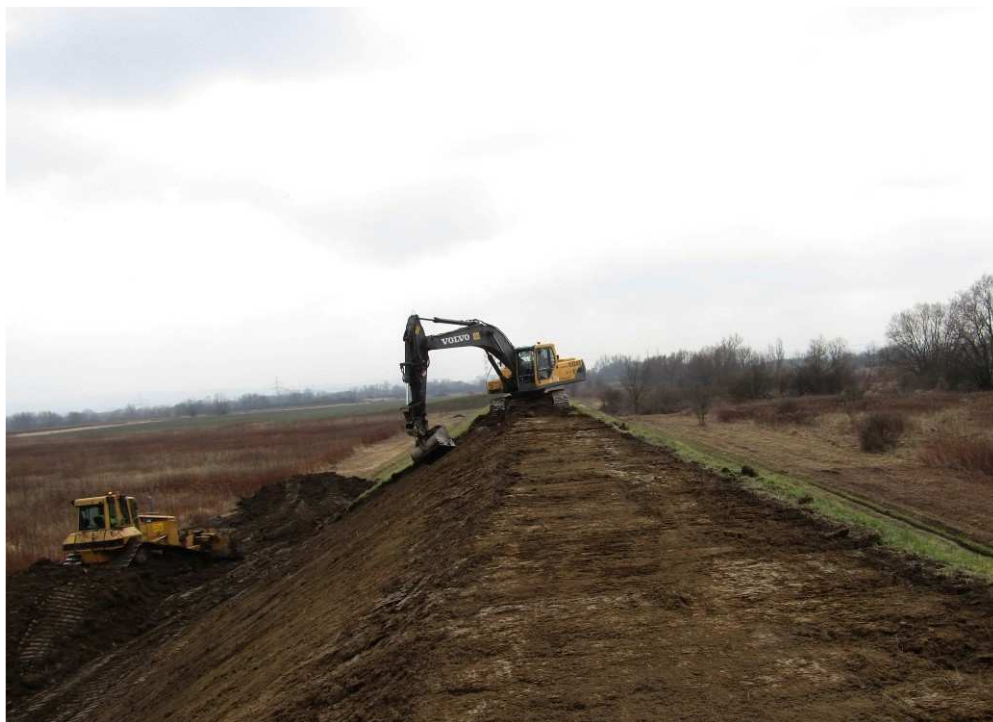
Fig. 21. Removal of a top-soil layer within Task 1 , status in the third decade of February 2020 (upstream view).
