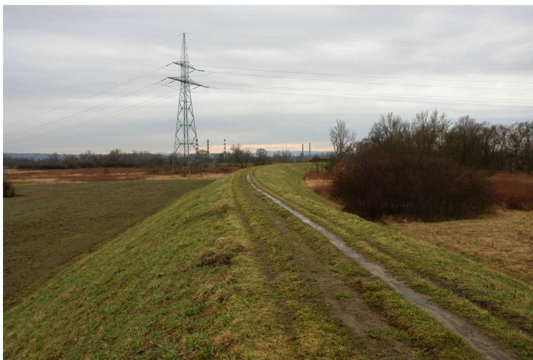
Fig. 1. Site condition in the first month of the works implementation period – the right Vistula embankment within Task 1 , status in the third decade of February 2020 (upstream view).
