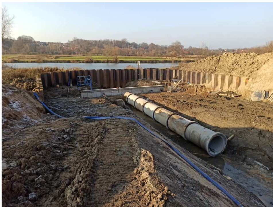
Fig. 26. Redevelopment of the embankment culvert at km 63+115 of the Vistula embankment on Task 2 , status in the third decade of November 2020 (view towards the embanked area).
