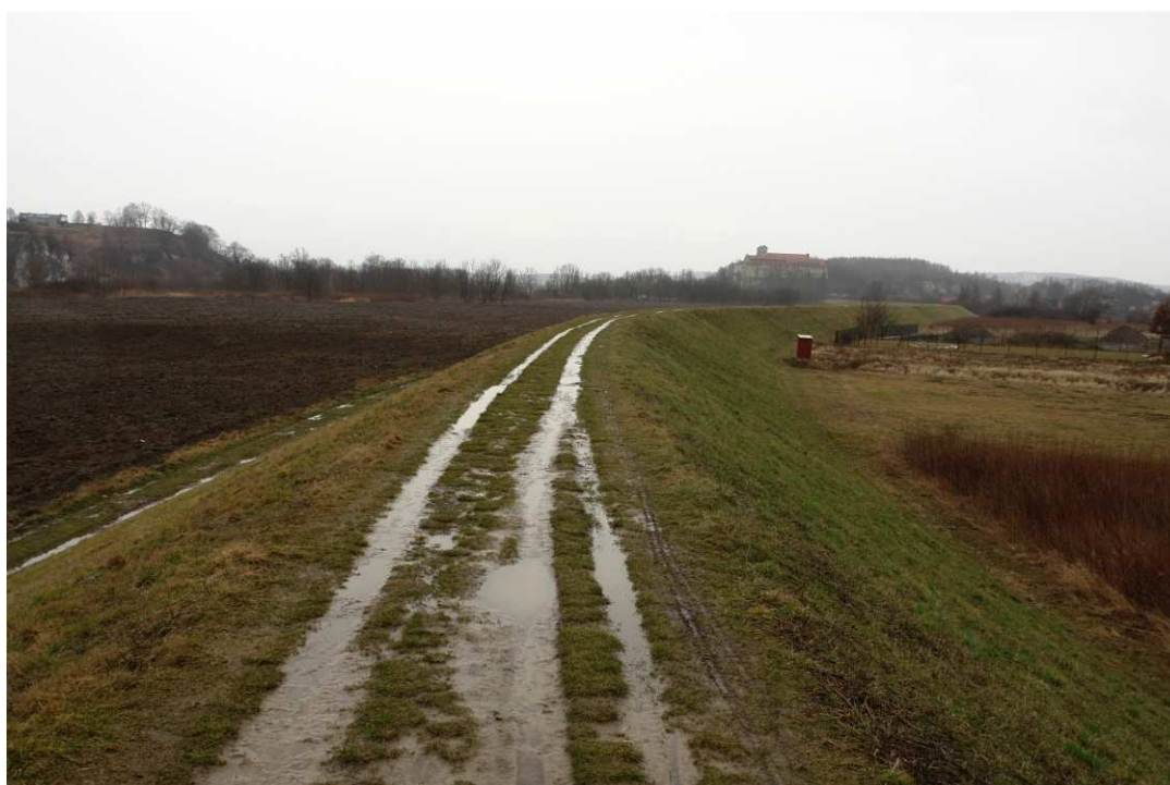
Fig. 4. Site condition in the first month of the works implementation period – the right Vistula embankment within Task 2 , status in the third decade of February 2020 (downstream view).
