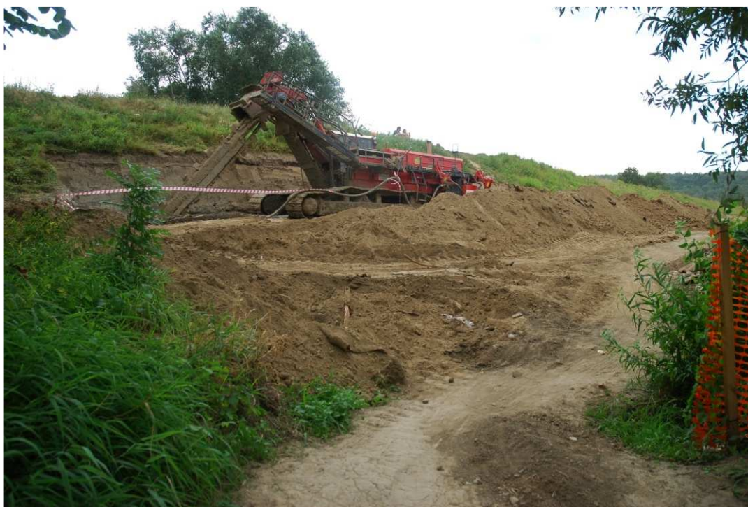
Fig. 29. Construction of a cement-bentonite barrier within Task 2 , status in the third decade of August 2020 (upstream view).
