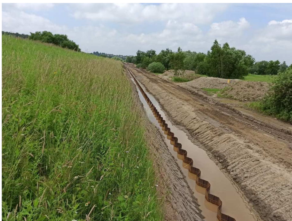
Fig. 28. Construction of a sheet piling barrier within Task 3 , status in the third decade of June 2020 (upstream view).
