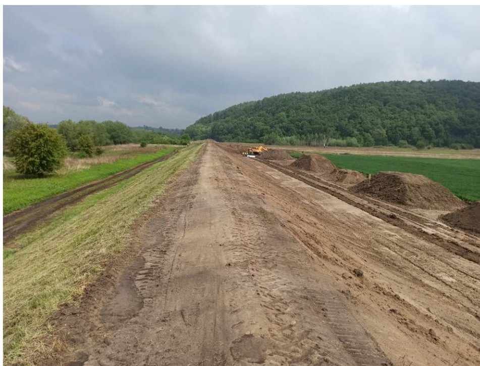
Fig. 23. Protection of top-soil piles within Task 1 , status in the third decade of May 2020 (downstream view).
