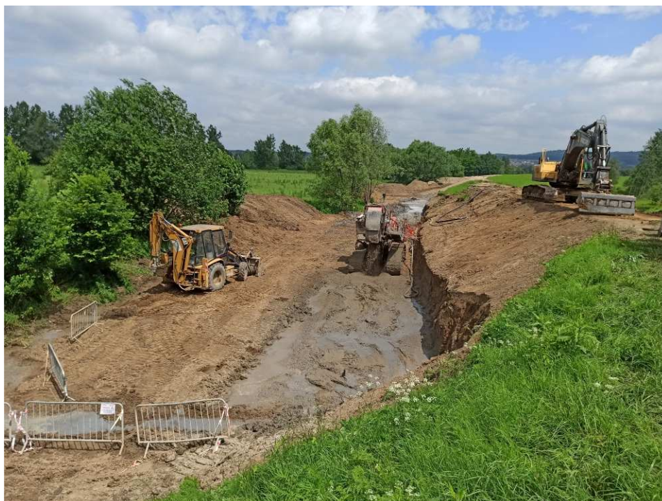
Fig. 30. Construction of a cement-bentonite barrier within Task 3 , status in the third decade of June 2020 (downstream view).
