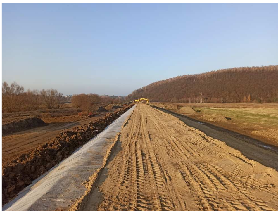
Fig. 34. Placement of bentomat on the slope of the flood embankment within Task 1 , status in the third decade of November 2020 (downstream view).
