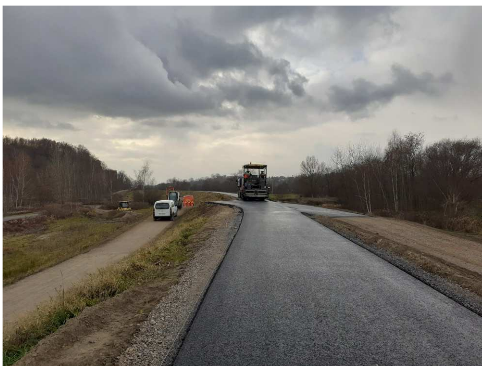
Fig. 38. Construction of a road on the crown of the flood embankment within Task 3 , status in the third decade of November 2021 (upstream view).
