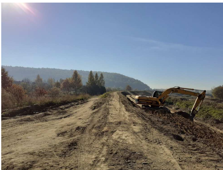
Fig. 36. Covering slopes of the flood embankment with a top-soil layer within Task 2 , status in the third decade of October 2021 (upstream view).
