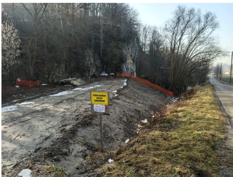
Fig. 14. Marking of the construction site within Task 3 , status in the third decade of February 2021 (upstream view).
