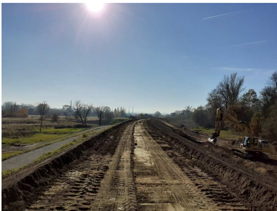
Fig. 35. Covering slopes of the flood embankment with a top-soil layer within Task 1 , status in the third decade of October 2021 (upstream view).
