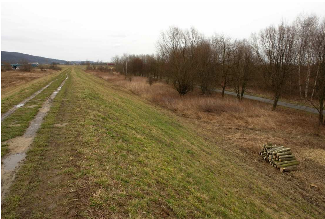
Fig. 6. Site condition in the first month of the works implementation period – the right Vistula embankment within Task 3 , status in the third decade of February 2020 (downstream view).
