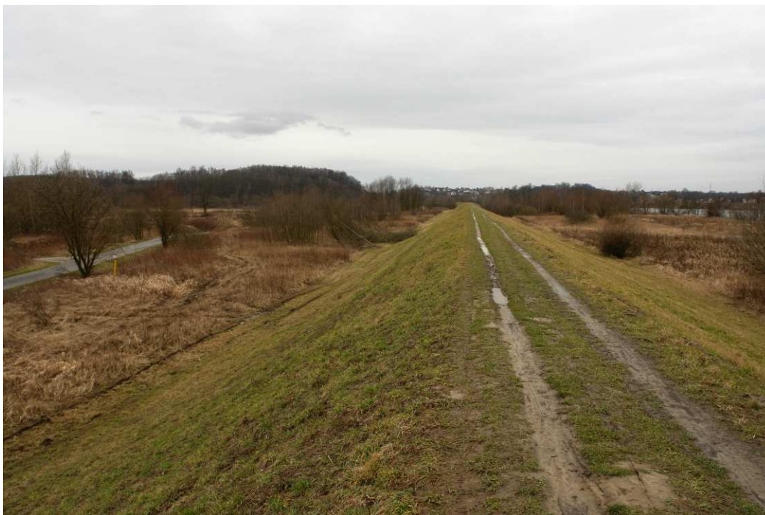
Fig. 5. Site condition in the first month of the works implementation period – the right Vistula embankment within Task 3 , status in the third decade of February 2020 (upstream view).
