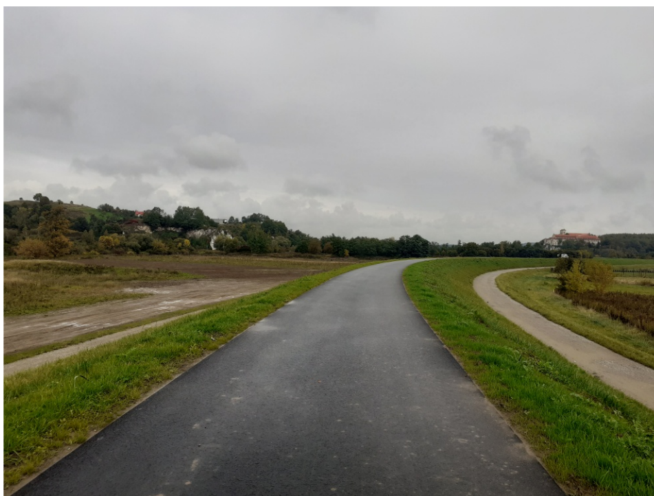
Fig. 44. Site condition in the last month of the works implementation period – the right Vistula embankment within Task 2 , status in the third decade of September 2022 (downstream view).
