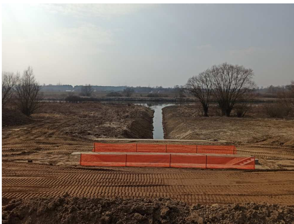
Fig. 16. Protection of hazardous sites within Task 1 , status in the third decade of March 2021 (view towards the embanked area).
