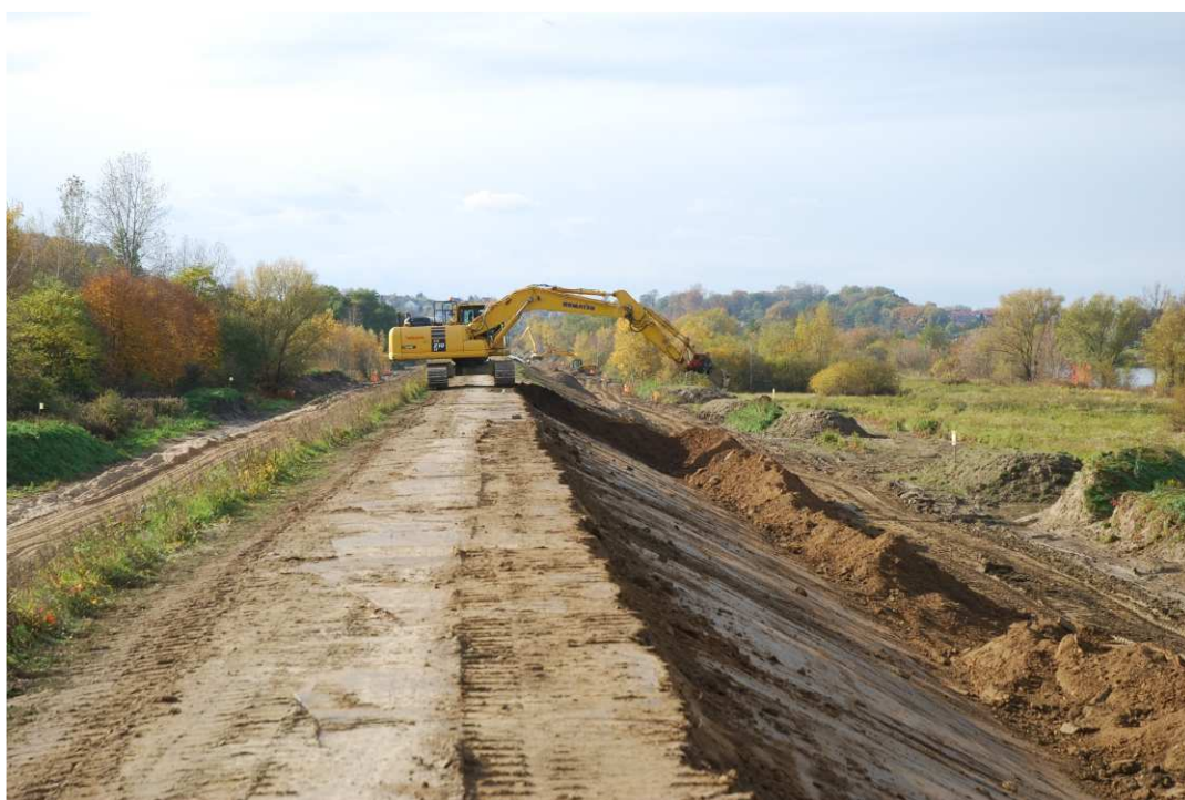
Fig. 32. Shaping the slopes of the flood embankment within Task 3 , status in the third decade of September 2020 (upstream view).
