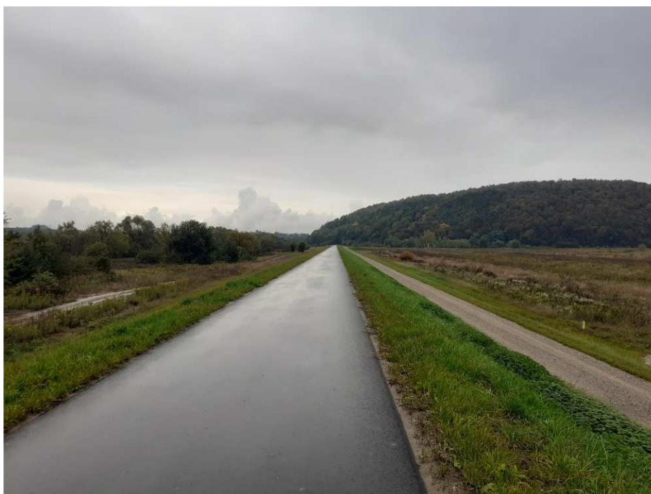
Fig. 42. Site condition in the last month of the works implementation period – the right Vistula embankment within Task 1 , status in the third decade of September 2022 (downstream view).
