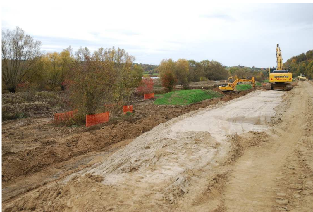
Fig. 17. Protection of trees and shrubs not intended to felling within Task 1 , status in the third decade of October 2020 (downstream view).
