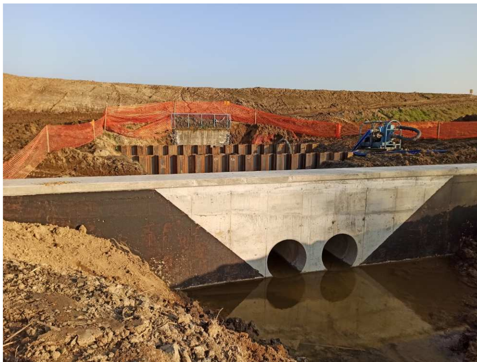
Fig. 25. Redevelopment of the embankment culvert at km 61+239 of the Vistula embankment on Task 1 , status in the third decade of November 2020 (view from the embanked area).
