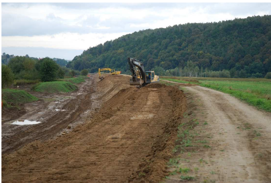
Fig. 31. Shaping the slopes of the flood embankment within Task 1 , status in the third decade of September 2020 (downstream view).
