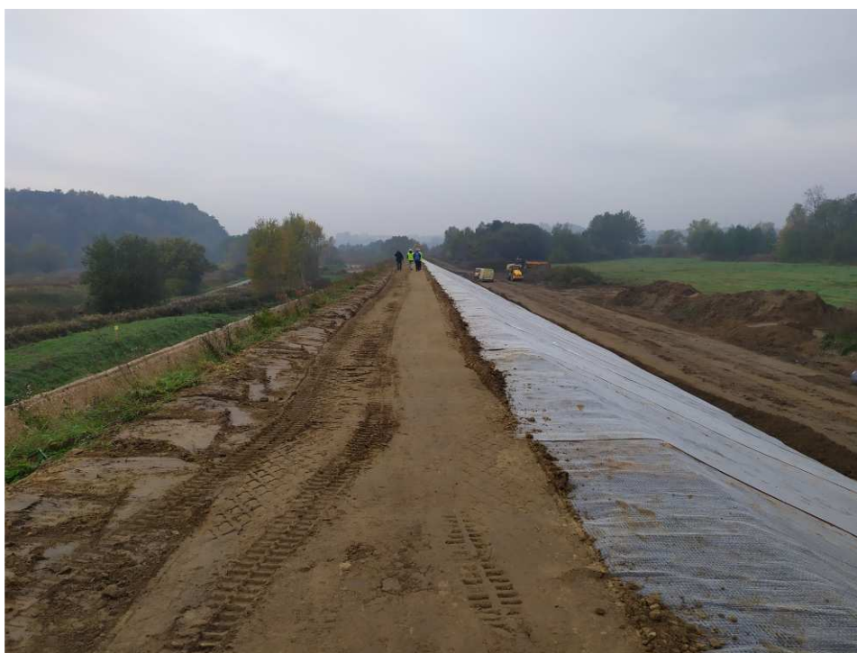
Fig. 33. Placement of bentomat on the slope of the flood embankment within Task 3 , status in the third decade of October 2020 (upstream view).
