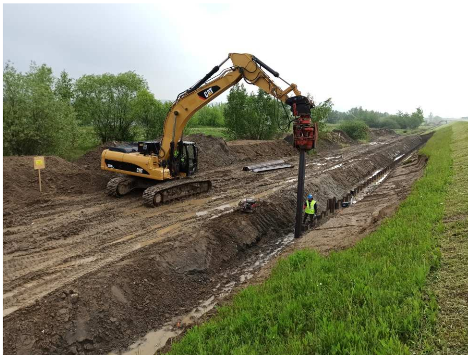
Fig. 27. Construction of a sheet piling barrier within Task 3 , status in the third decade of May 2020 (downstream view).
