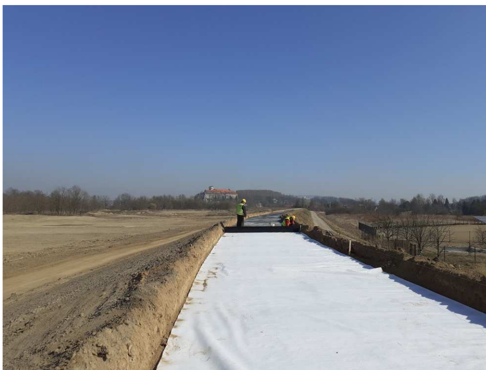
Fig. 37. Construction of a road on the crown of the flood embankment within Task 2 , status in the third decade of March 2022 (downstream view).
