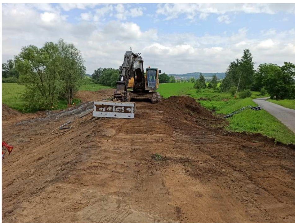
Fig. 22. Removal of a top-soil layer within Task 3 , status in the third decade of June 2020 (downstream view).
