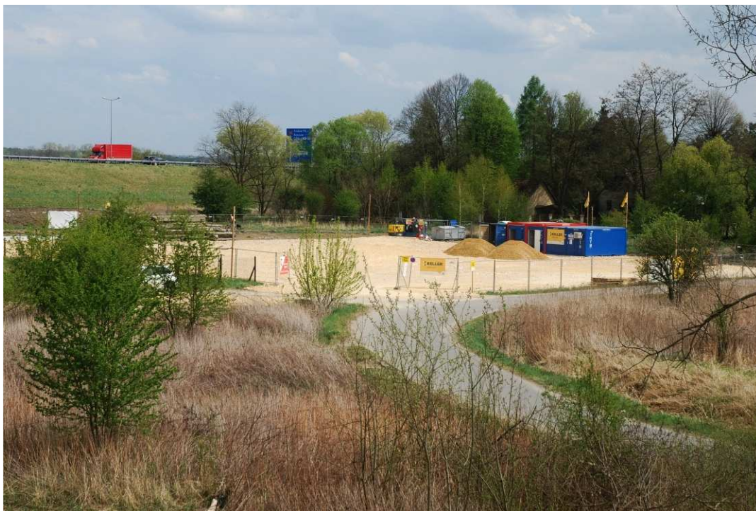
Fig. 9. Site facilities in the area beyond the right Vistula embankment at the height of Task 3 , status in the third decade of April 2020 (view towards the south-east).
