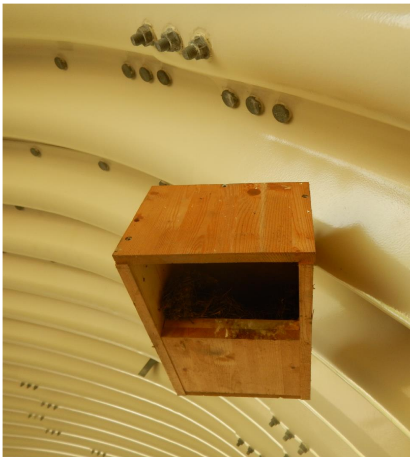
Photo.9. Dipper box installed in the investment premises under the new bridge over Nowinka stream - Contract implementation stage.
