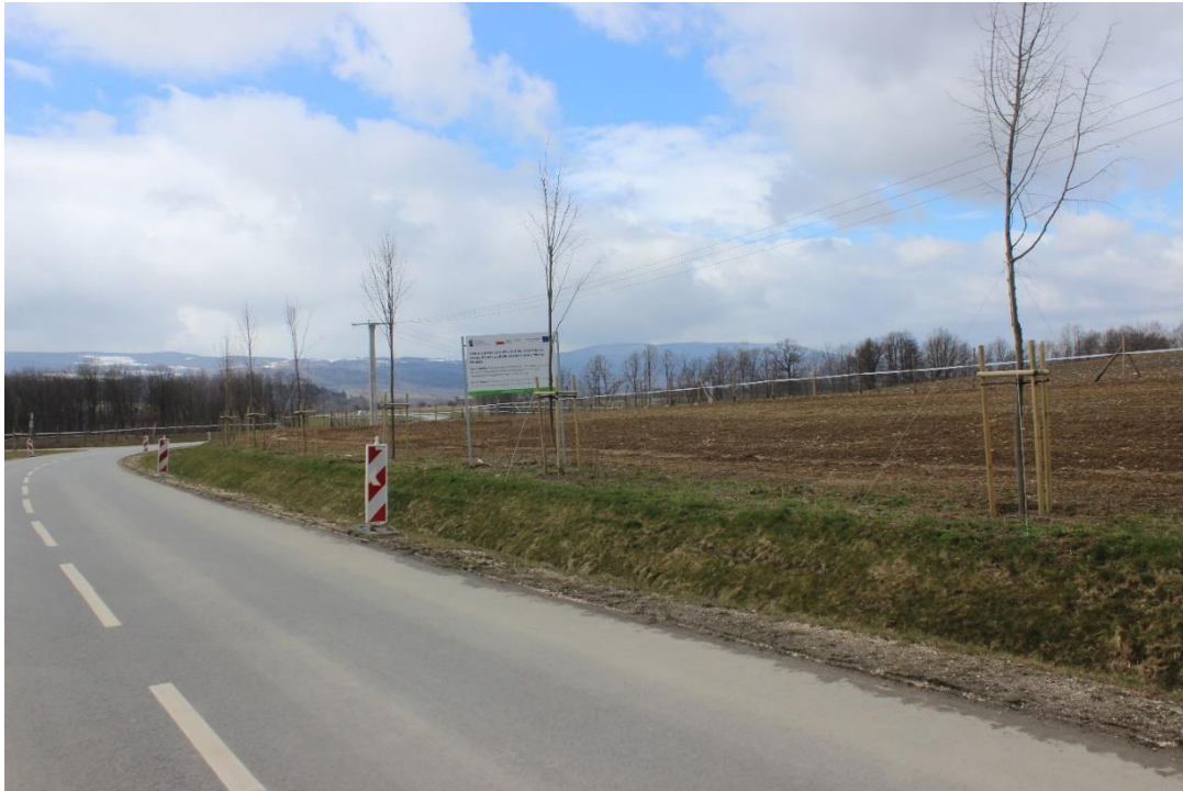
Photo.3. Newly-built section of the 3233D county road. Plantings of trees can be seen along the road - Contract implementation stage.
