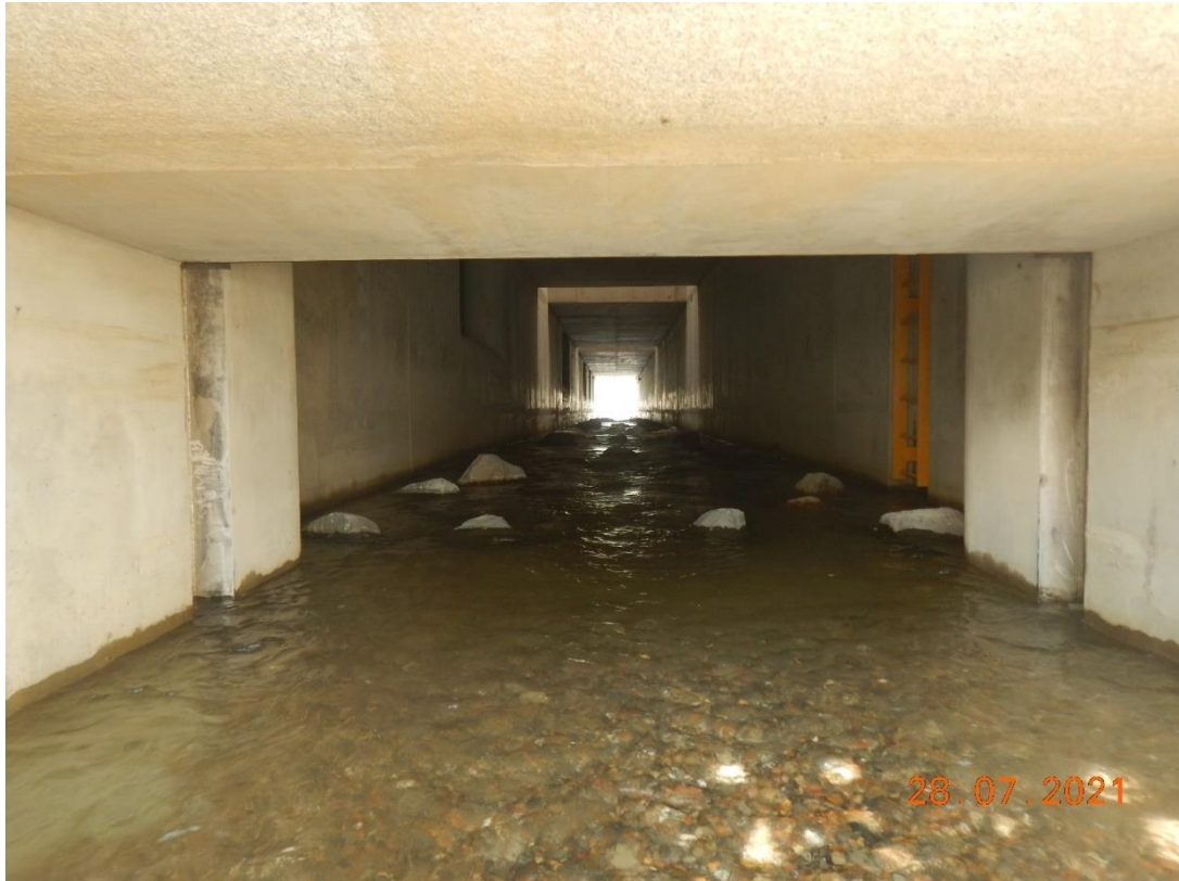
Photo.5. Layout of the Goworówka stream bed in the gallery under the reservoir dam - Contract implementation stage.
