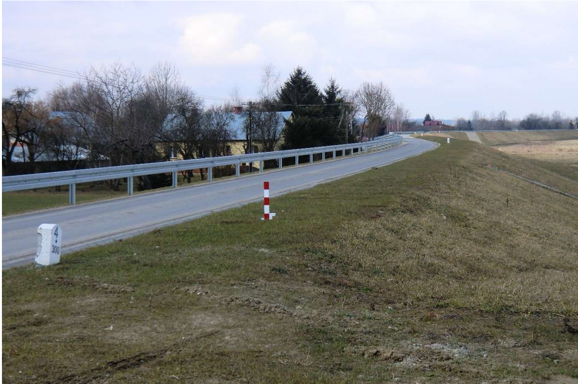
Photo no. 8. Completed embankment redevelopment (San III km 4.315 – public road on the embankment crest) (source: own materials of AECOM Polska Sp. z o.o.).
