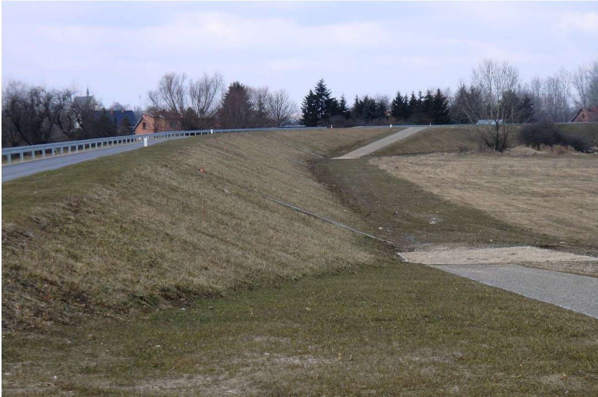
Photo no. 7. Completed embankment redevelopment (San III km 3.895 – descent road to the embanked area) (source: own materials of AECOM Polska Sp. z o.o.).
