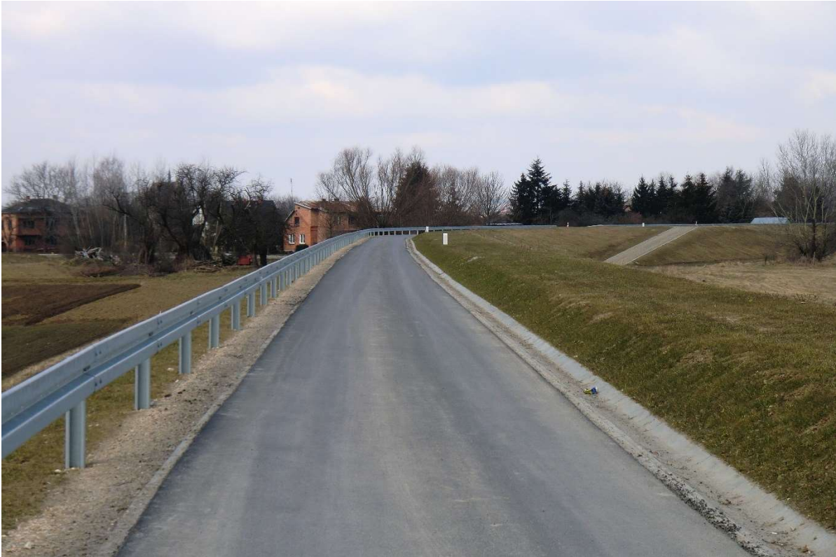
Photo no. 6. Completed embankment redevelopment (San III km 3.895 – public road on the embankment crest) (source: own materials of AECOM Polska Sp. z o.o.).
