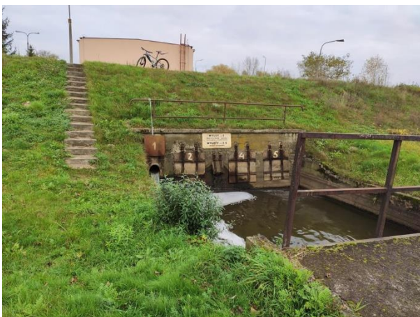
Photo no. 8: Outlet of storm drainage, treatment plant in the background.
