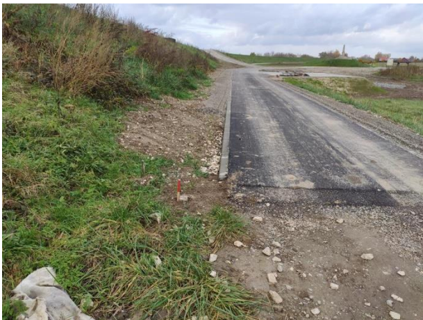
Photo no. 26: Beginning of the investment at the right embankment (at the Vistula River).
