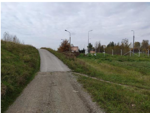
Photo no. 5: Access road onto the embankment at the treatment plant (asphalt course).
