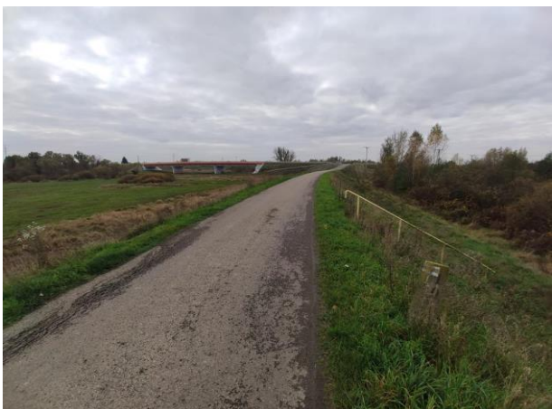
Photo no. 5: Culvert, valve at the water course running through the embankment.
