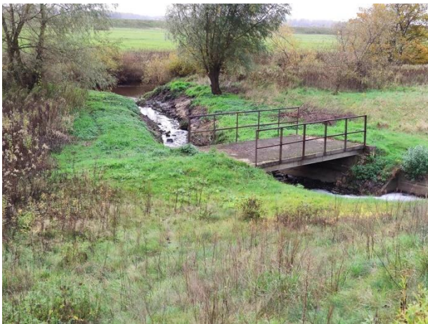
Photo no. 7: Discharge of water from the treatment plant, bridge.
