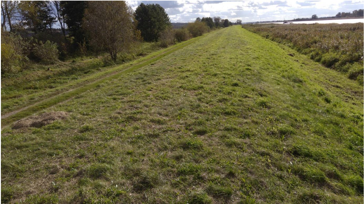
September 2017, Marwice - Krajnik, condition of embankments before the modernization
