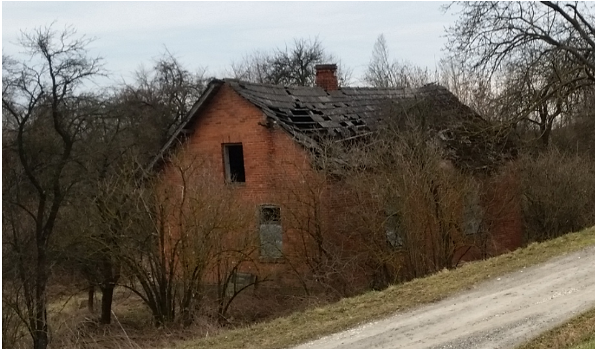
Fig. 4 Building planned to be demolished (the land plot no. 975, the precinct of Wrzawy).
