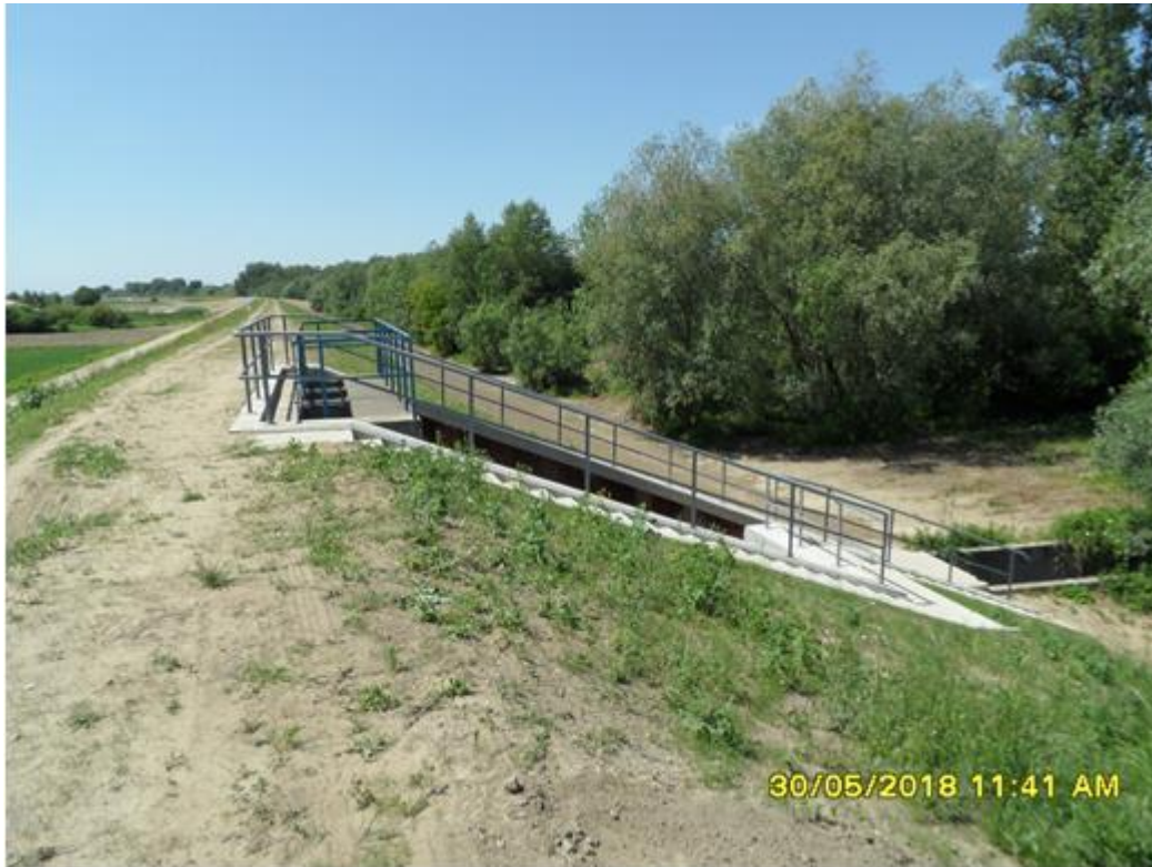
Photo 2. The reconstructed embankment culvert (outlet from the sewage treatment plant at km 9+589 – chainage in line with the building design) (source: own resources of Aecom Polska Sp. z o.o.).
