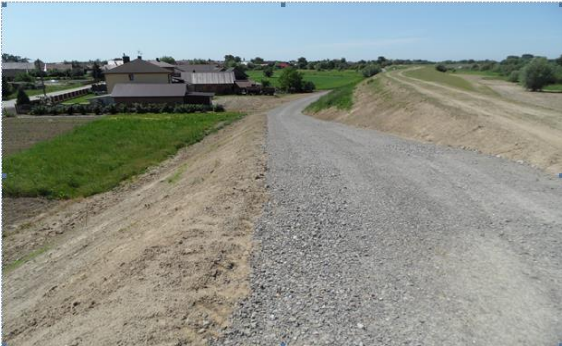
Photo 5. Works completed in the vicinity of the residential area (km 7+500 – 7+700 in line with the building design) (source: the Contractor's Monthly Report).
