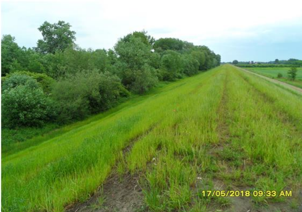
Photo 3. Part of the crown and water side slope of the embankment, ca. at km 9+500 in line with the building design (source: the Contractor's Monthly Report).
