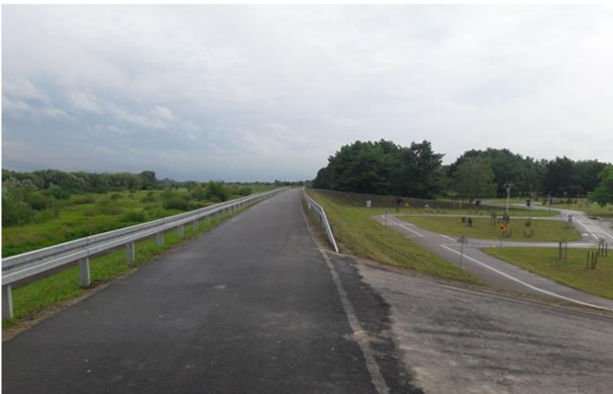
Photo 7. The extended embankment (km 9+535 in line with the agreement with the Catchment Board in Sandomierz in line with the building design km 15+485) (source: the Contractor's Monthly Report).
