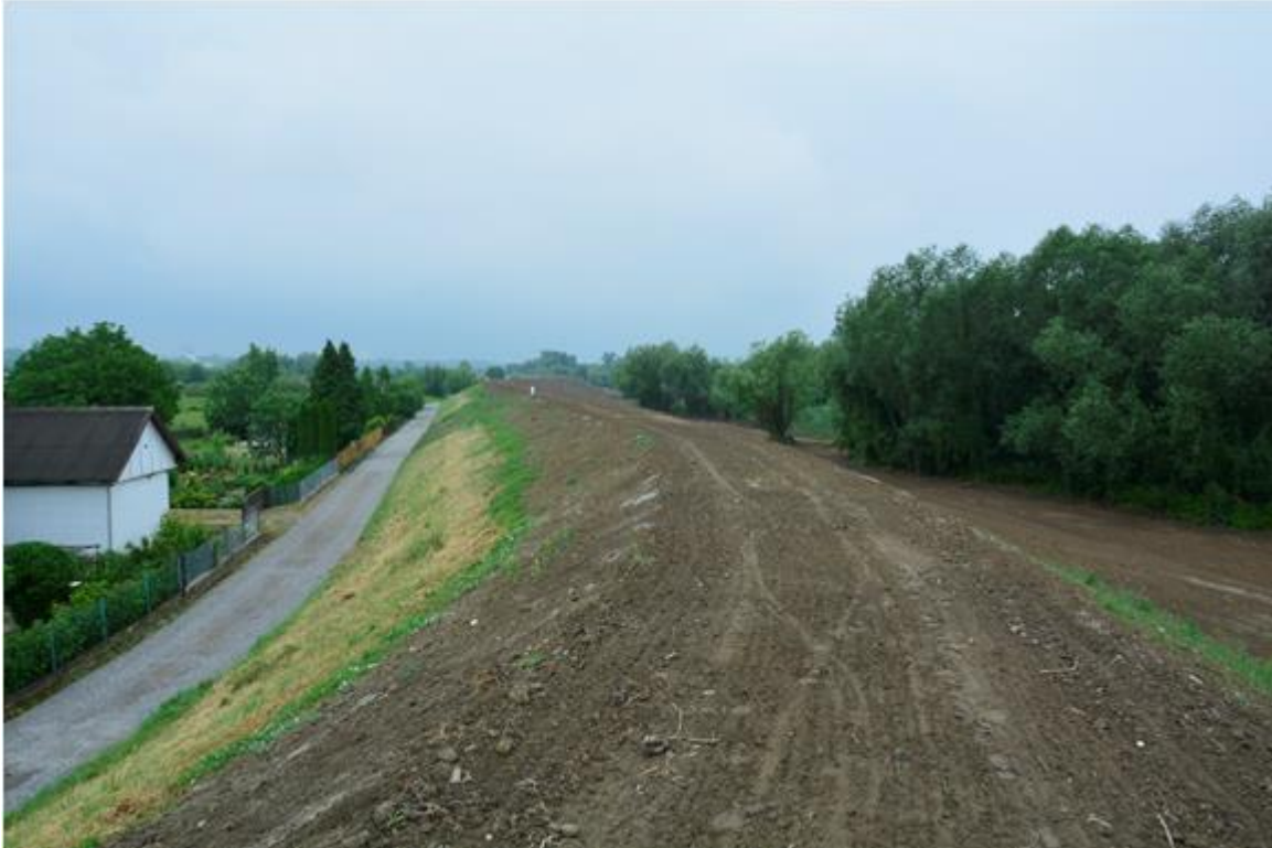
Photo 4. Works completed in the vicinity of the residential area (km 12+800 – 13+400 in line with the building design) (source: the Contractor's Monthly Report).
