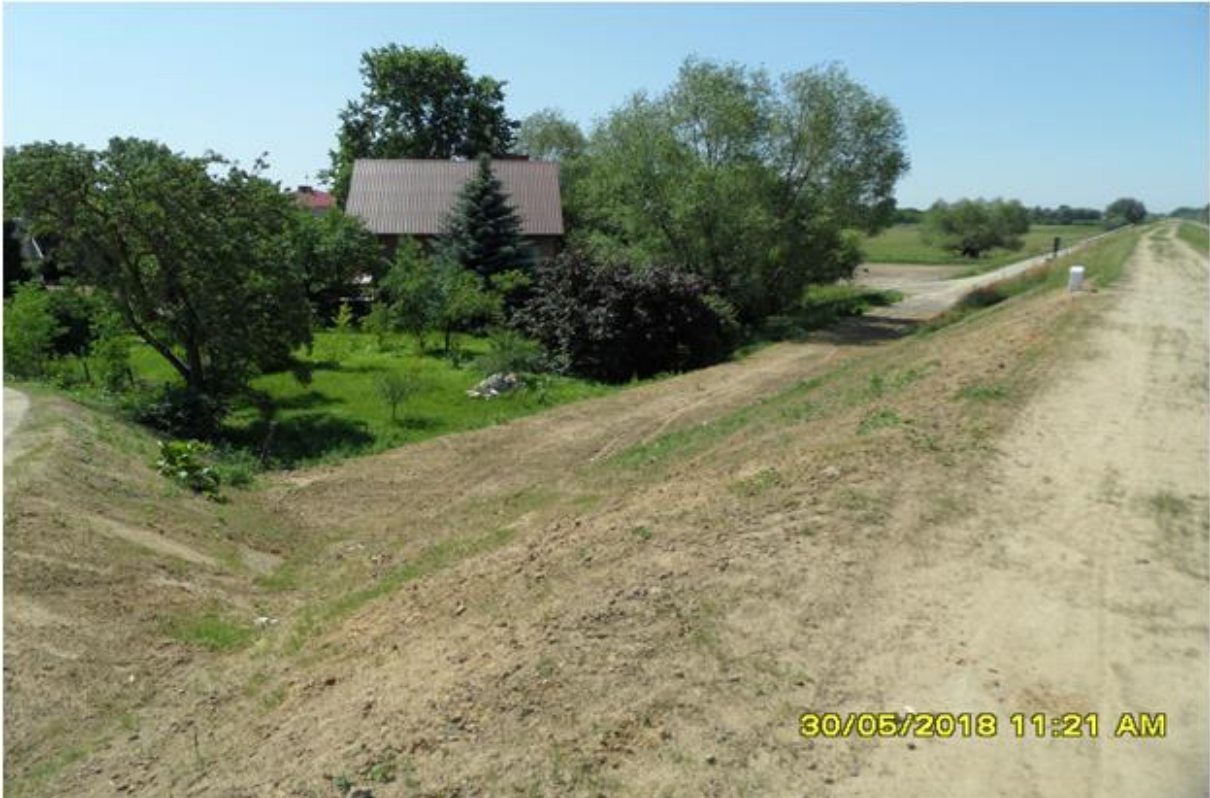
Photo 6. Works completed in the vicinity of the residential area (km 8+200 – 8+300 in line with the building design) (source: own resources of Aecom Polska Sp. z o.o.).
