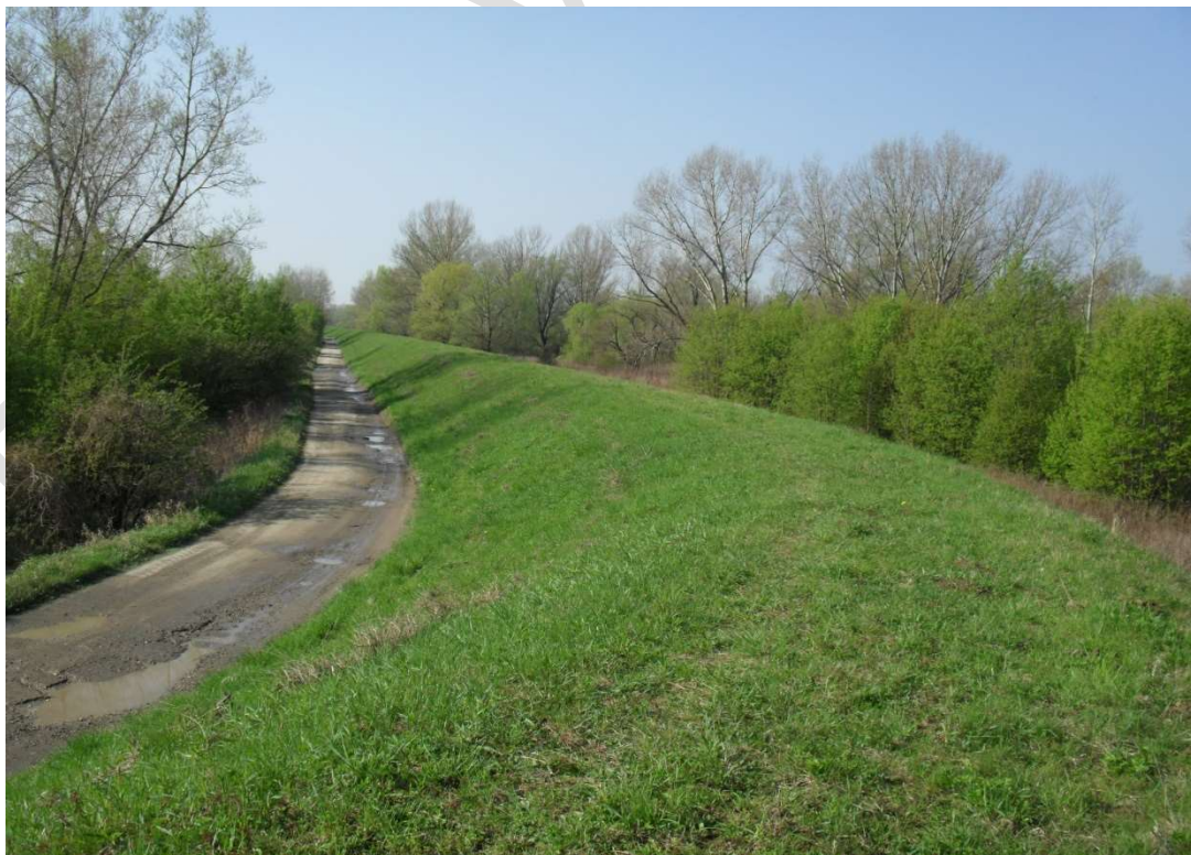
Photo no. 1 Left embankment at chainage km 0+000 – view to the embanked area and a hardened road along the embankment.
