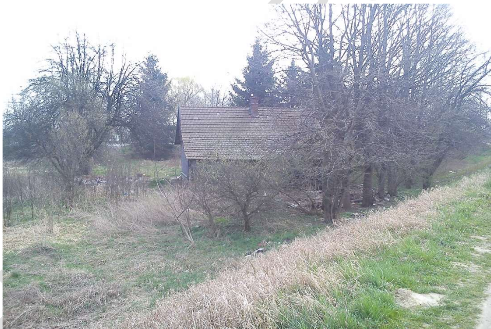
Photo no. 7 Right embankment 5+260 – 5+860 - building approx. 5.0 m from the embankment, trees.
