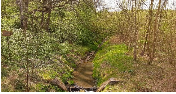
Photo no. 3: Works Contract 3A.2/2, Malinówka 2– investment implementation site – Source: own materials
