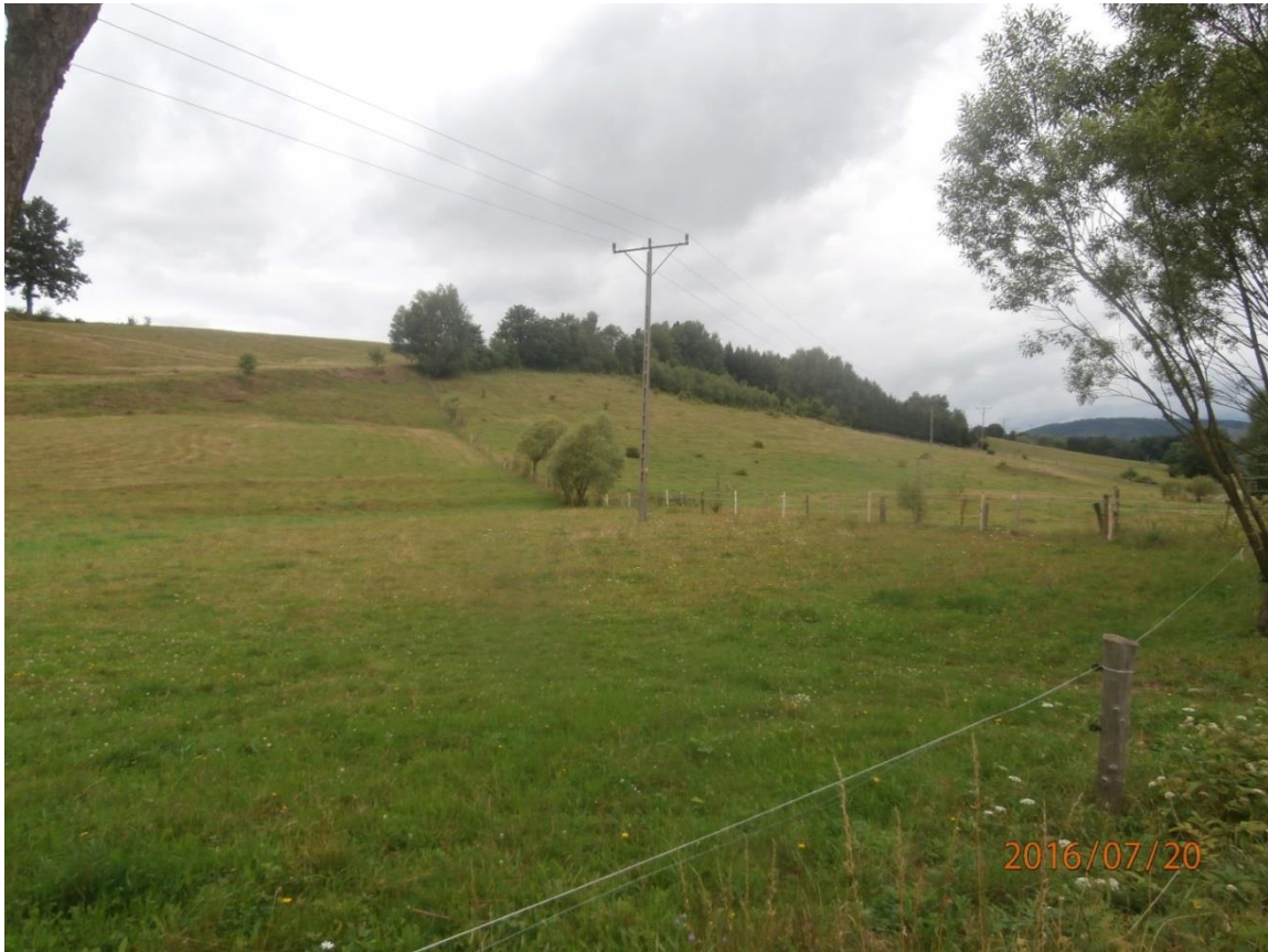
Drawing 4 – The overhead 20 kV MV power line The line is anticipated for refurbishment.
